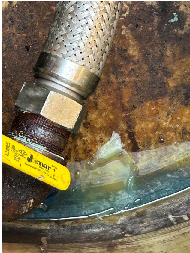
5: Product present in Diesel sump
