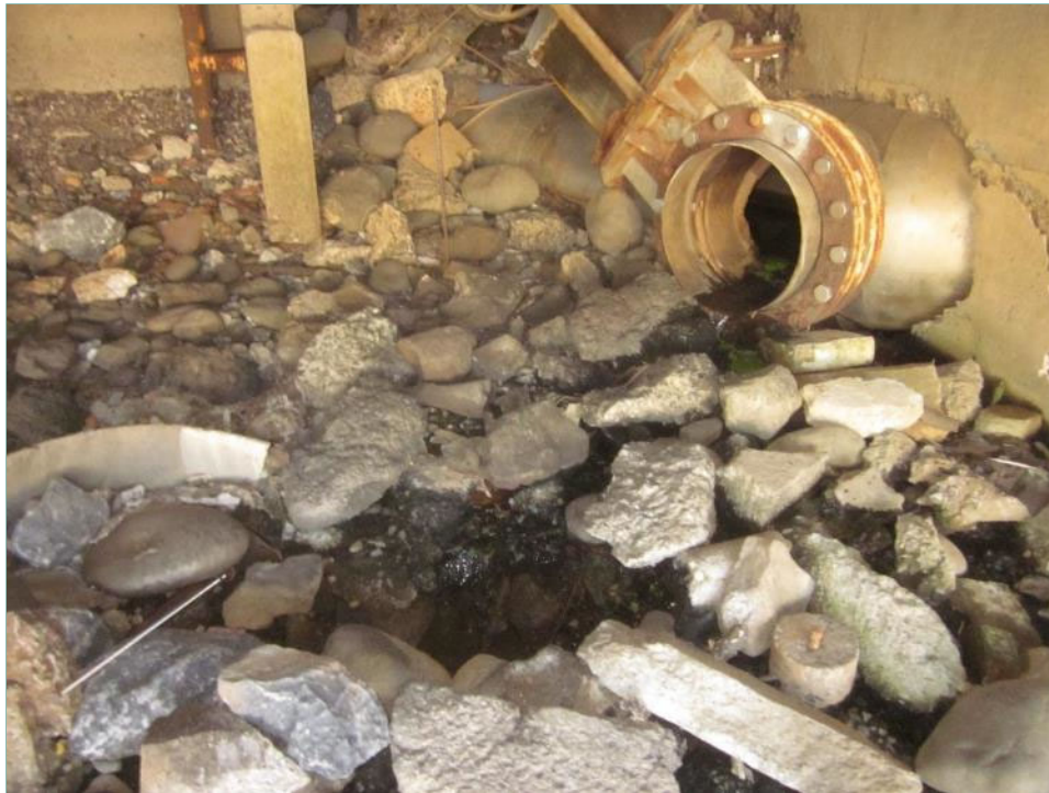
Photo 5: View of knife gate at Tailrace 1 (Outfall 4) discharge area.
