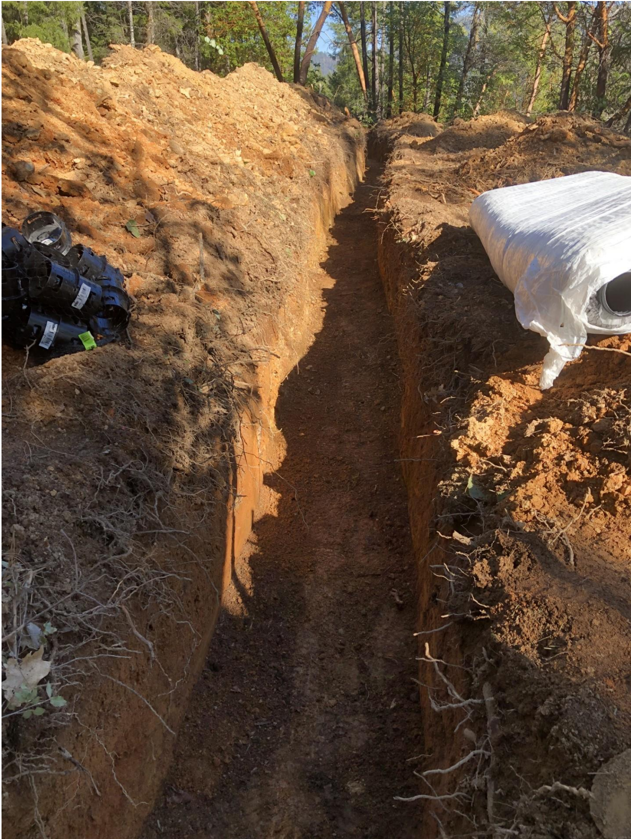
Leach Line #4 – 70 Feet
