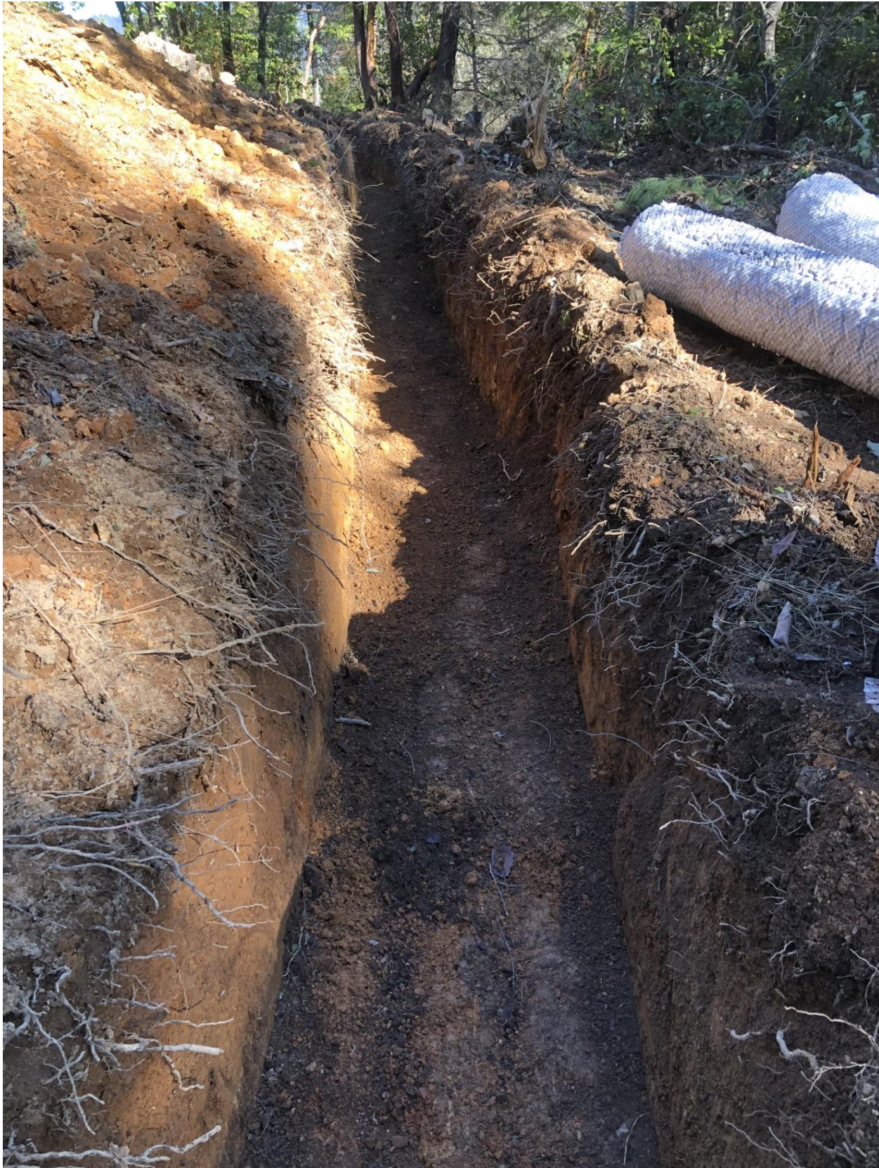
Leach Line #5 – 50 Feet
