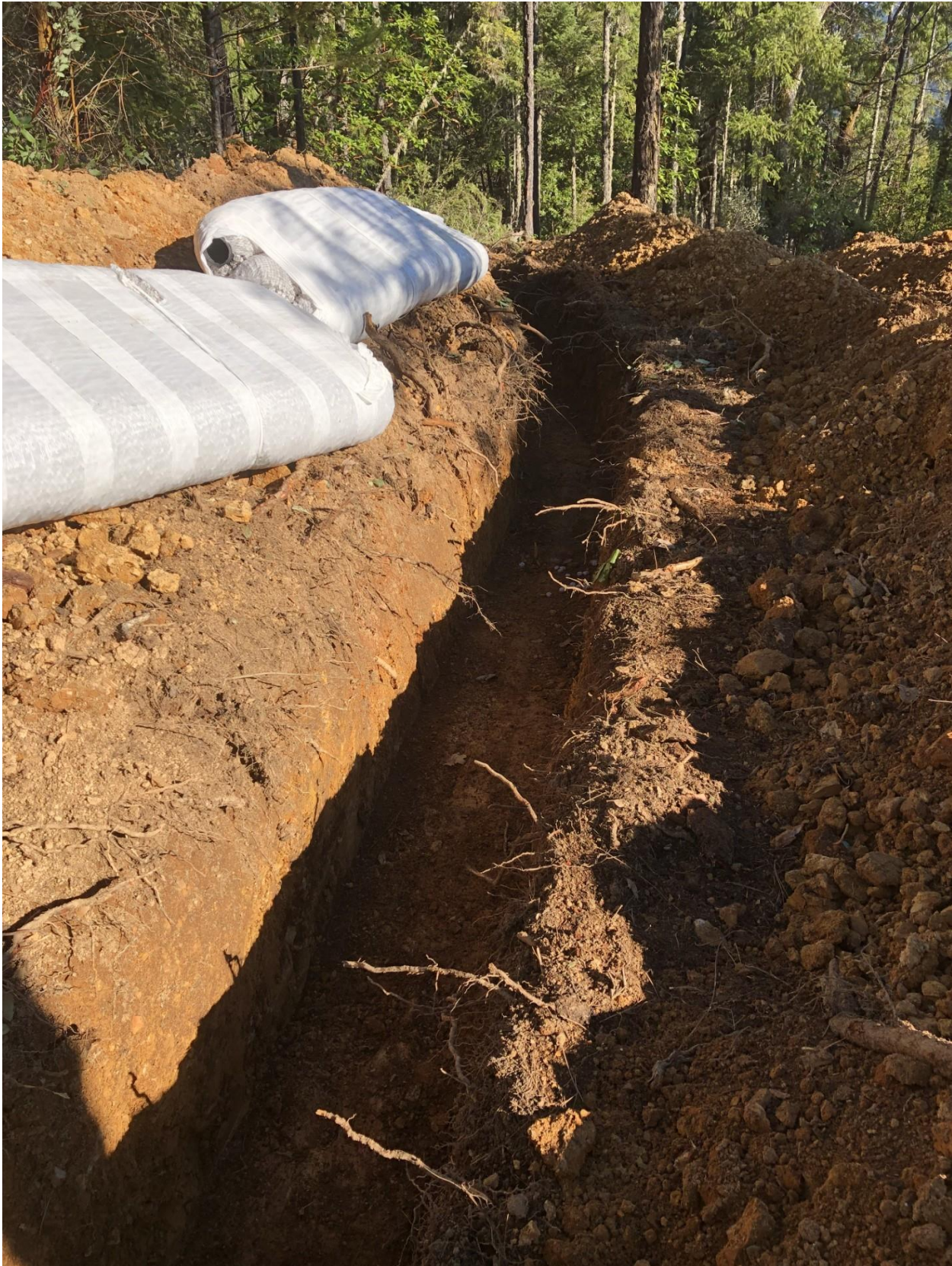
Leach Line #1 - 50 Feet
