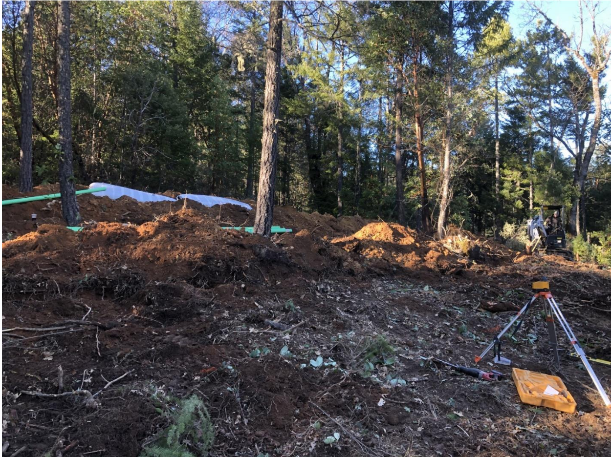
Leach Line #3 – 70 Feet
