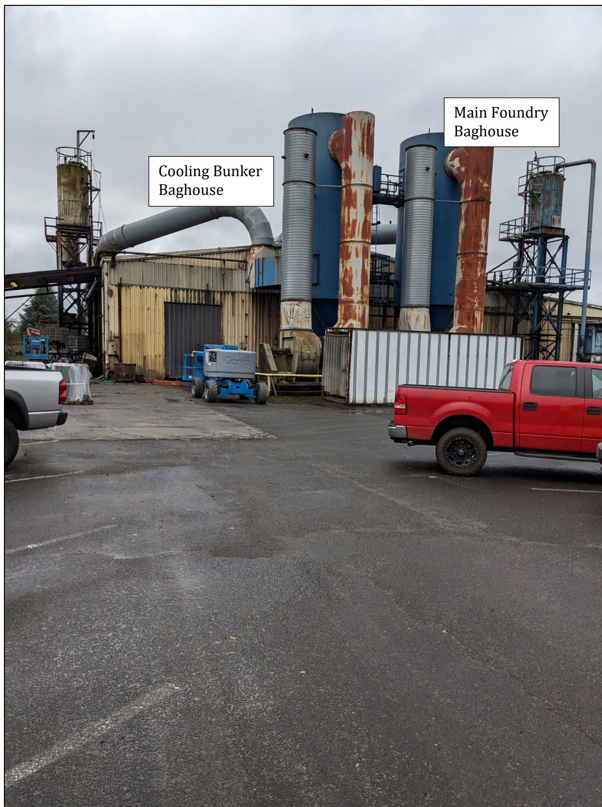
Figure 1 Main Foundry and Cooling Bunker Baghouses
