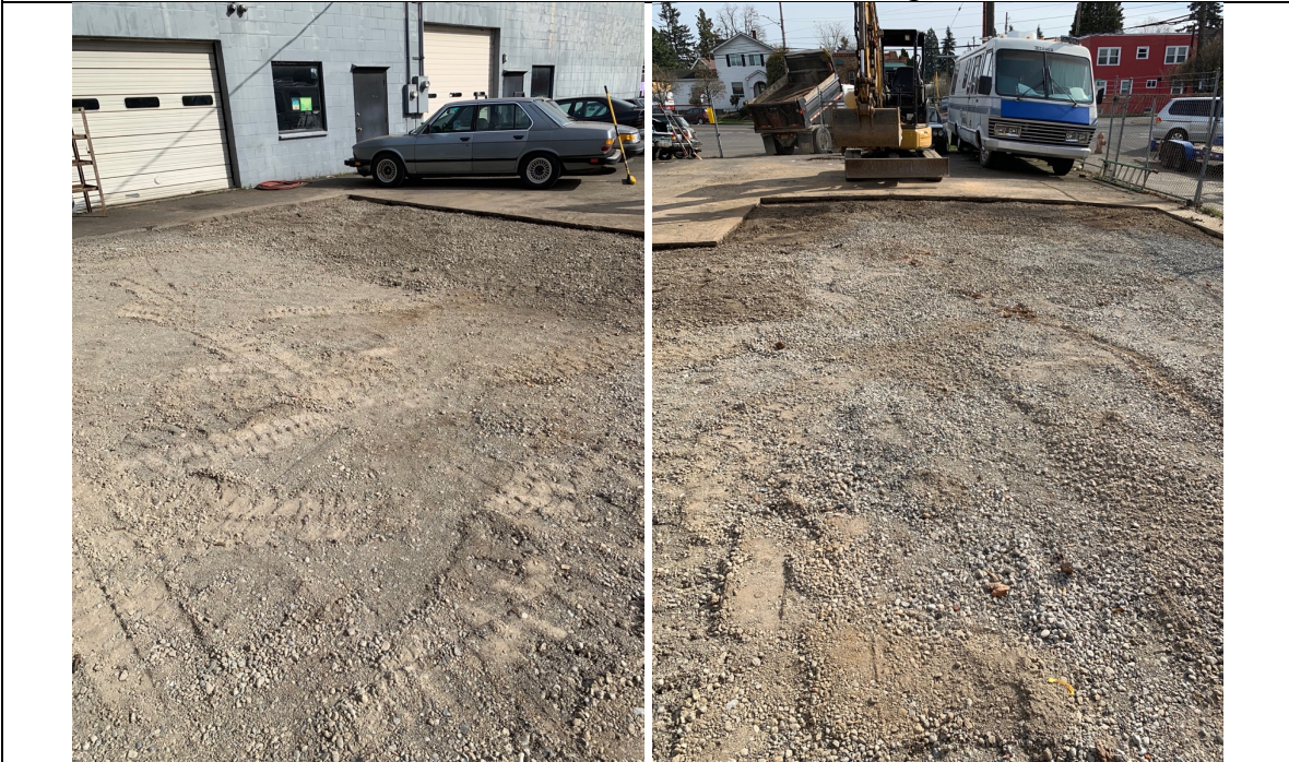
Following receipt of all laboratory analytical results, the tank areas were backfilled with compacted gravel and the surface was repaved with new asphalt.
