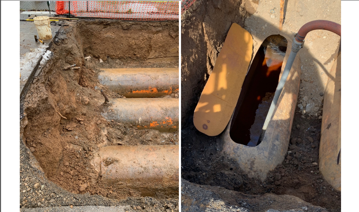
SSES exposed tanks T4, T5, and T6 and inerted them with carbon dioxide. The USTs were then cut open. SSES removed the liquids and the tanks were thoroughly pressure washed.
