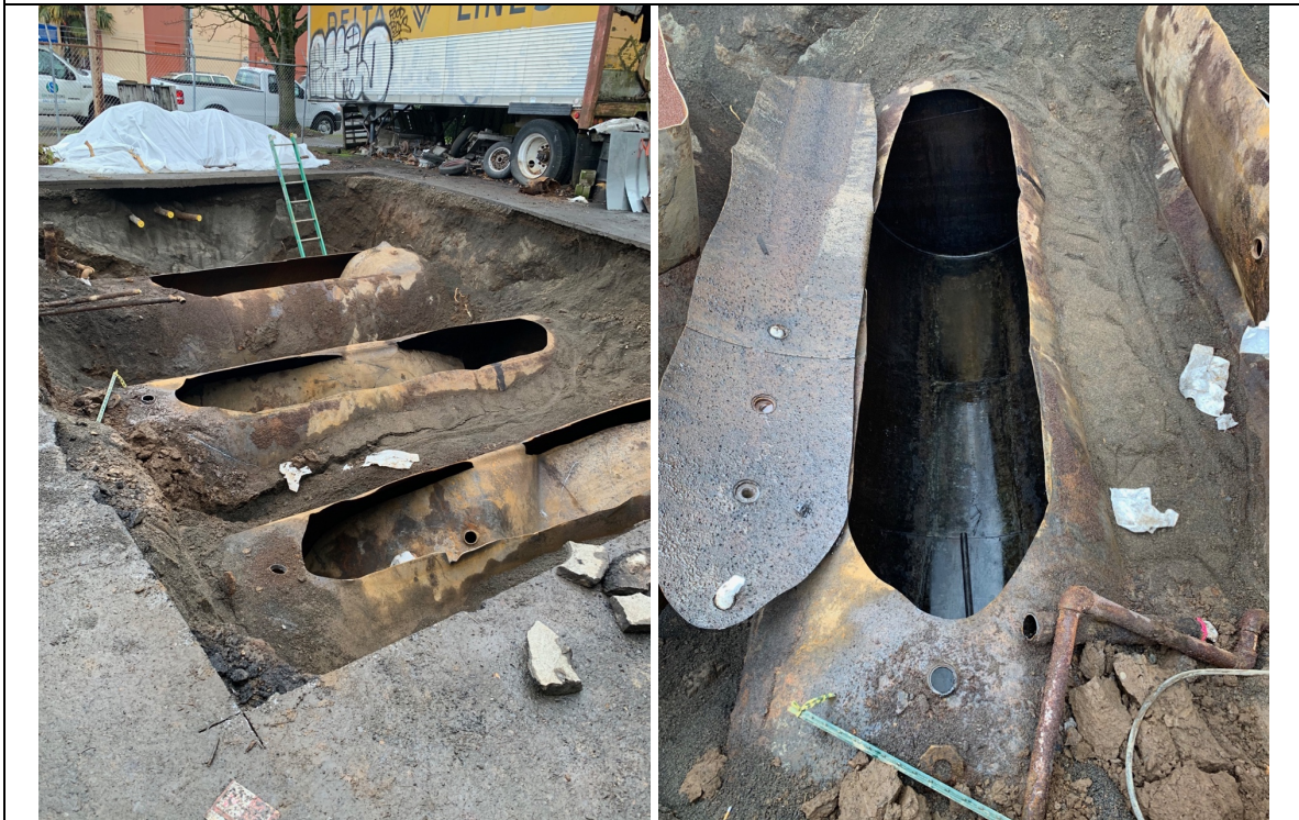
SSES uncovered the tops of T1, T2, and T3 and inerted them with carbon dioxide. The USTs were then cut open. SSES removed the liquids and the tanks were thoroughly pressure washed.
