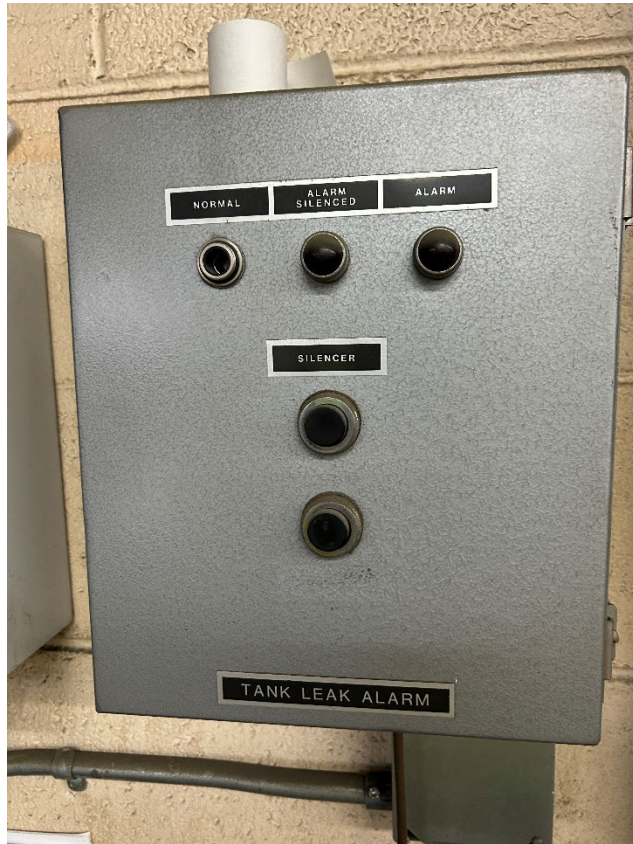
3: Tank leak alarm
