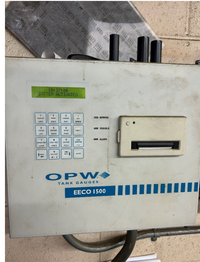
2: OPW Tank gauge
