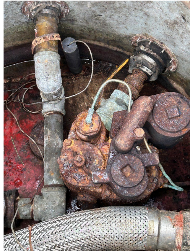
22: Regular sump and turbine
