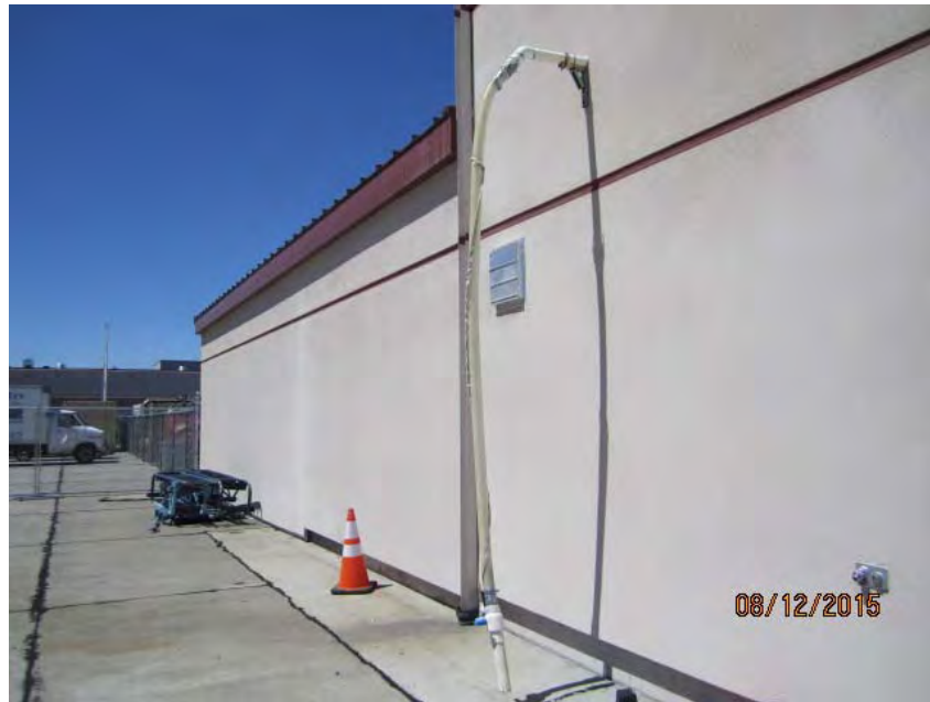
Photo 11: Gravity Pipe for AFFF Supply at Current Fire Station
