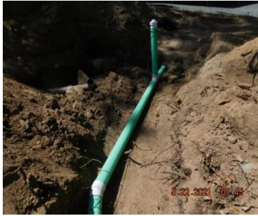
Tank Outlet W/ Cleanout
