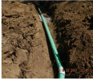
Tank To Drop Box
