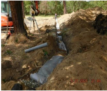
Tile Dewatering Drain, East End
