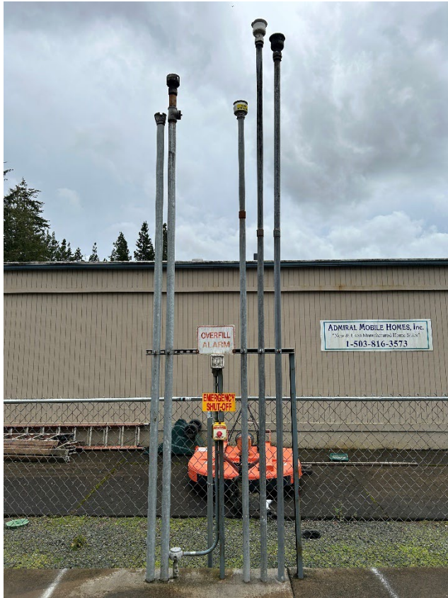
7: Pressure valve vents
