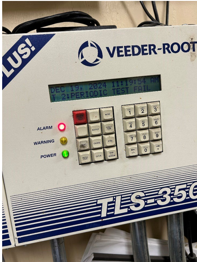
1: Tank 2 alarm at 36453 Hwy 101, Nehalem, OR 97131
