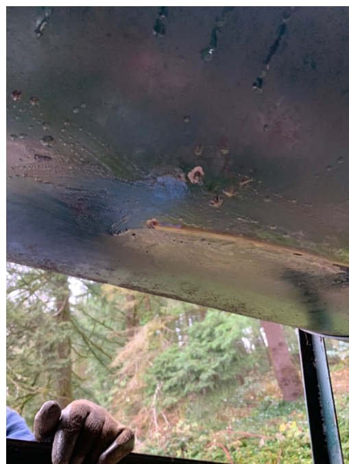
Photo 6. A pinhole and pitting were observed on the tank bottom. View is from under the tank.
