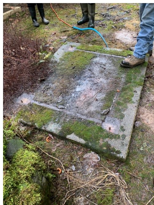
Photo 8. Contaminated concrete was observed below the former AST location. View of concrete pad.
