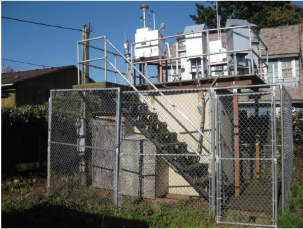
Figure 5: The Air Toxics Monitoring Station in North Portland.
