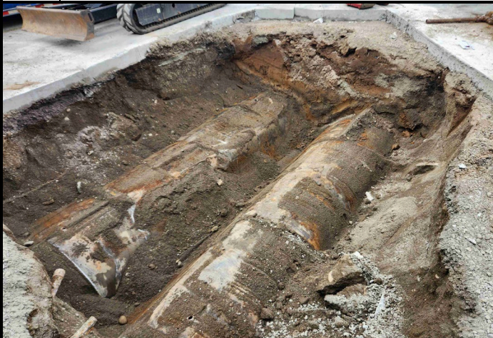
Photo #3: Exposed USTs
