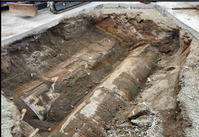
Photo #3: Exposed USTs
