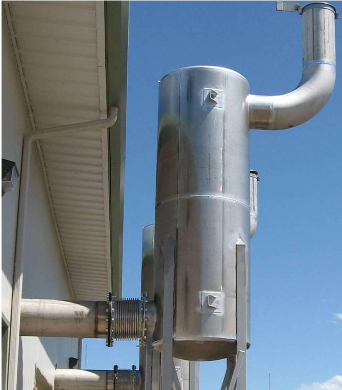
CAT engine exhaust stacks used to generate electricity
