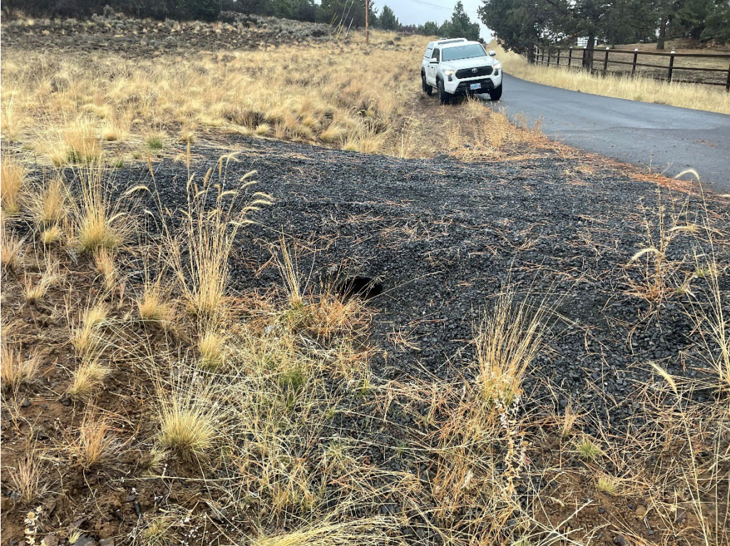
Parcel AR – Minor gravel blockage but culvert has generally unrestricted capacity.
