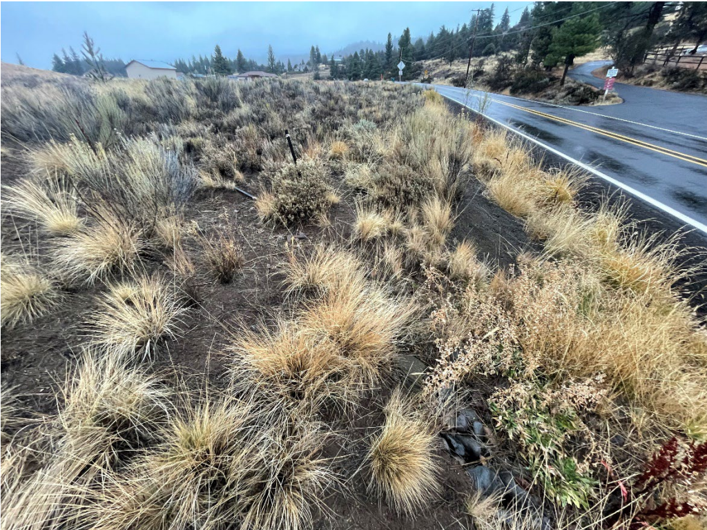
Parcel AP – No repairs made to gully near southeast corner of parcel.
