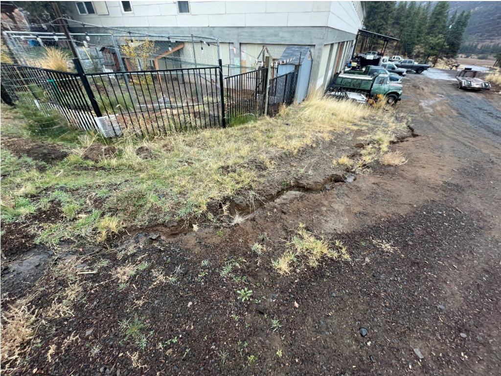
Parcel MBK-G – No repairs made to gully near southeast corner of warehouse.
