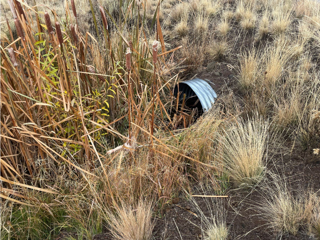
Parcel AP – Some vegetation blockage but culvert has generally unrestricted capacity.
