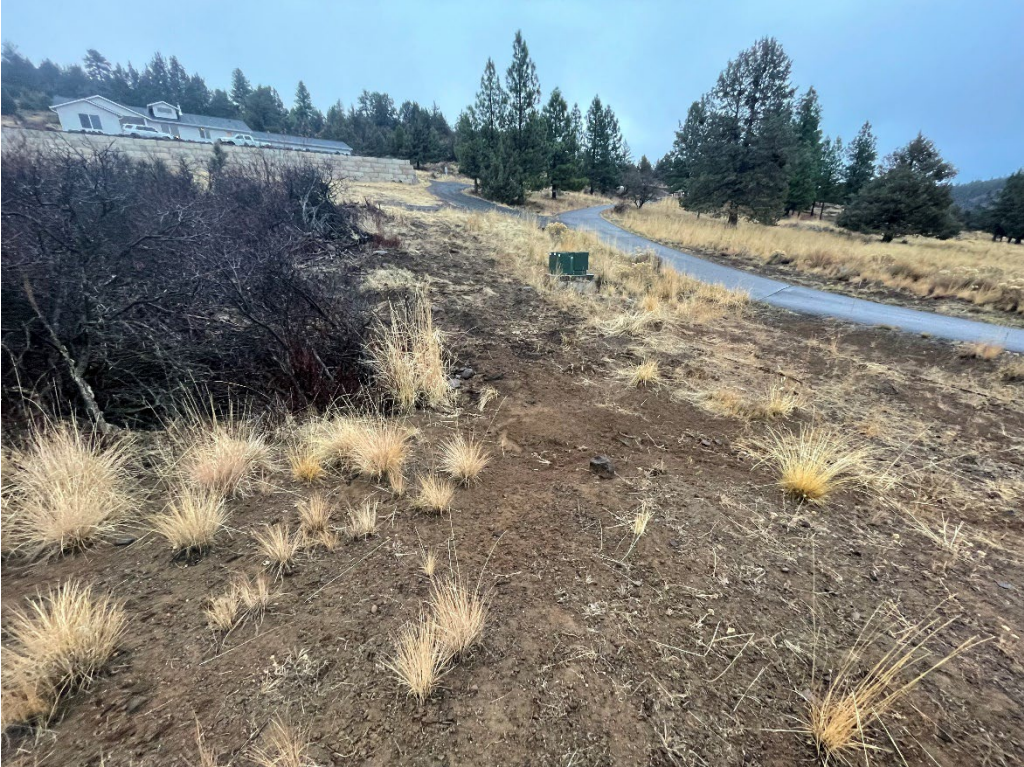
Parcel H – Gully near north edge of Lot H2 backfilled with soil and graded on slope.
