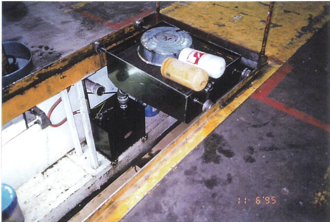
Photograph 2: Remote fill from maintenance pit to waste oil UST (Facing north)
