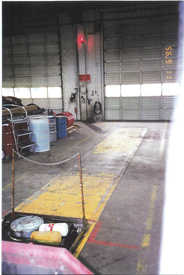
Photograph 3: View of length of underground piping run from the remote fill location to the waste oil UST (facing northeast)
