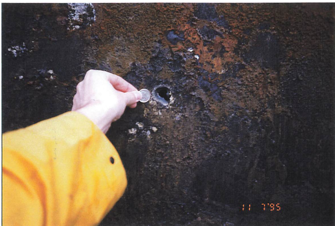
Photograph 5: View of corrosion hole found on west side of the southeast end wall of the UST
