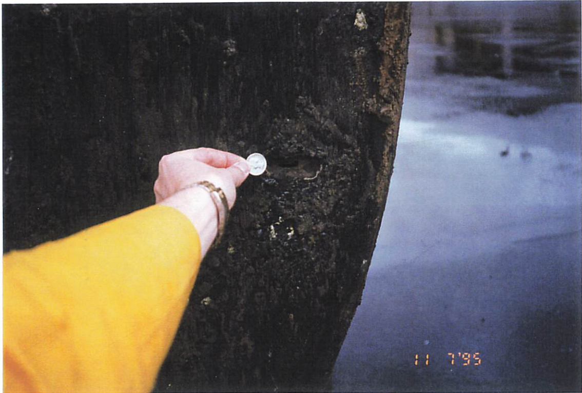
Photograph 6: View of corrosion hole found on east side of the southeast end wall of the UST
