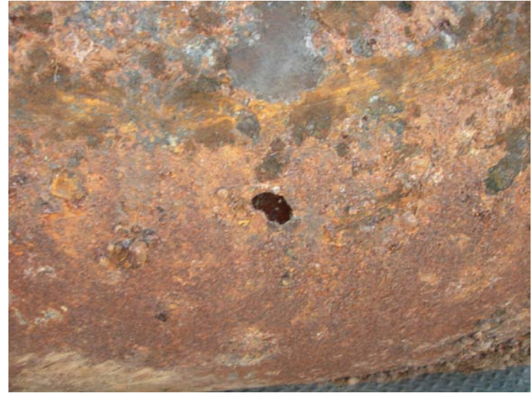
Corrosion holes visible in the side of the tank.
