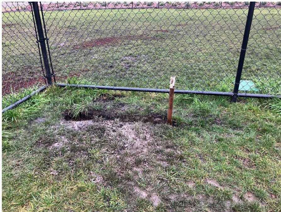
PHOTO I.D. 10: SUBSURFACE IRRIGATION LINE REPAIR WITHIN THE SMALL DOG PARK IN DISPOSAL CELL #2. PHOTOGRAPH TAKEN FACING EAST.
