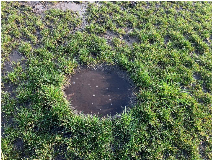
PHOTO I.D. 4: HOLE IN SOIL CAP WITHIN THE LARGE DOG PARK IN DISPOSAL CELL #2.
