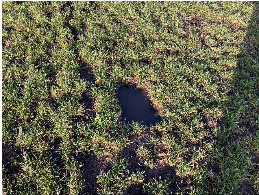
PHOTO I.D. 3: HOLE IN SOIL CAP WITHIN THE LARGE DOG PARK IN DISPOSAL CELL #2.
