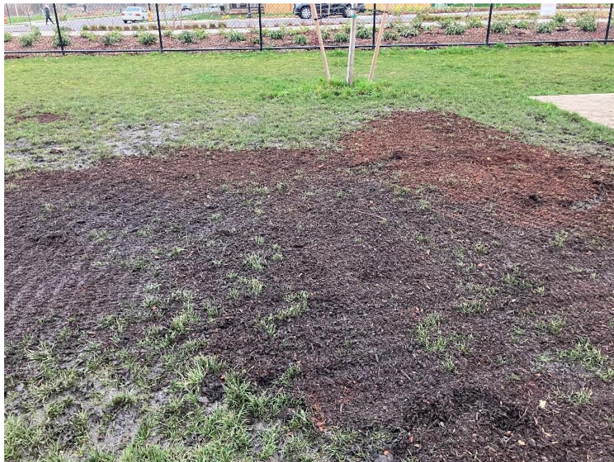
PHOTO I.D. 12: AREA OF SOIL CAP REPAIR WITHIN THE LARGE DOG PARK IN DISPOSAL CELL #2 WHERE A LOW SPOT WITH PONDED WATER HAD BEEN OBSERVED. PHOTOGRAPH TAKEN FACING EAST.
