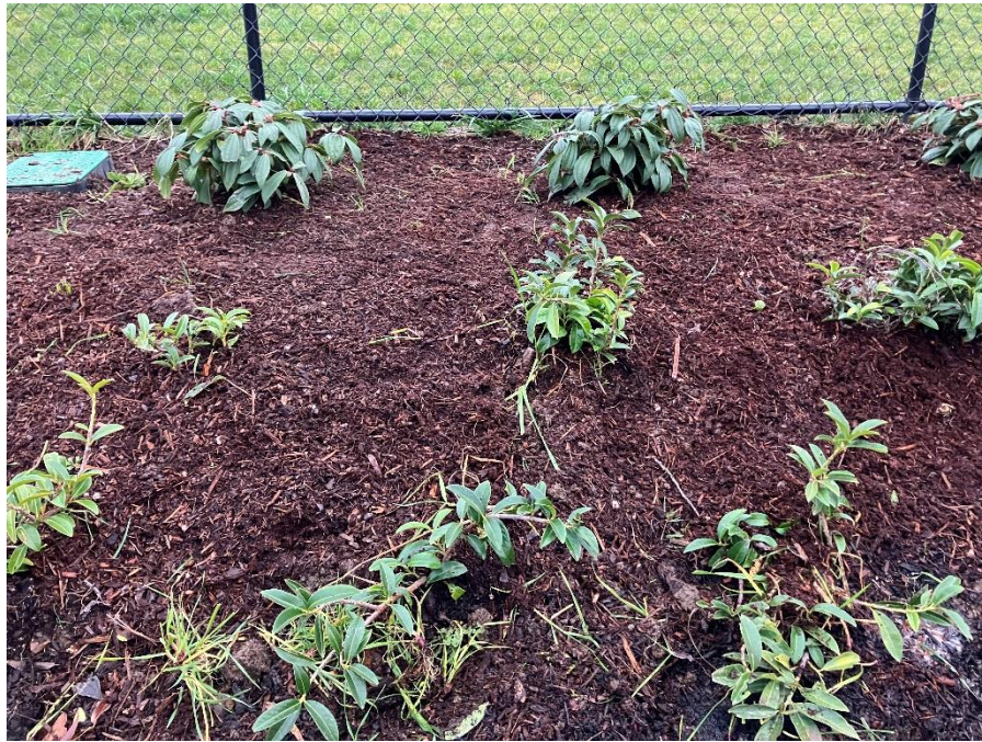
PHOTO I.D. 11: AREA OF SOIL CAP REPAIR IN LANDSCAPING ALONG THE NORTHWEST PORTION OF DISPOSAL CELL #2 WHERE EROSION HAD BEEN OBSERVED. PHOTOGRAPH TAKEN FACING SOUTHWEST.
