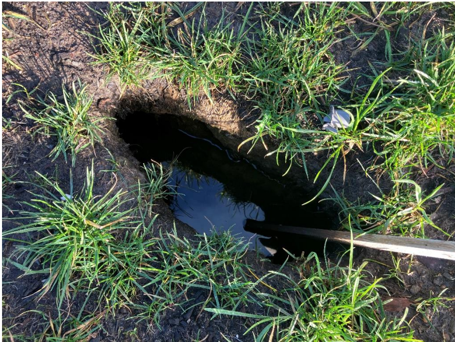
PHOTO I.D. 2: HOLE IN SOIL CAP FROM BROKEN IRRIGATION LINE WITHIN THE SMALL DOG PARK IN DISPOSAL CELL #2.
