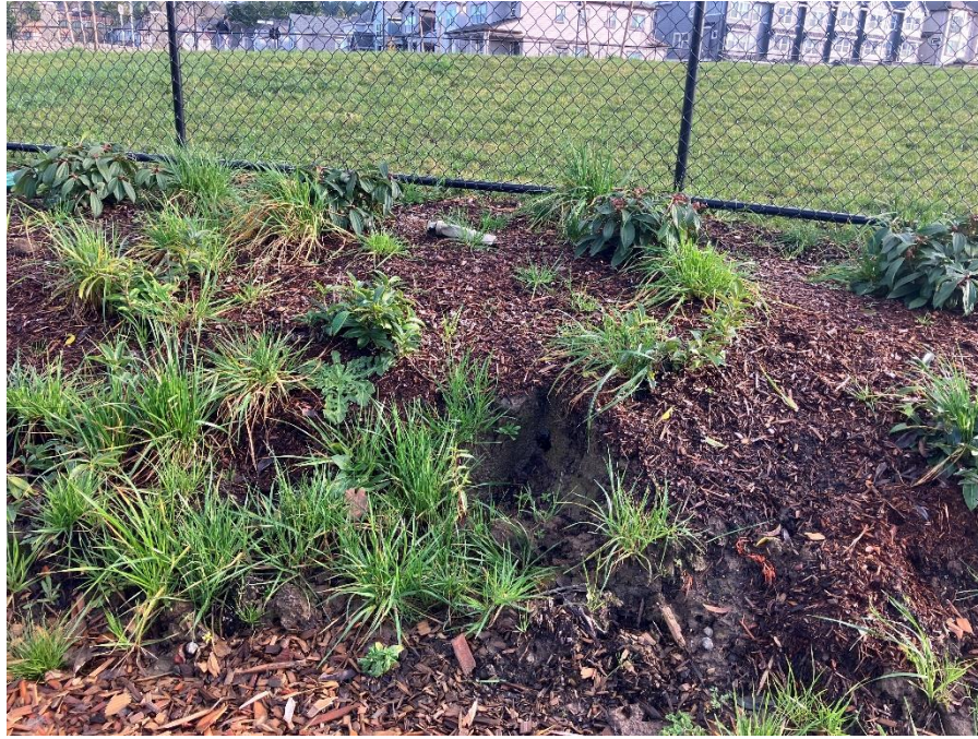
PHOTO I.D. 5: EROSION IN LANDSCAPING ALONG THE NORTHWEST SLOPE OF DISPOSAL CELL #2. PHOTOGRAPH TAKEN FACING SOUTHWEST.
