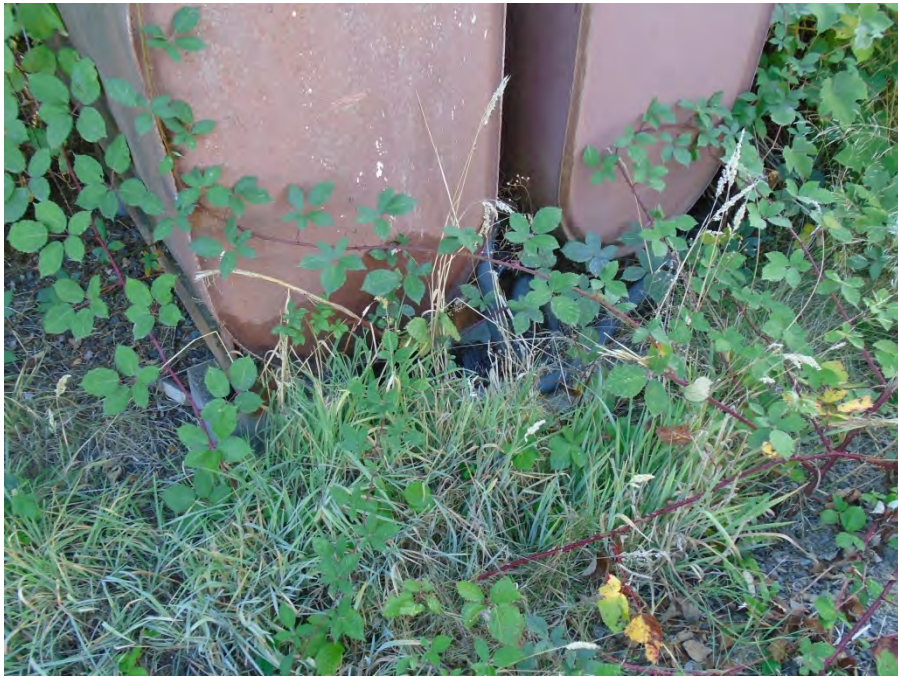
LEAKING HEATING OIL AST LOCATED ADJACENT TO THE RESIDENCE LOCATED AT 15685 SW 150 TH AVENUE. PHOTOGRAPH TAKEN FACING EAST.
