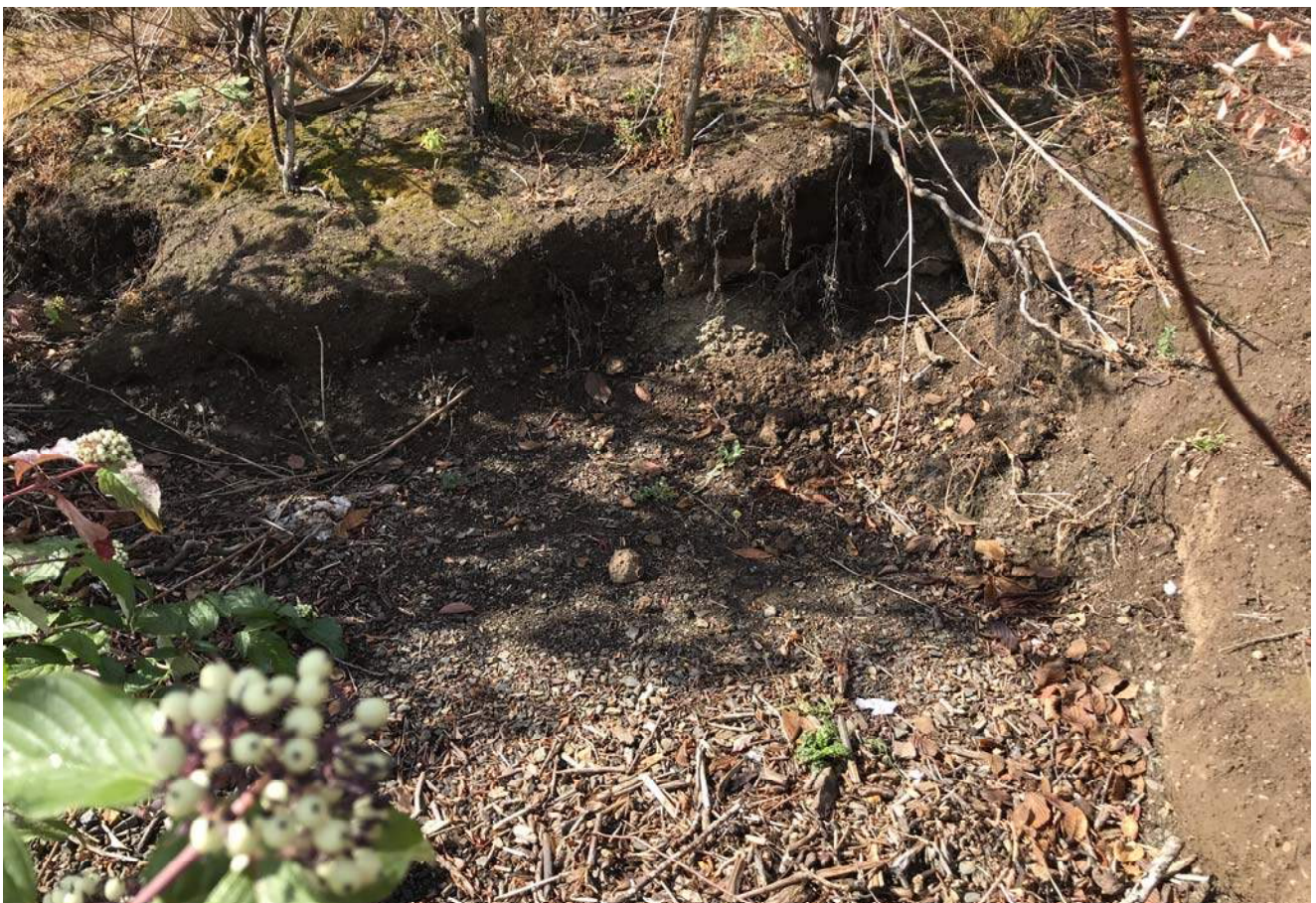
STA: 25+00 - Lower bank erosion
