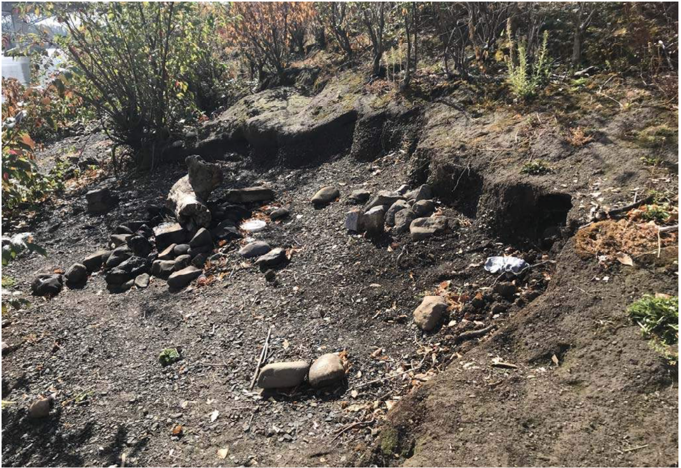
STA: 25+50 - Lower bank erosion and fire pit
