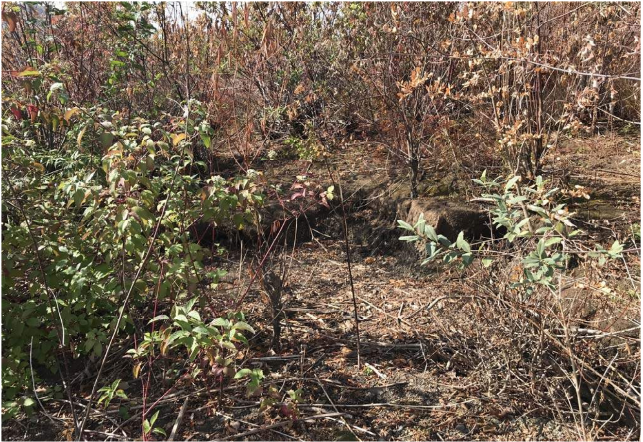
STA: 24+00 - Lower bank erosion to approximate elevation 17'
