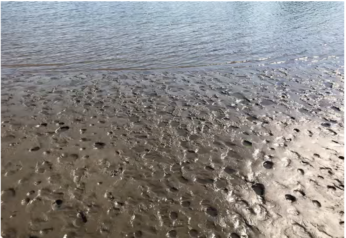
Sediment buildup in the slipway ramp looking east.
