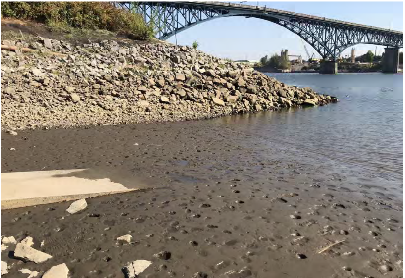
Sediment buildup in the slipway ramp looking northeast.
