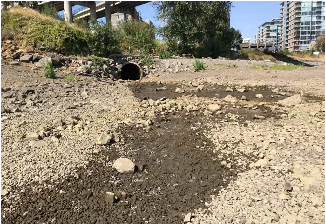
City outfall 07B.
