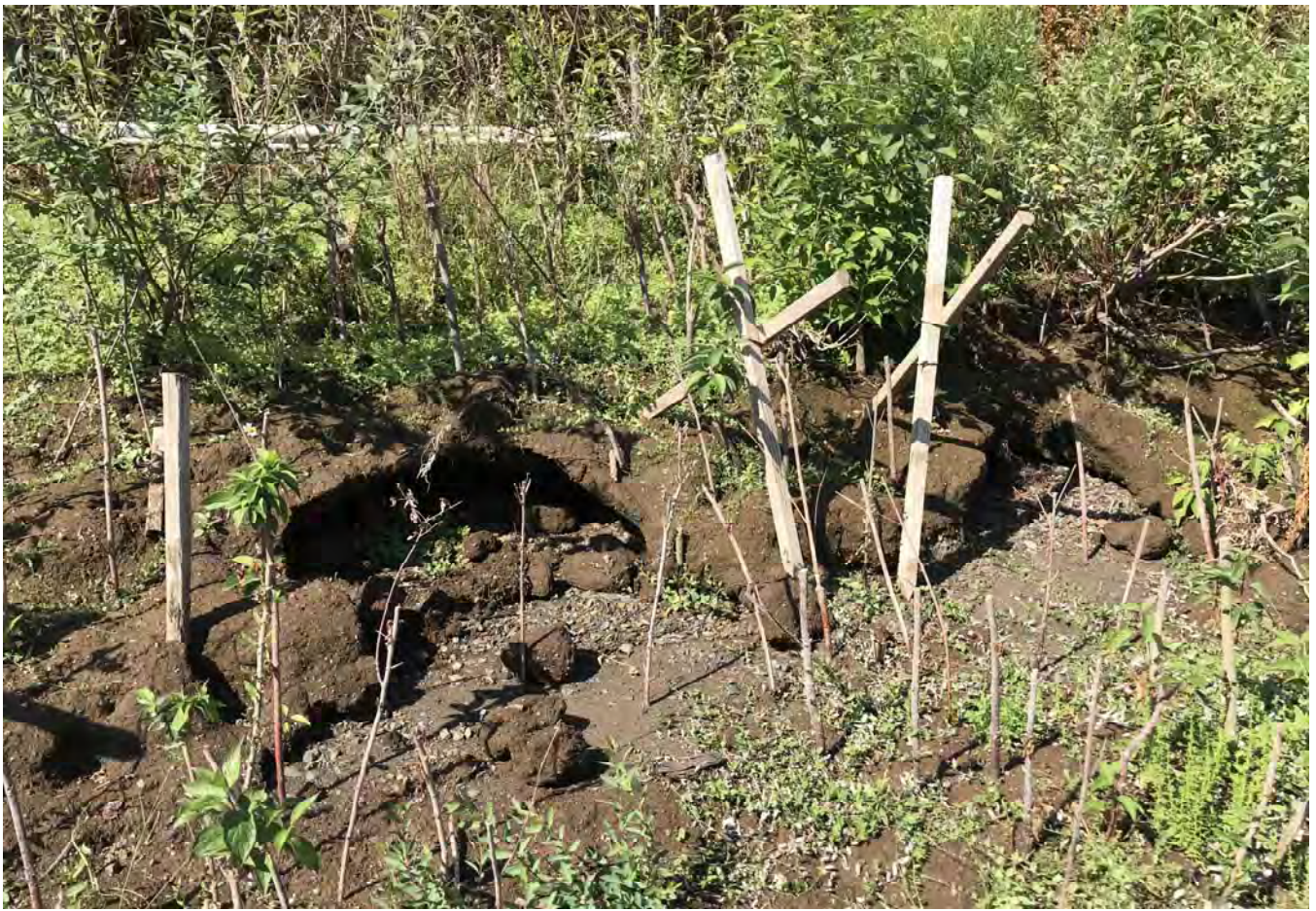
STA: 18+50 - Undercut erosion on lower bank.
