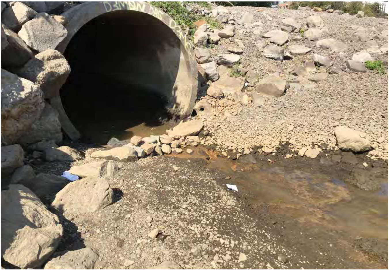
Water flowing from City outfall 07B.
