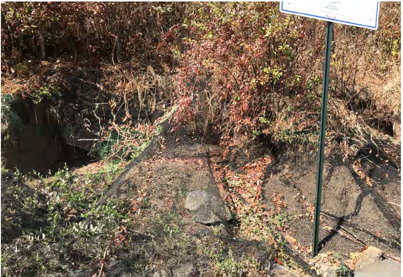
STA: 6+25 - Bank erosion above top of rock armor.
