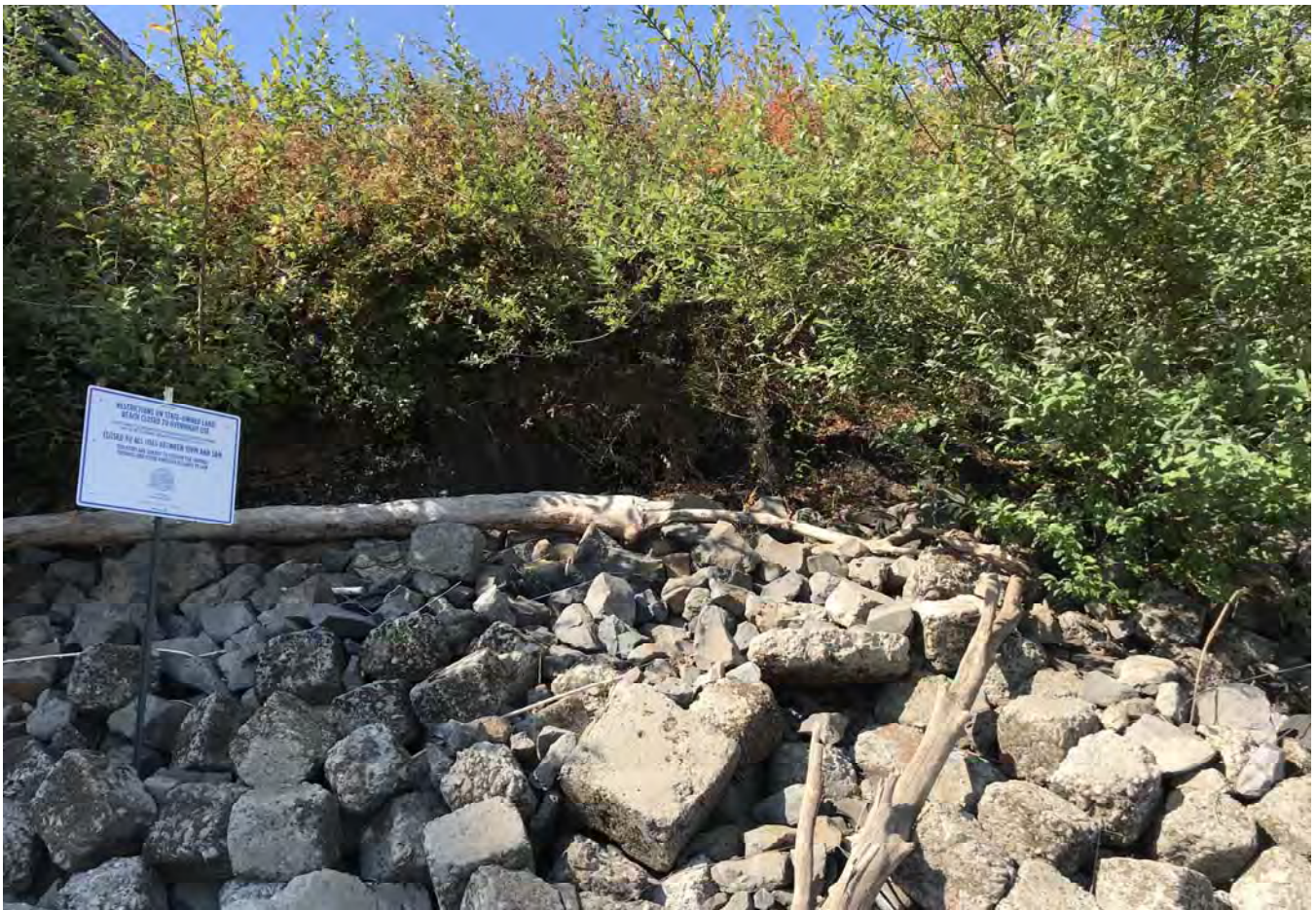
STA: 7+50 - Bank erosion over top of rock armor.
