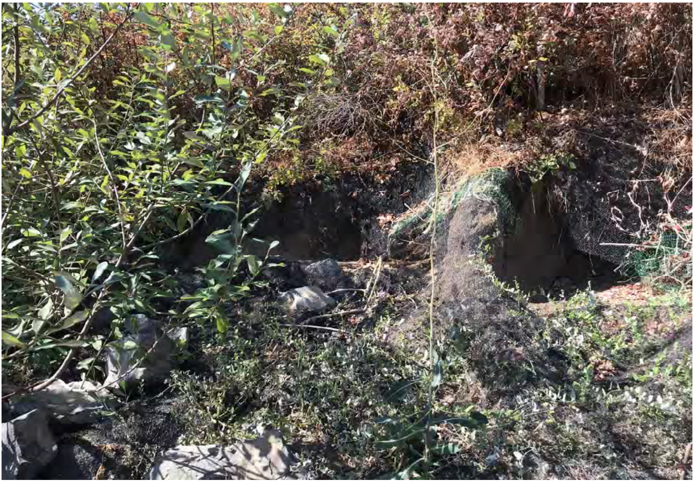
STA: 6+00 - Bank erosion above edge of rock armor.
