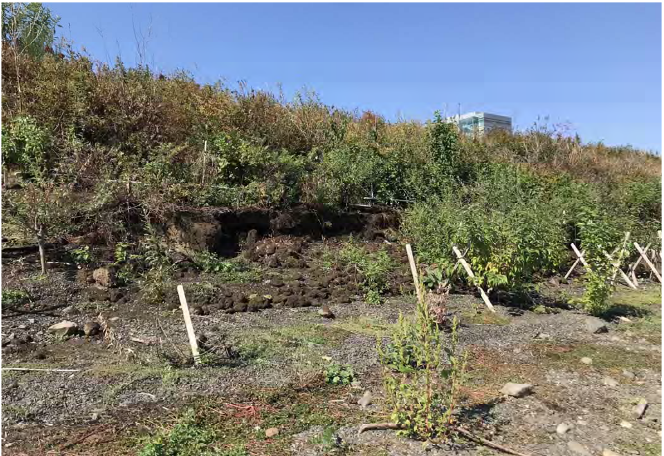
STA: 12+75 - Bank erosion on lower bank looking northwest.
