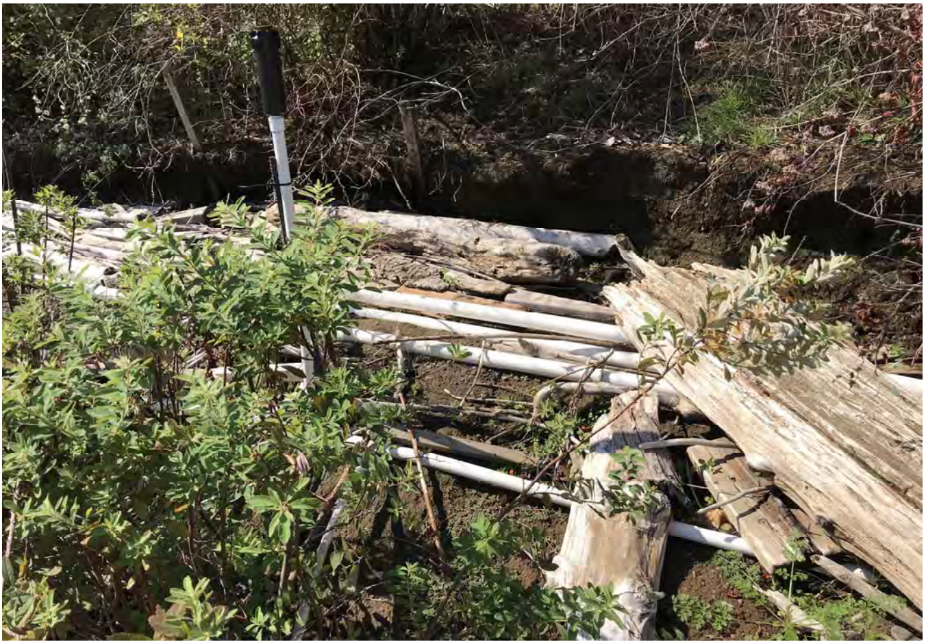
STA: 20+50 - Erosion on lower bank around irrigation lines.
