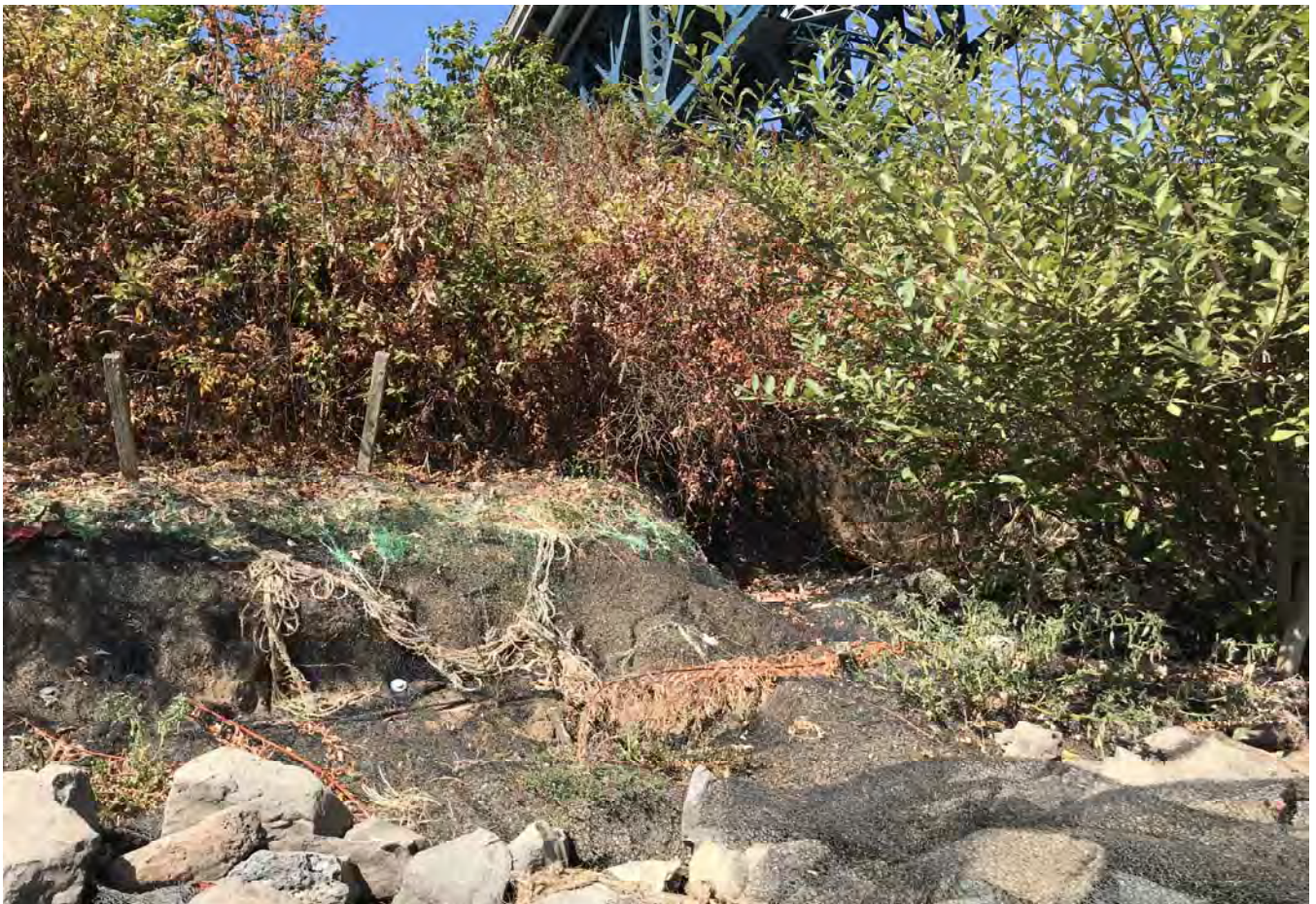
STA: 6+00 - Bank erosion above rock armor.
