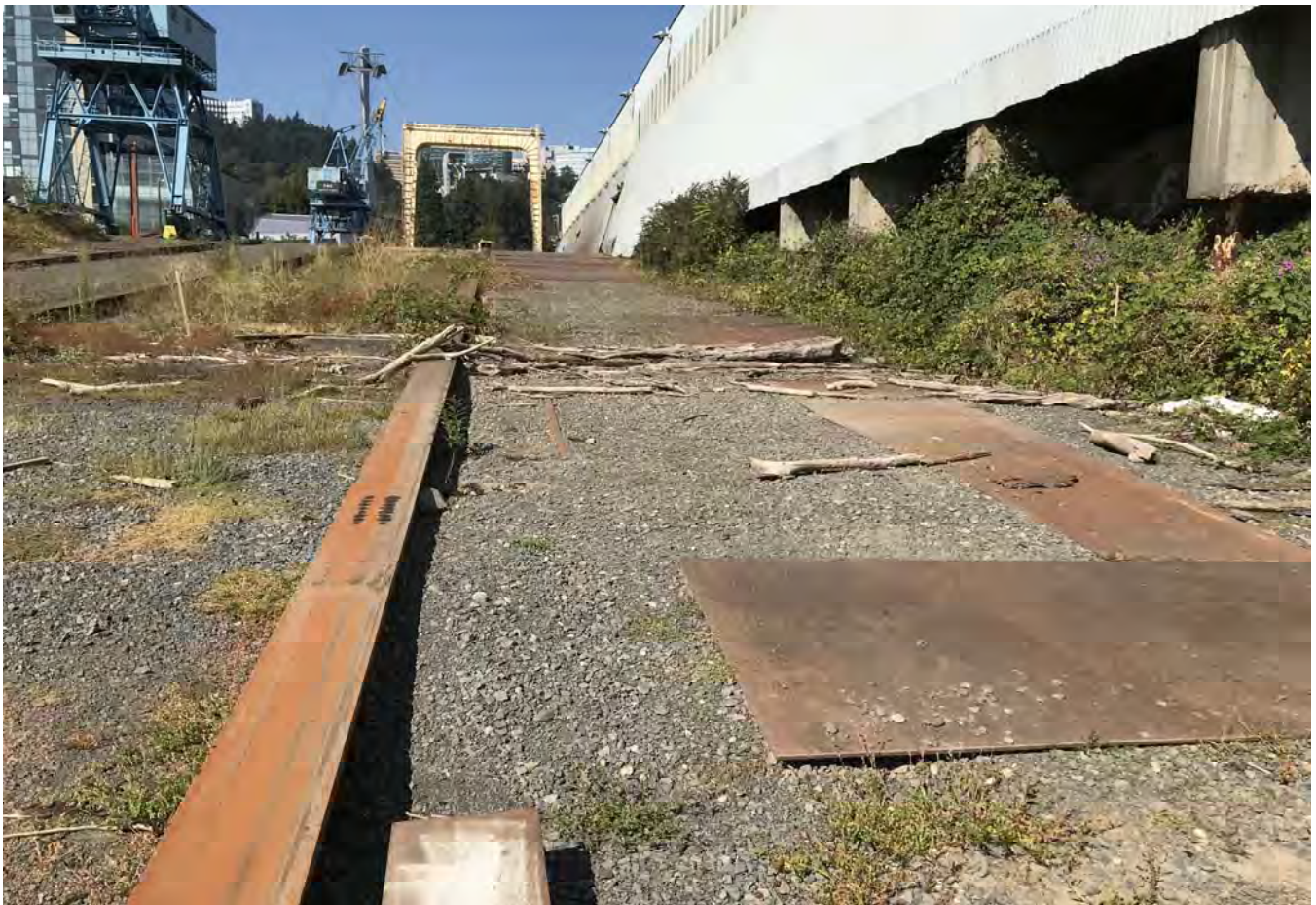
Debris and gravel in slipway ramp looking west.
