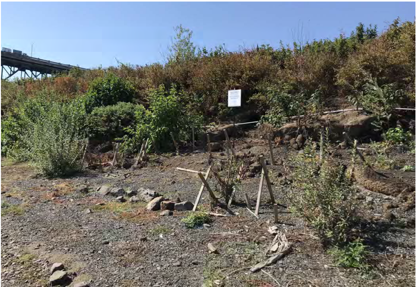
STA: 12+50 - Bank erosion and access restriction sign looking southwest.
