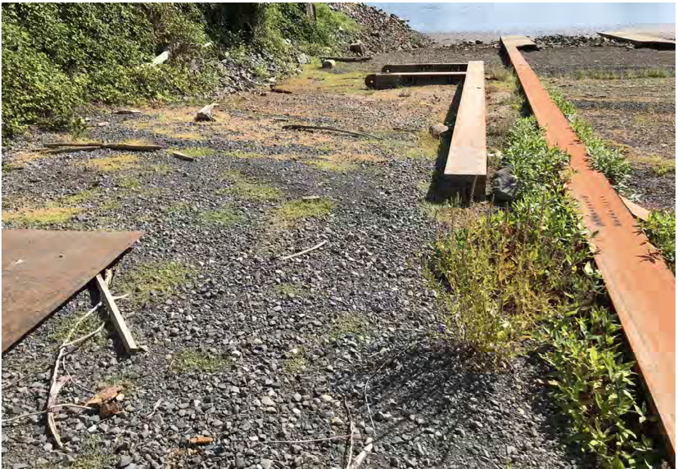
Vegetation, woody debris, and gravel in slipway ramp looking east.
