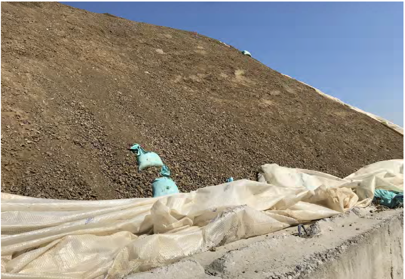
Geotextile cover not secured on gravel stockpiles on site.
