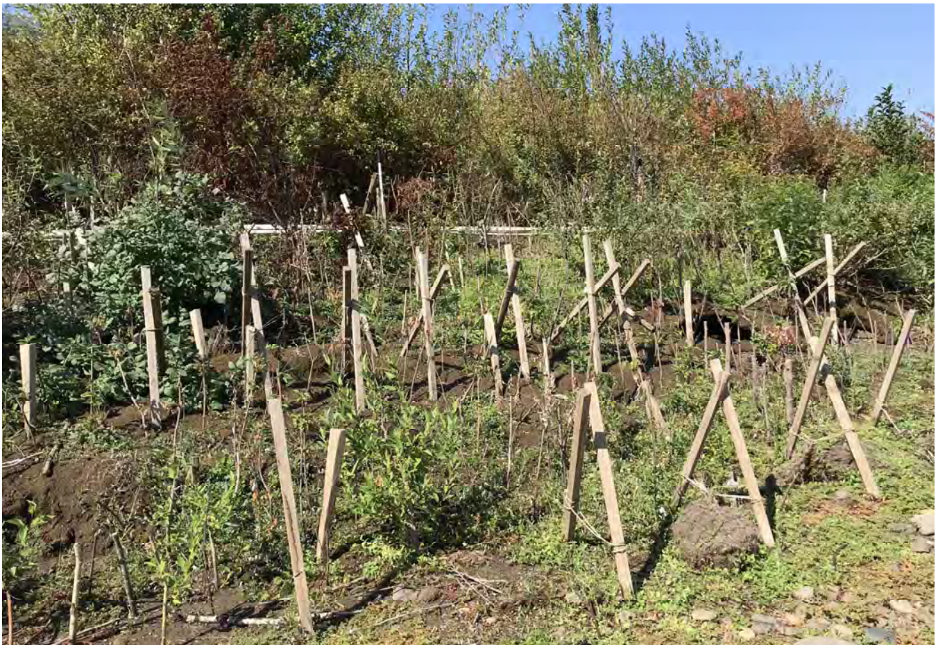
STA: 18+50 - Erosion and vegetation loss on lower bank.
