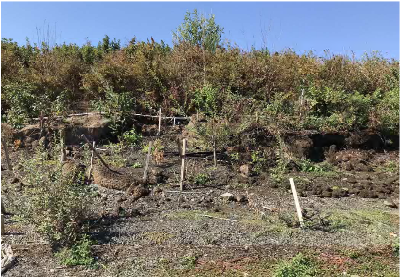
STA: 12+50-75 - Bank erosion on lower bank looking west.
