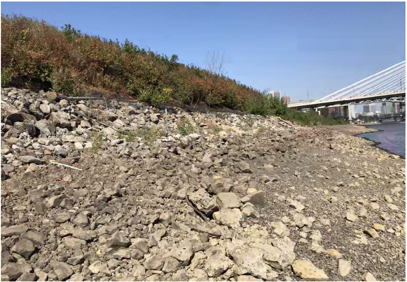
STA: 9+00 - Bank repair area ballast stones migrating over sediment cap area.
