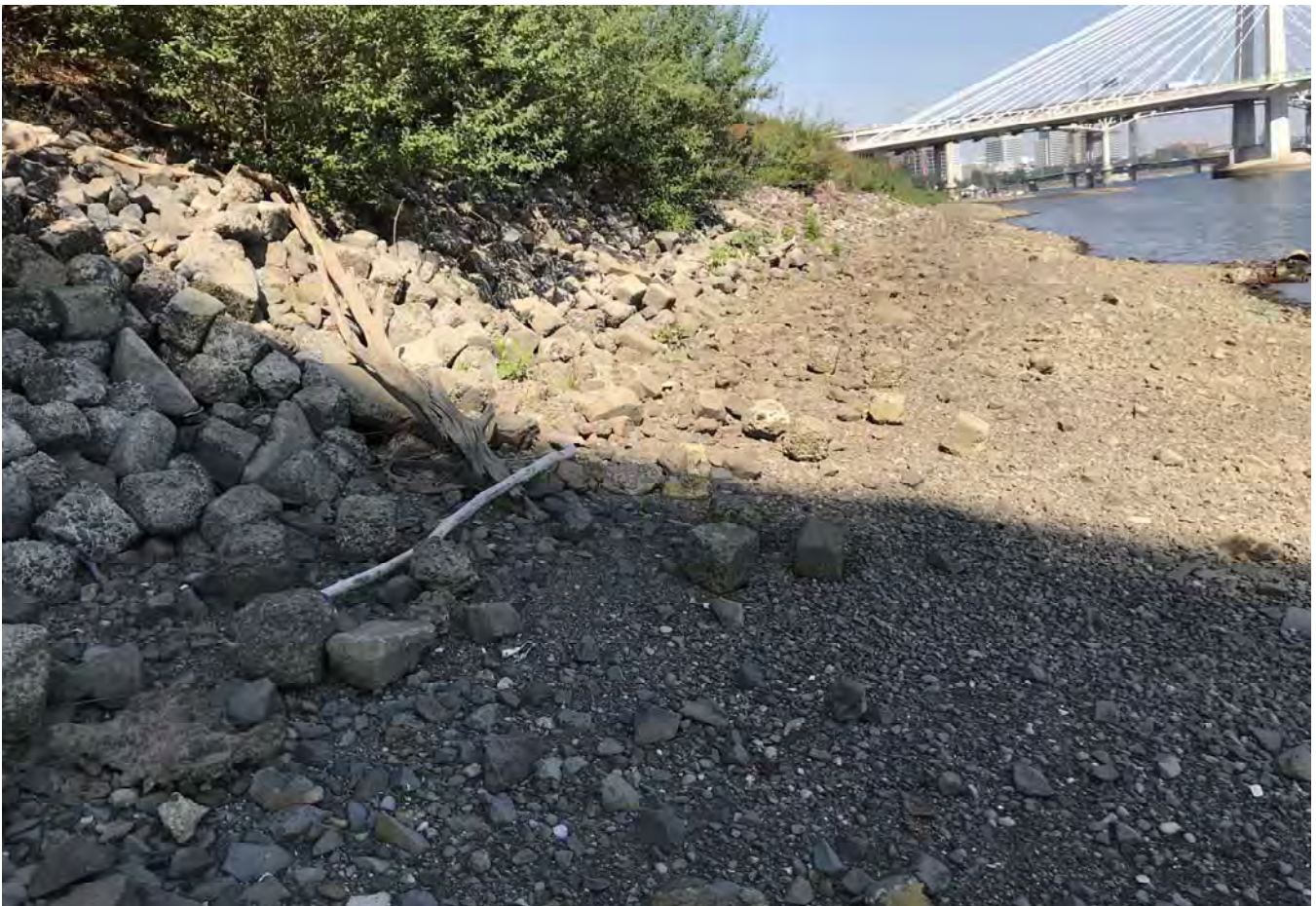
STA: 7+25 - Ballast stones from bank repair area migrating over sediment cap.
