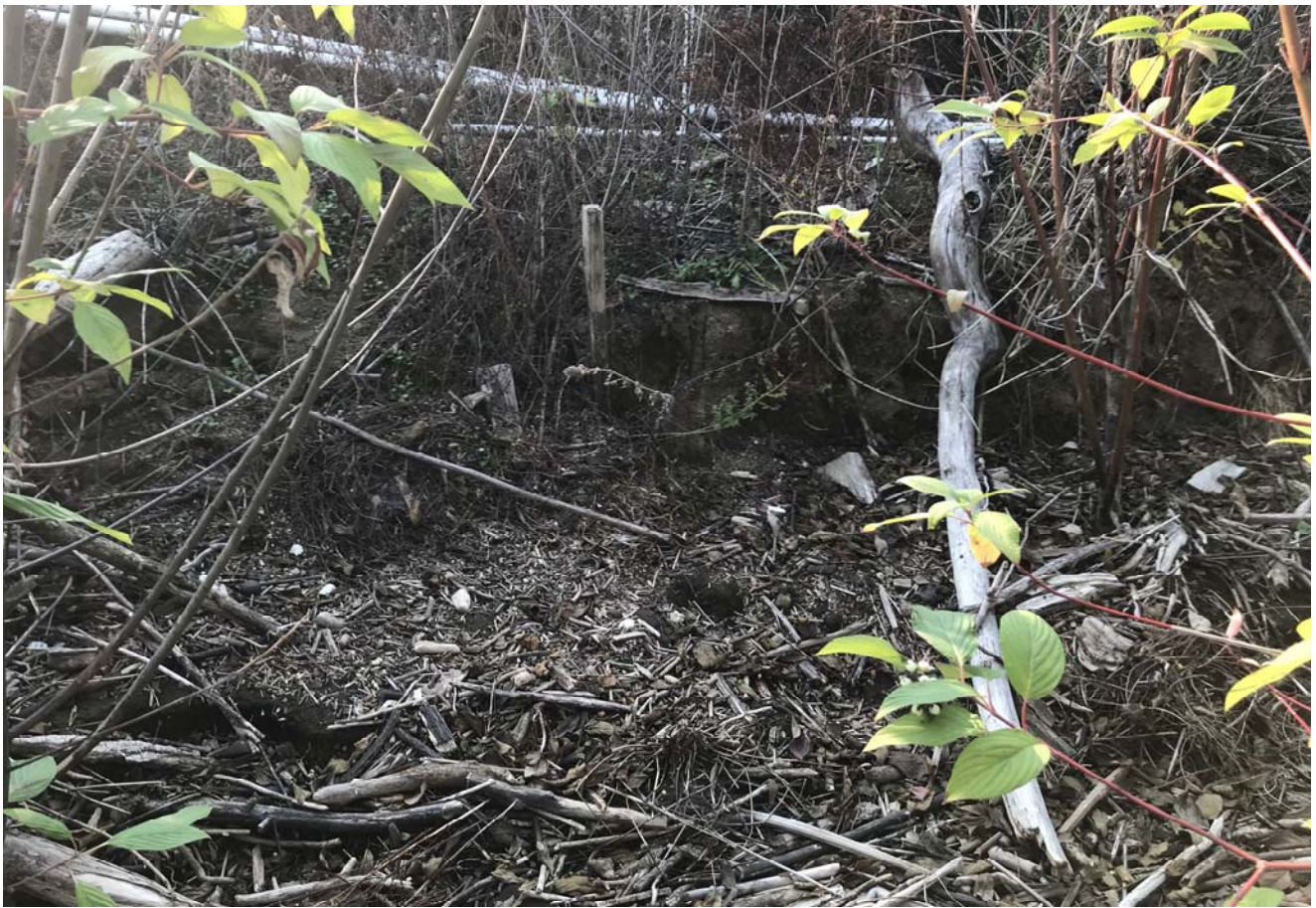
STA: 22+00 - Bank erosion elevations 11'-18' COP
