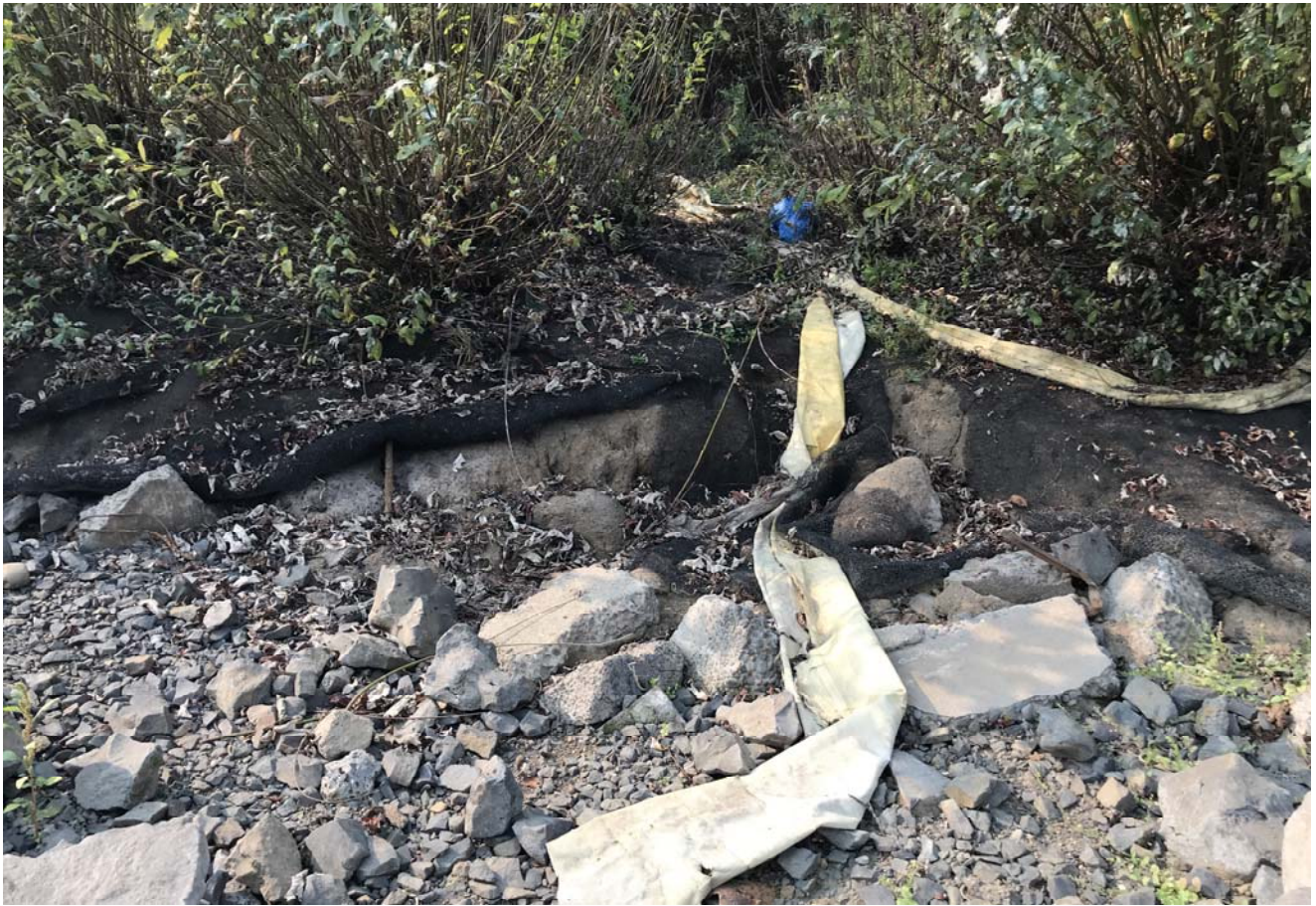
STA 0+20 - Exposed TRM and visible soil, negligible change from 2019 inspection
