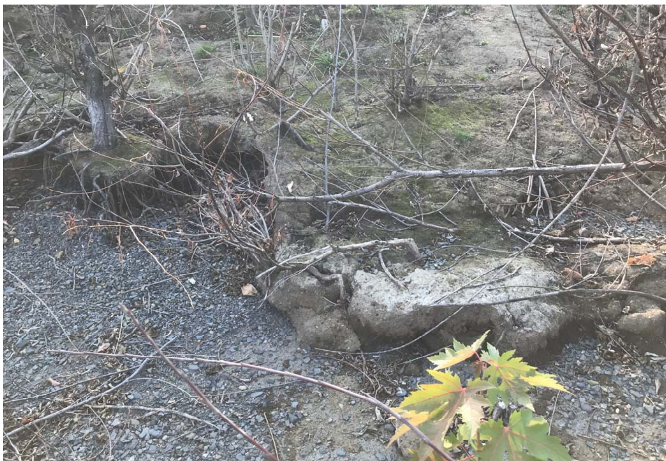
STA: 25+75 - Lower bank erosion below elevation 16'
