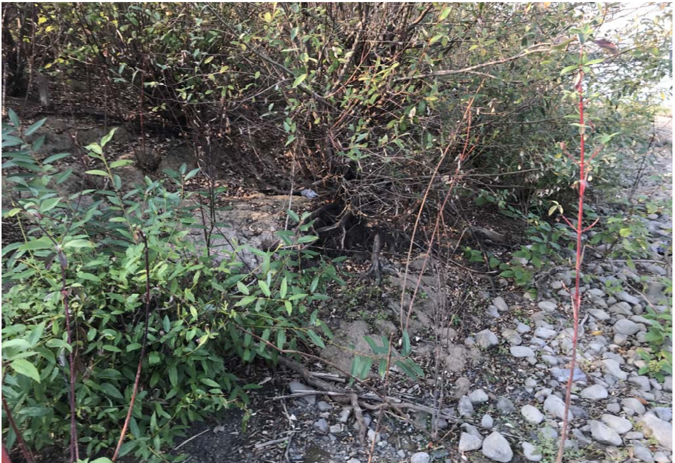
STA: 24+25 - Lower bank erosion elevation 11'-18'
