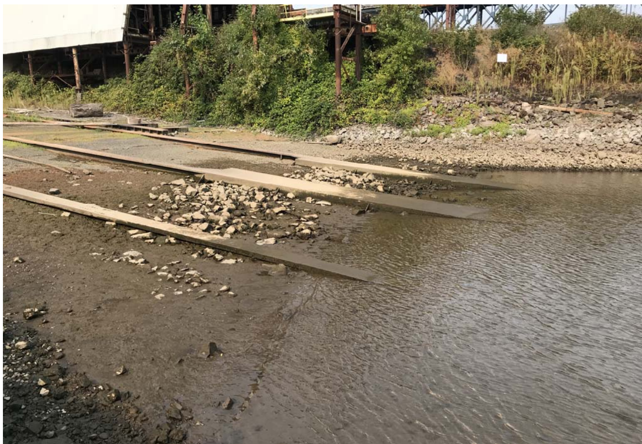
Slipway rails and sedimentation
