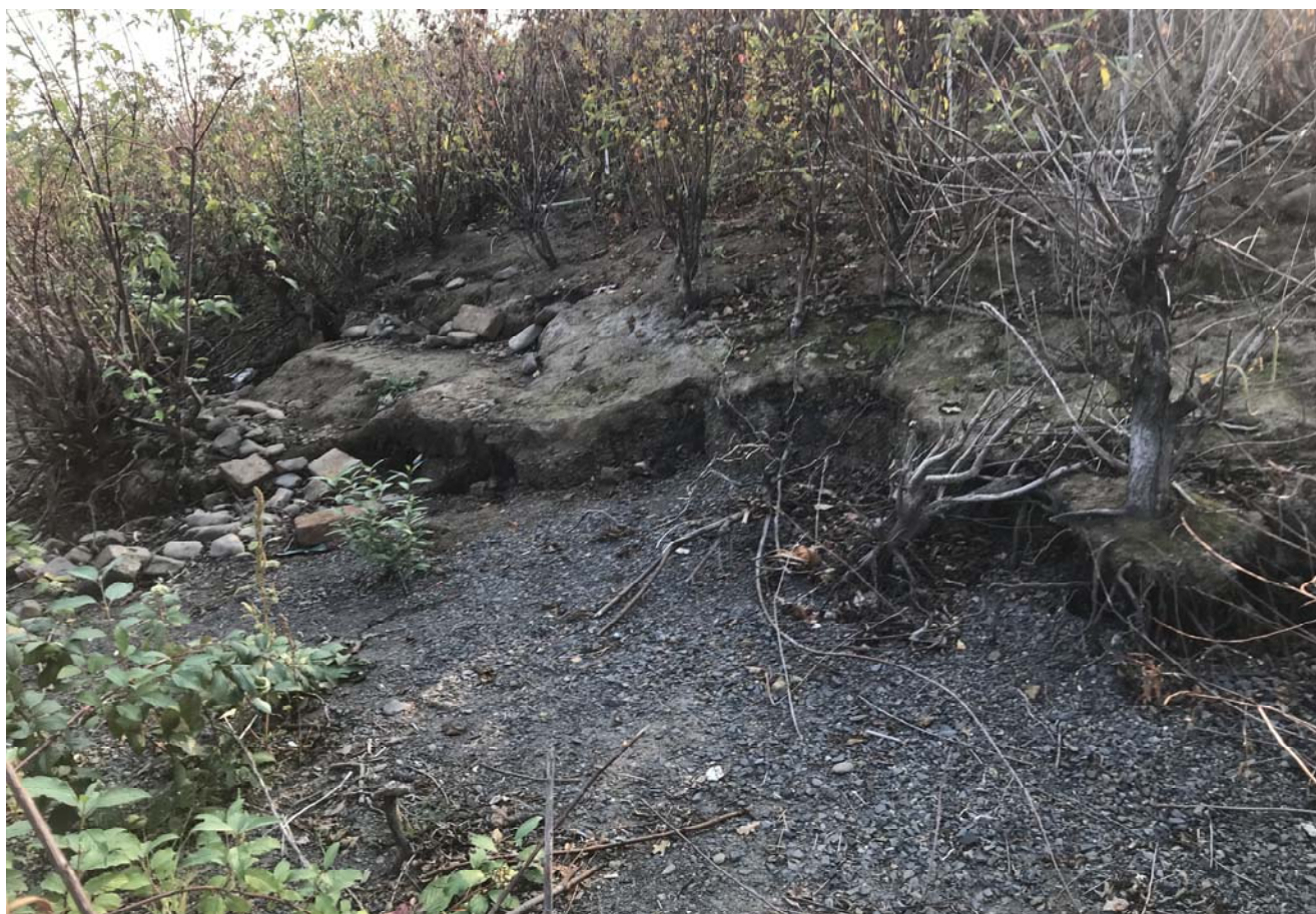
STA: 26+00 - Lower bank erosion below elevation 18'
