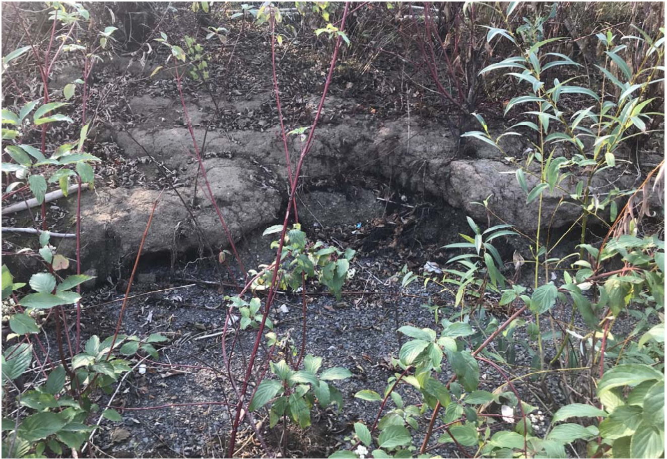
STA: 24+00 - Lower bank erosion elevation 11'-18'
