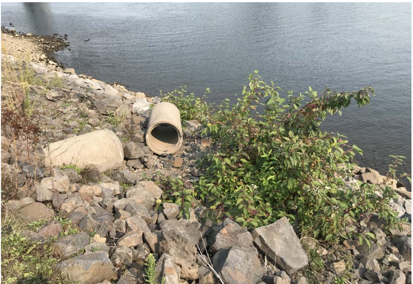
Stormwater outfall pipe segment separated, no change since previous inspections
