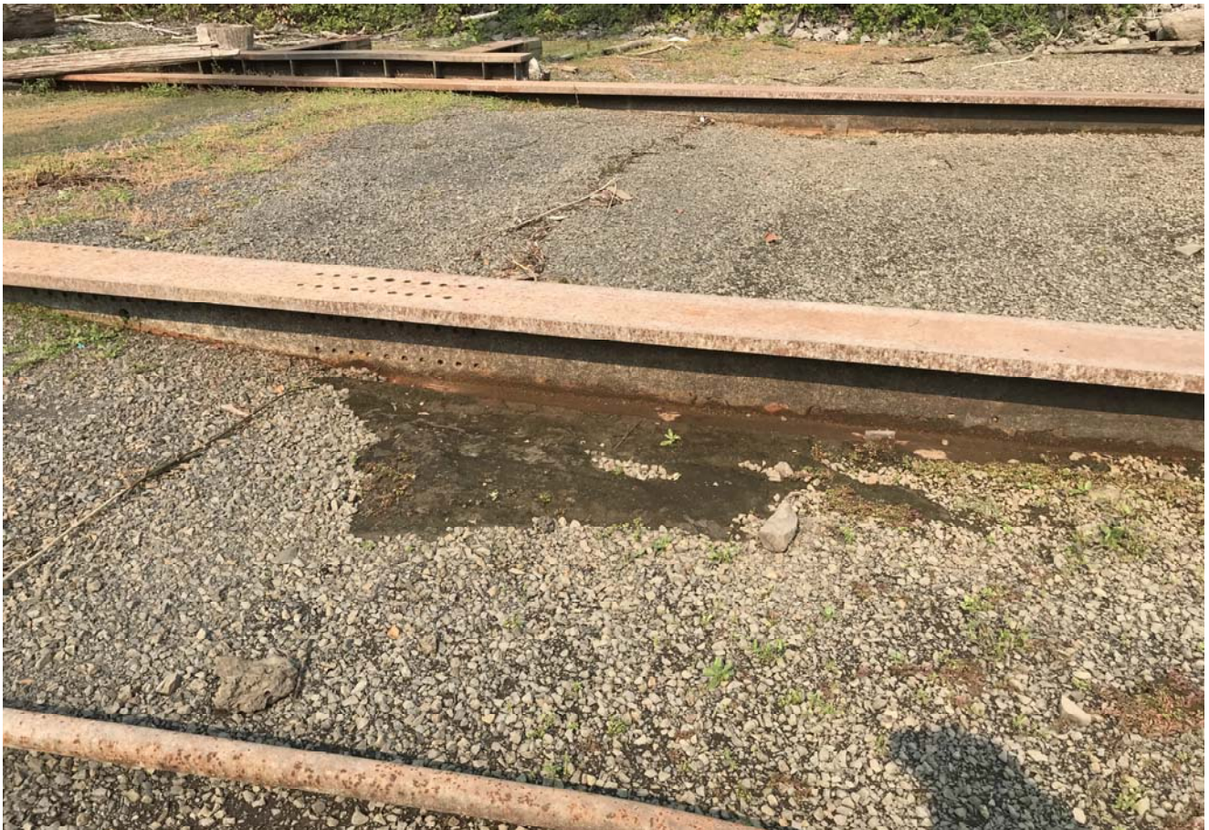
Minor area of exposed RCM adjacent to center rail, area is stable
