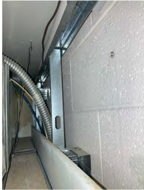
Photo 10 - View of sample location KP75 in the medical office admin area. The off-white crumbly coating material on the CMU wall has 2% chrysotile asbestos. (10/29/2024)
