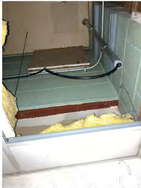
Photo 8 - View of sample location KP72 in the landscape shop. The green crumbly coating material on the CMU walls has 2% chrysotile asbestos. (10/29/2024)
