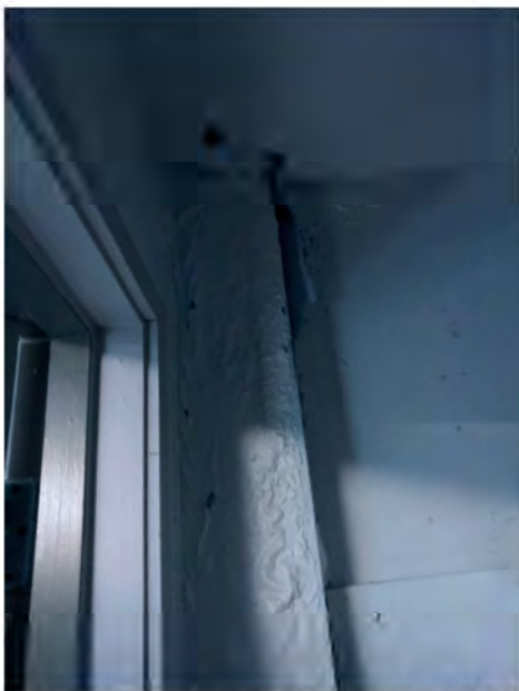
Photo 7 - View of sample location KP8p, an off-white paint on wood and gypsum wallboard in the landscape office. (11/10/2023)
