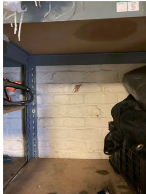
Photo 10 - View of sample location KP12p, an off-white paint on the brick wall in the landscape area garage bay. (11/10/2023)
