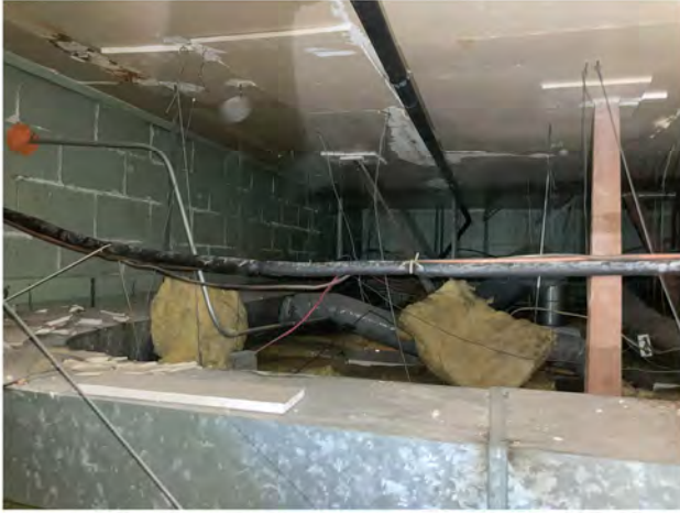
Photo 5 - View of sample locations KP49 (electrical room, back wall) and KP73 (restroom, side wall) taken from above the drop down ceiling. The green crumbly coating material on the CMU walls has 2-3% chrysotile asbestos. (11/10/2023)
