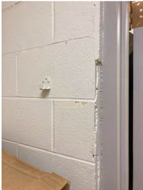
Photo 9 - View of sample location KP10p, an off-white paint on wood and CMU walls in the landscape area restroom. (11/10/2023)
