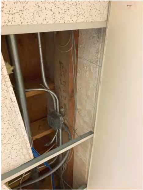
Photo 9 - View of sample location KP74 in the landscape breakroom. The off-white crumbly coating material on the CMU walls has 2% chrysotile asbestos. (10/29/2024)
