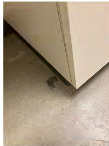
Photo 4 - View of sample location KP10 in the medical office breakroom. The black mastic associated with the gray patterned SVT flooring has 5% chrysotile asbestos. (11/10/2023)
