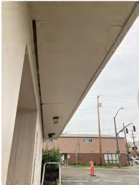
Photo 7 - View of sample location KP63 on the east side of the building. The cement board soffit material has 37% chrysotile asbestos. (11/10/2023)
