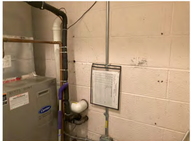
Photo 6 - View of sample location KP7p, an off-white paint on the CMU wall in the medical office utility room. Sample KP18p was collected from the opposite wall. (11/10/2023)
