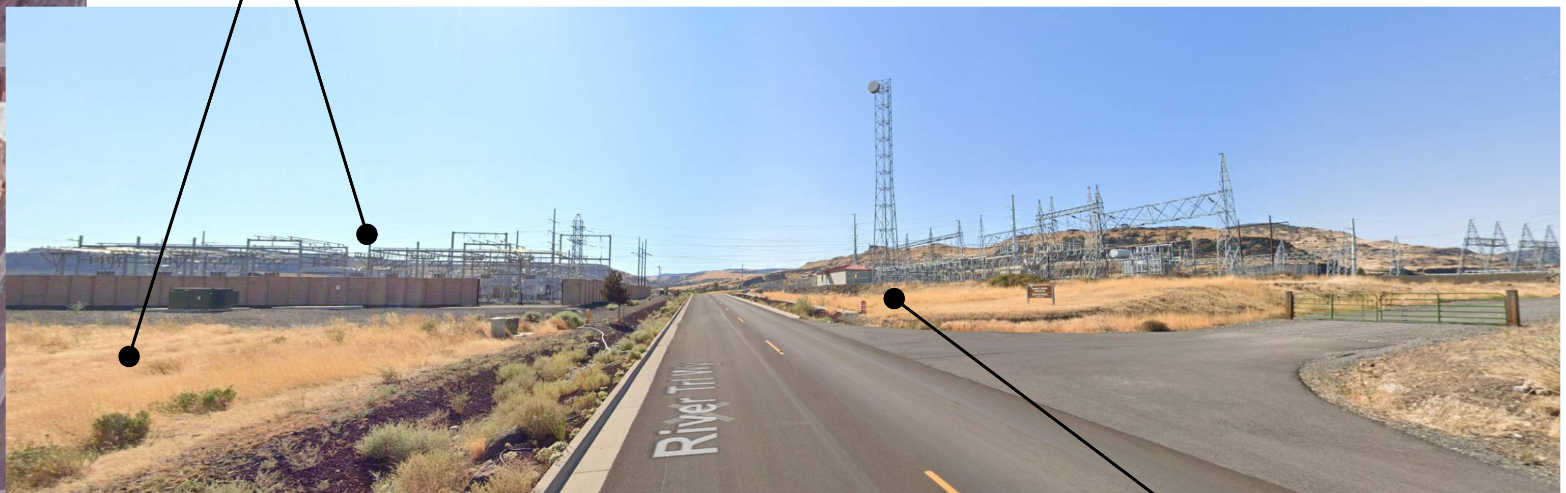
4290 River Trl Way AND ADJACENT PROPERTY WITH UTILITY INFRASTRUCTURE
