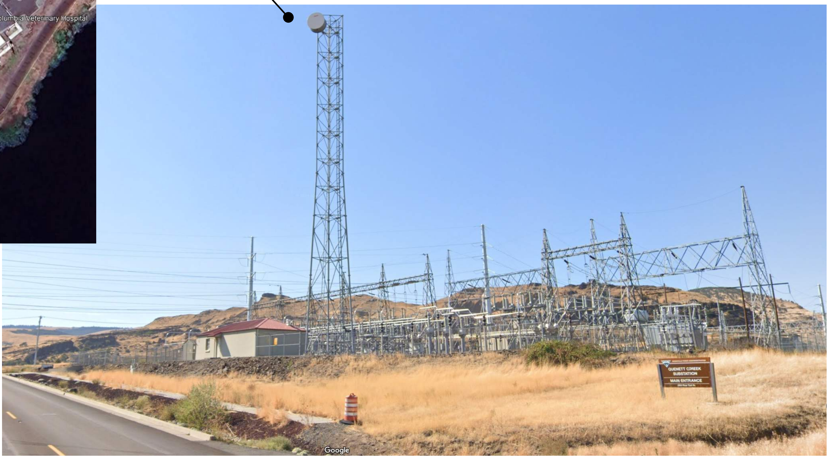
EXISTING TELEMETRY TOWER ACROSS THE STREET
