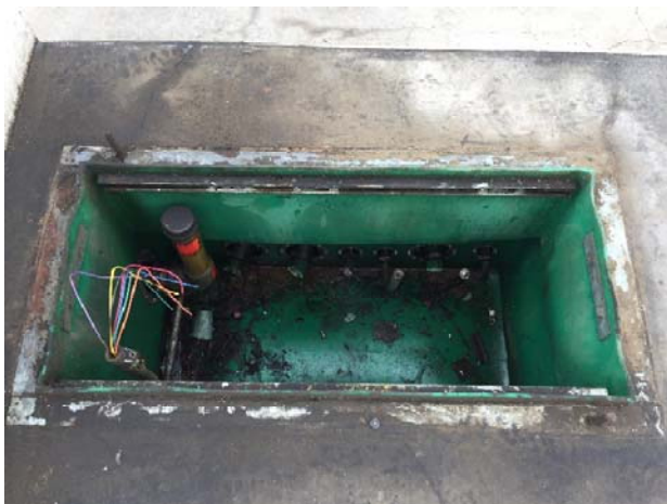
3. Fuel pump and electrical junking box.
