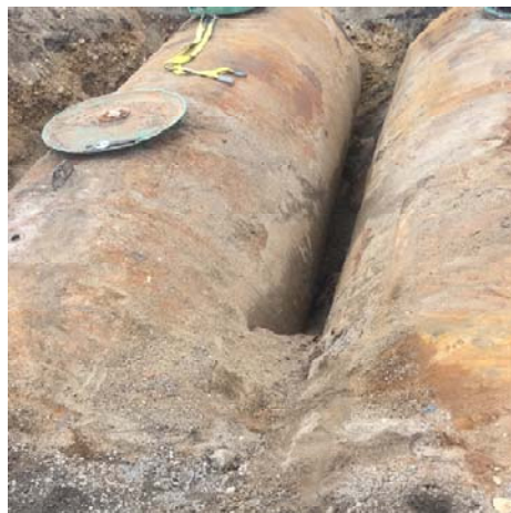
12. Underground storage tanks, facing north.
