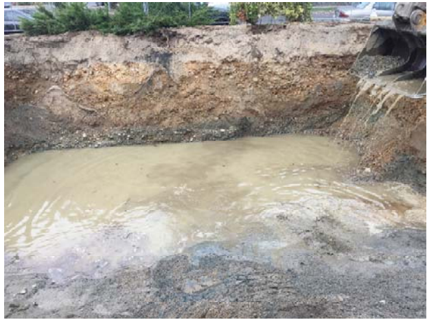
16. Tank pit, facing the north sidewall, and S10 and S13 sample locations.
