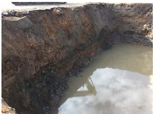
18. Tank pit, facing the south sidewall, and S14, S15, and S16 sample locations.
