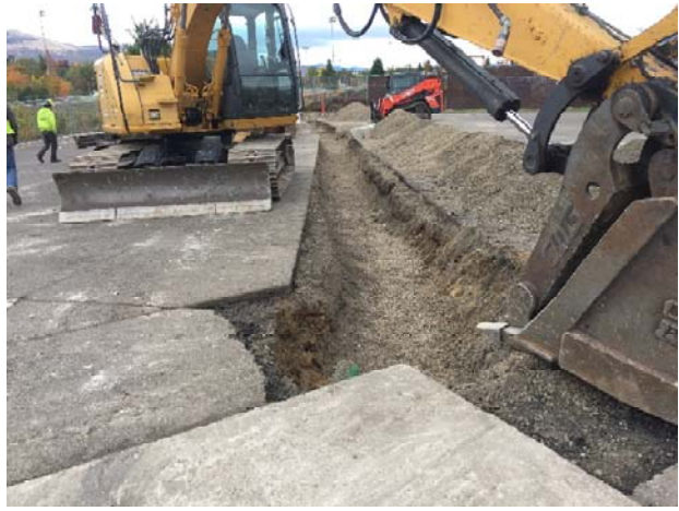
4. Fuel line trench, to former fuel pump satellites, facing southeast from fuel tanks.
