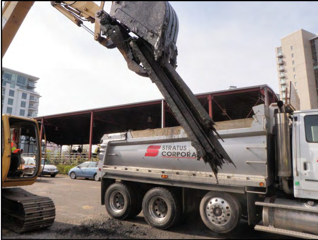
Photograph B-3: Current condition of cribbing
