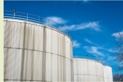
Bulk fuel storage
