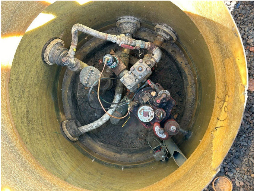
11: Tank top sump #1
