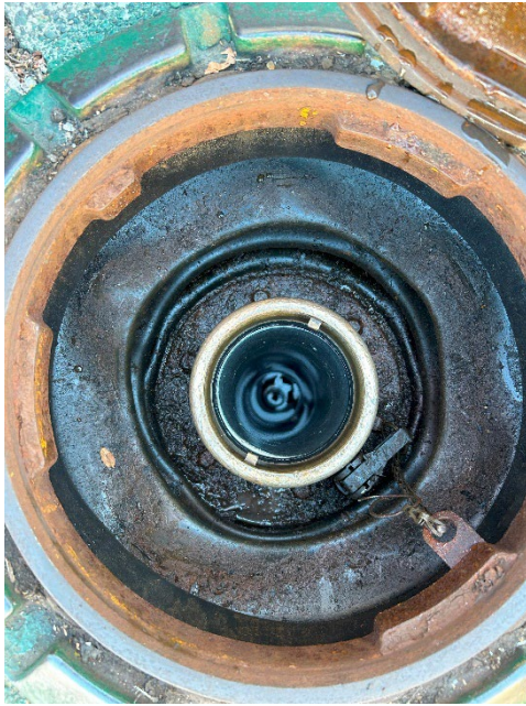
3: Diesel spill bucket
