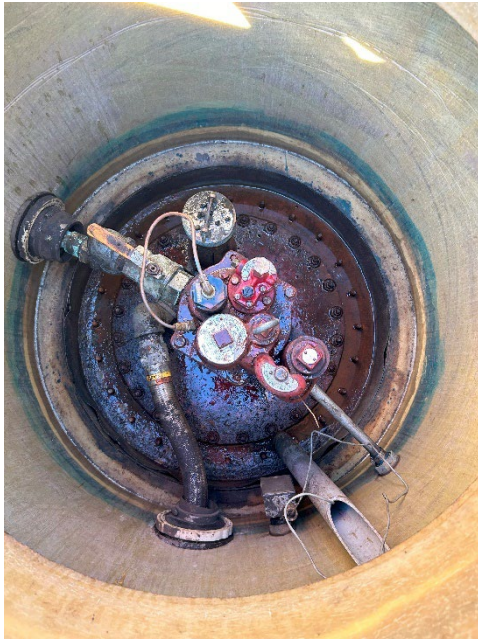
17: Tank top sump #3
