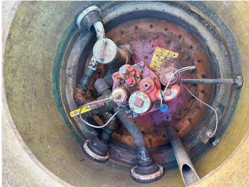
13: Tank top sump #2
