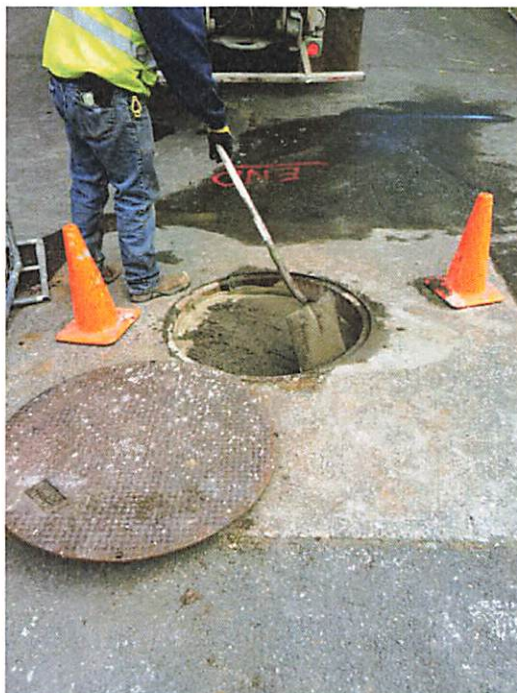
Photo 6. Gasoline tank filled with CDF.
