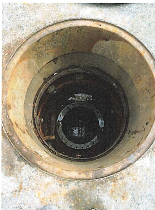
Photo 4. View of the interior of the diesel UST.
