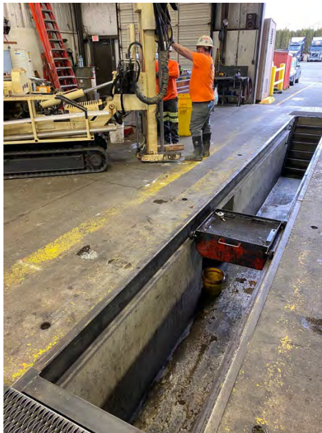
Photo 4. View east of drilling Boring B-15 adjacent to the east alcove in the mechanic pit. Note seepage of gear oil at the wall-floor joint on the pit floor.
