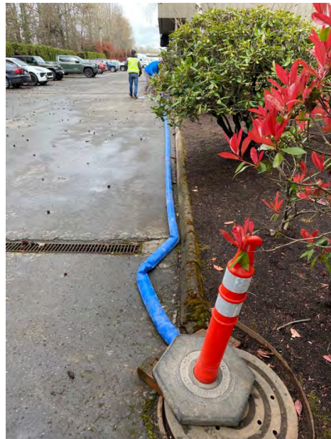
Photo 33. View west of the transfer hose from the Baker tanks to the City of Portland sanitary sewer.
