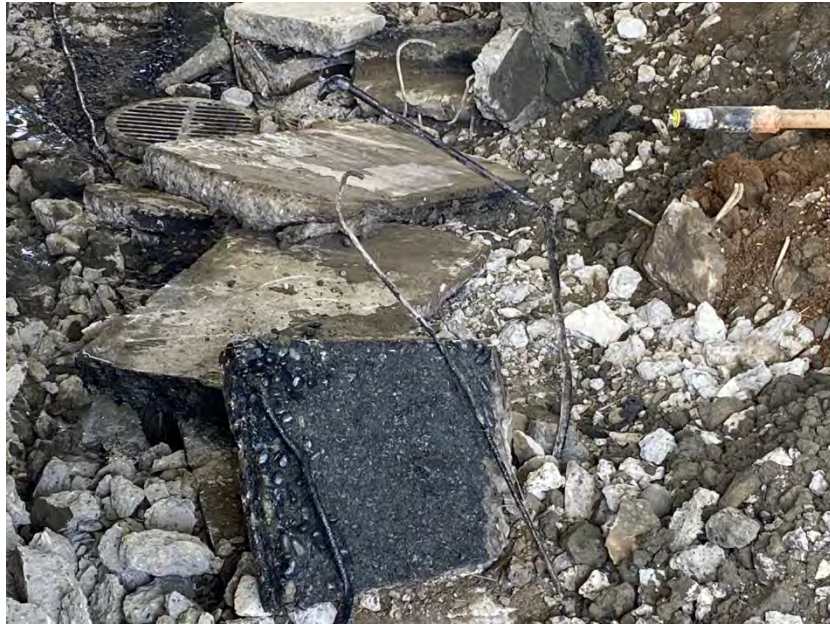
Photo 18. View of the broken-up slabs of the mechanic pit floor. Note the dark gear-oil stain on the slab bottom, as well as the tubing that transferred lubricants to the former hose reel alcoves.
