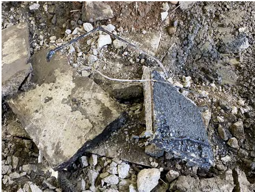
Photo 23. View of concrete pit floor slabs showing gear oil staining and lubricant tubing that was installed beneath the floor.
