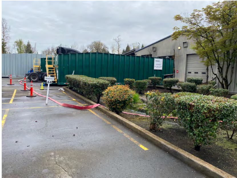
Photo 30. View north of the Baker tanks and the discharge hose along the west side of the truck shop and office building.
