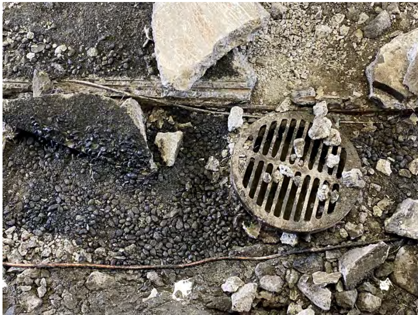
Photo 15. View of the sump for the mechanic pit. The concrete floor was removed exposing the gravel and tubing beneath. The dark stain is due to the gear oil release into the gravel.
