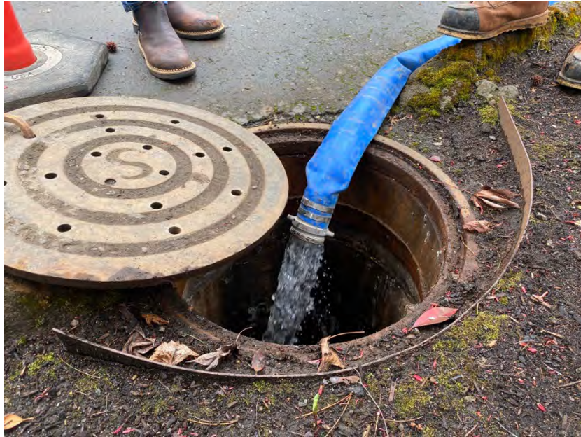
Photo 32. View of water from the Baker tanks approved for transfer to a City of Portland sanitary sewer.
