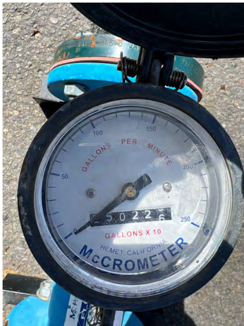
Photo 29. View of the meter that records the volume of tested groundwater approved for discharge to City of Portland sanitary sewer.
