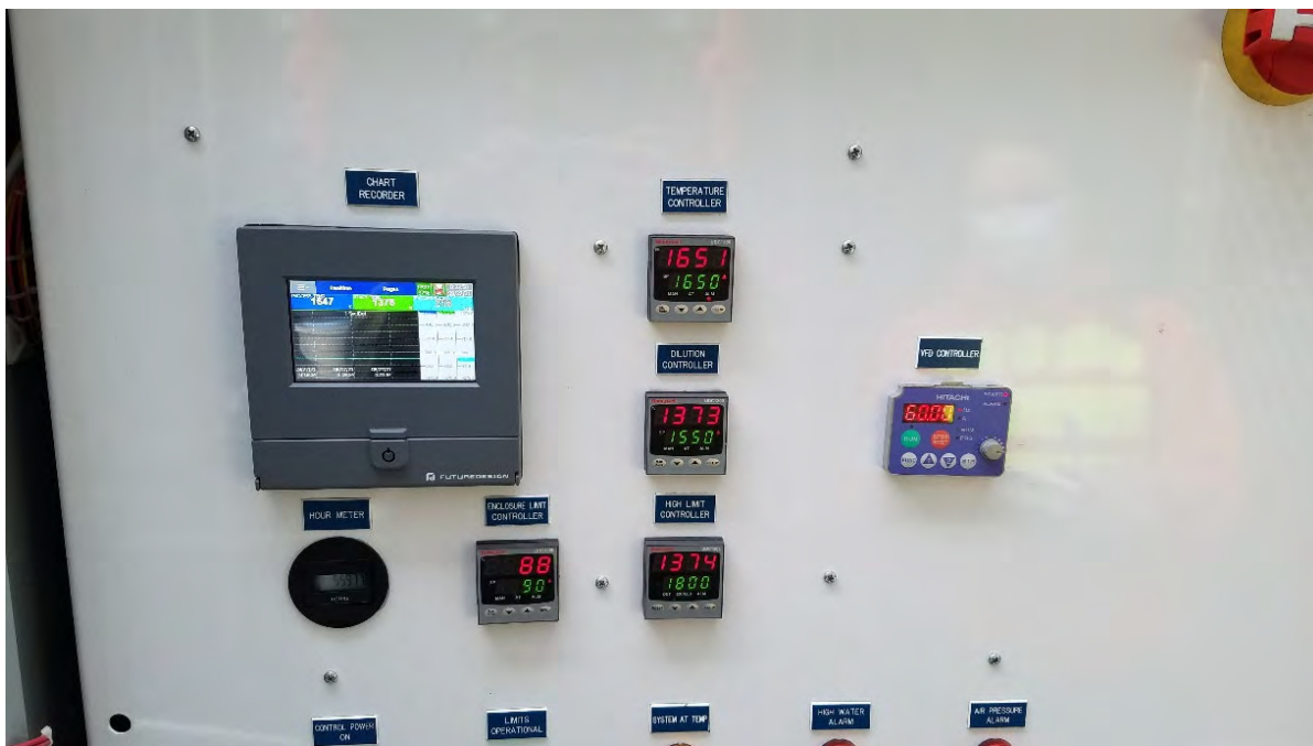
SVE SYSTEM CONTROL PANEL. PHOTOGRAPH TAKEN AUGUST 26, 2021.
