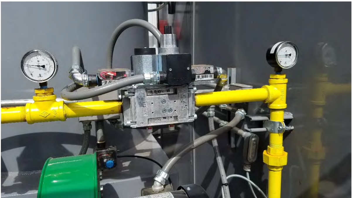
GAS SOLENOID VALVE ON SVE SYSTEM.
