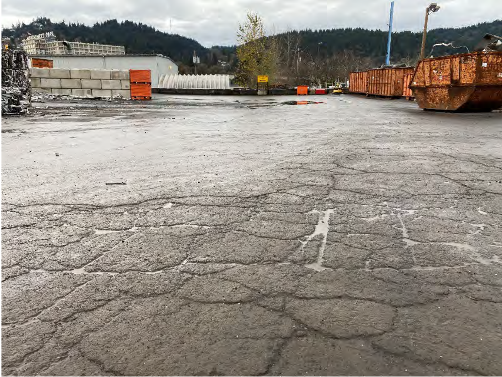
Photo 8 – Cracking on Calbag Metals Lot looking SW, outside of area paved in 2019
