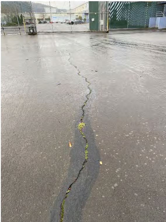
Photo 7 - Cracking in NE of Site Looking West
