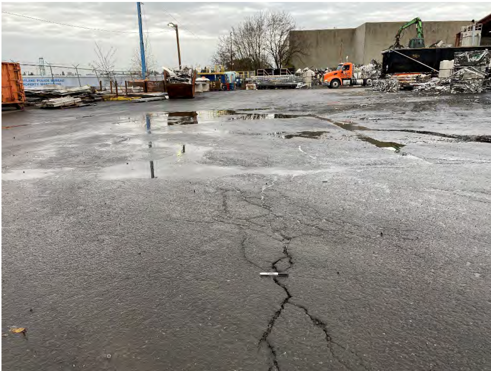
Photo 9 – Cracking on Calbag Metals Lot looking NE, outside of area paved in 2019
