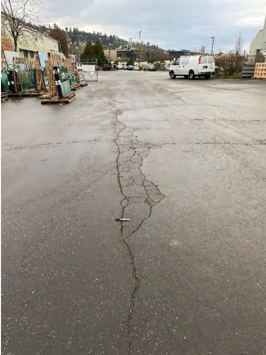
Photo 6 - Cracking in NW of Site Looking South
