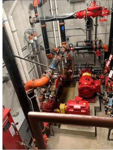
8. Fire pump room.
