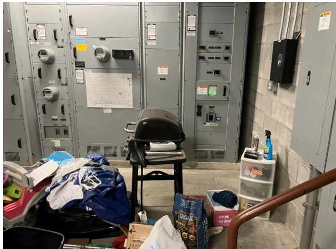
1. Electrical room in subterranean parking garage.
