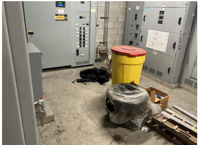
2. Electrical room in subterranean parking garage/building foundation.
