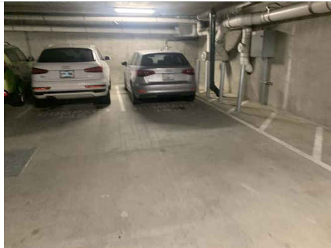
3. Utility penetration in parking garage/building foundation
