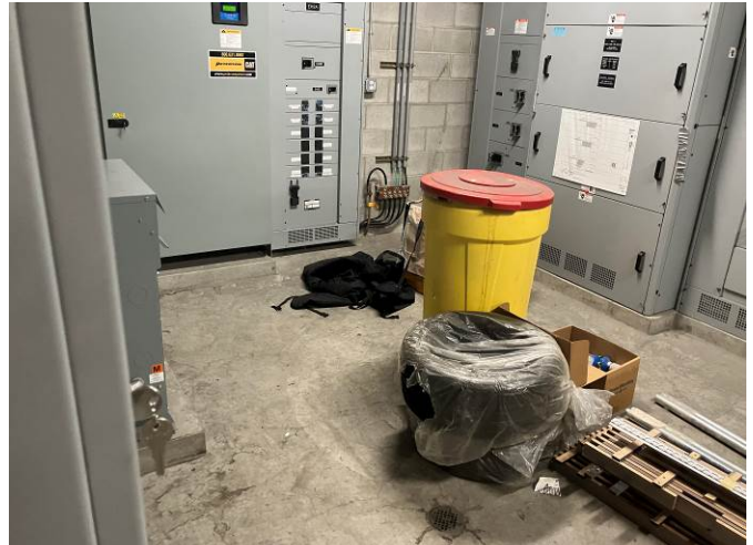
2. Electrical room in subterranean parking garage/building foundation.
