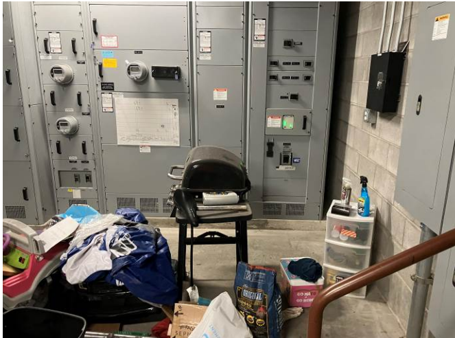
1. Electrical room in subterranean parking garage.
