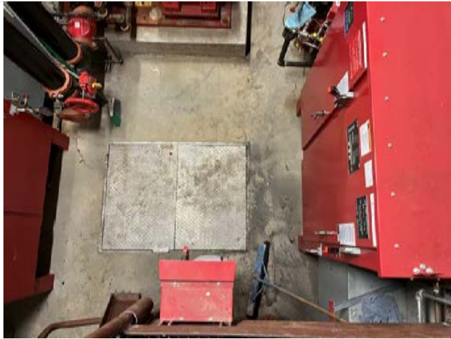
9. Fire pump room view from above
