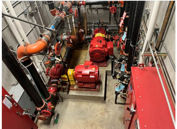
10. Fire pump room
