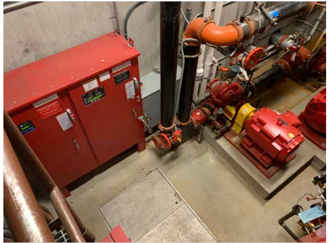
10. Fire pump room
