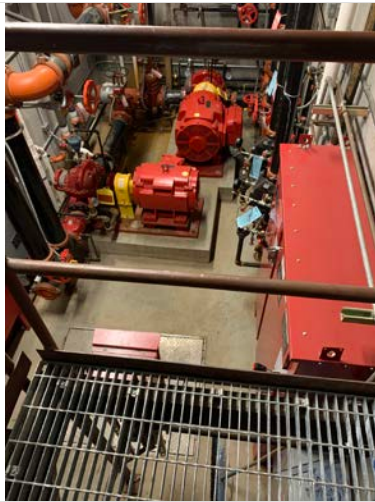
9. Fire pump room view from above
