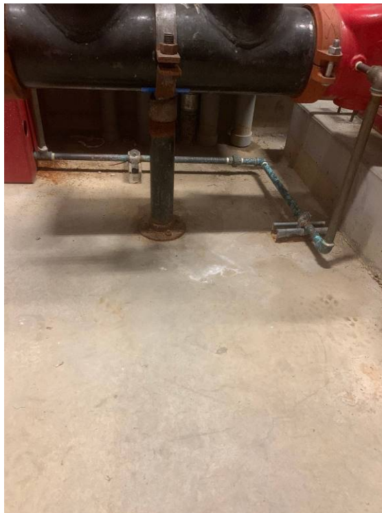
Photograph 8: Interior Pump Room A
