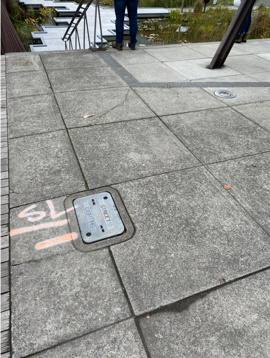
Photo Point 3 – cracks in asphalt have not changed since last year’s inspection
