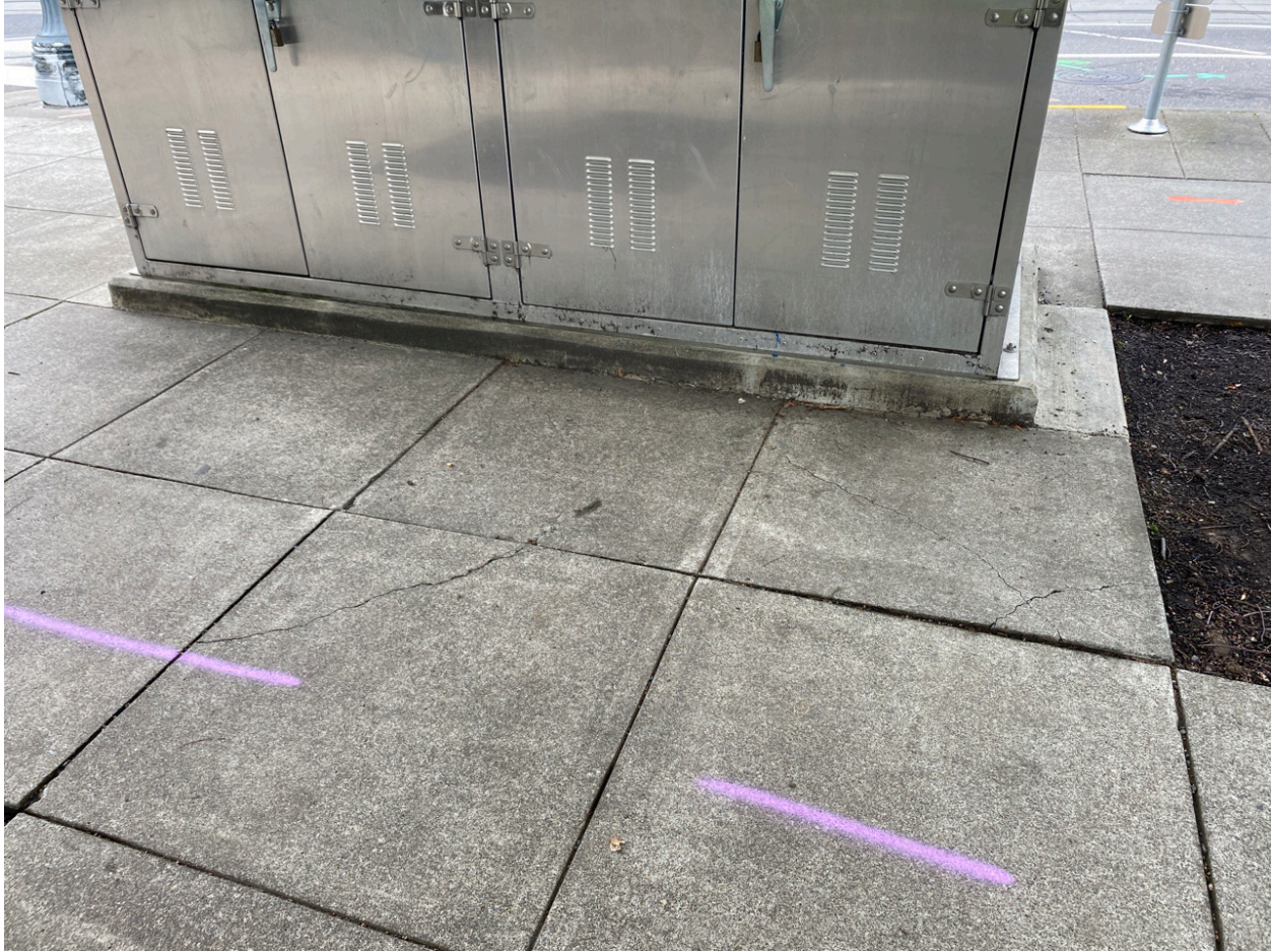
Photo Point 6 – Cracks in concrete panels near utility vault has not changed noticeably over the last couple of years
