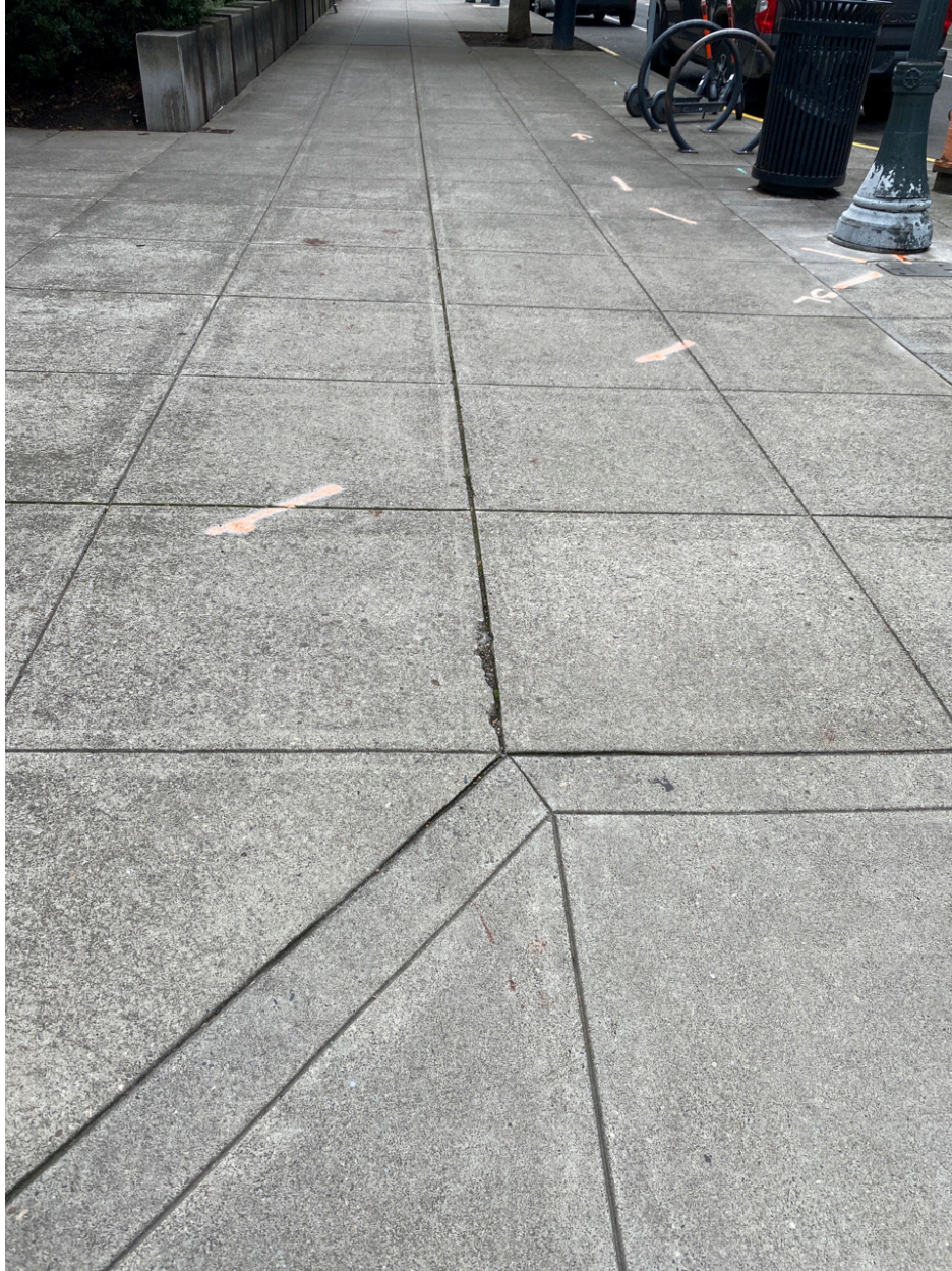
Photo Point 7 – looking south down sidewalk from northwest corner of the park. Cement in good condition, only minor surficial damage of one panel in this shot.
