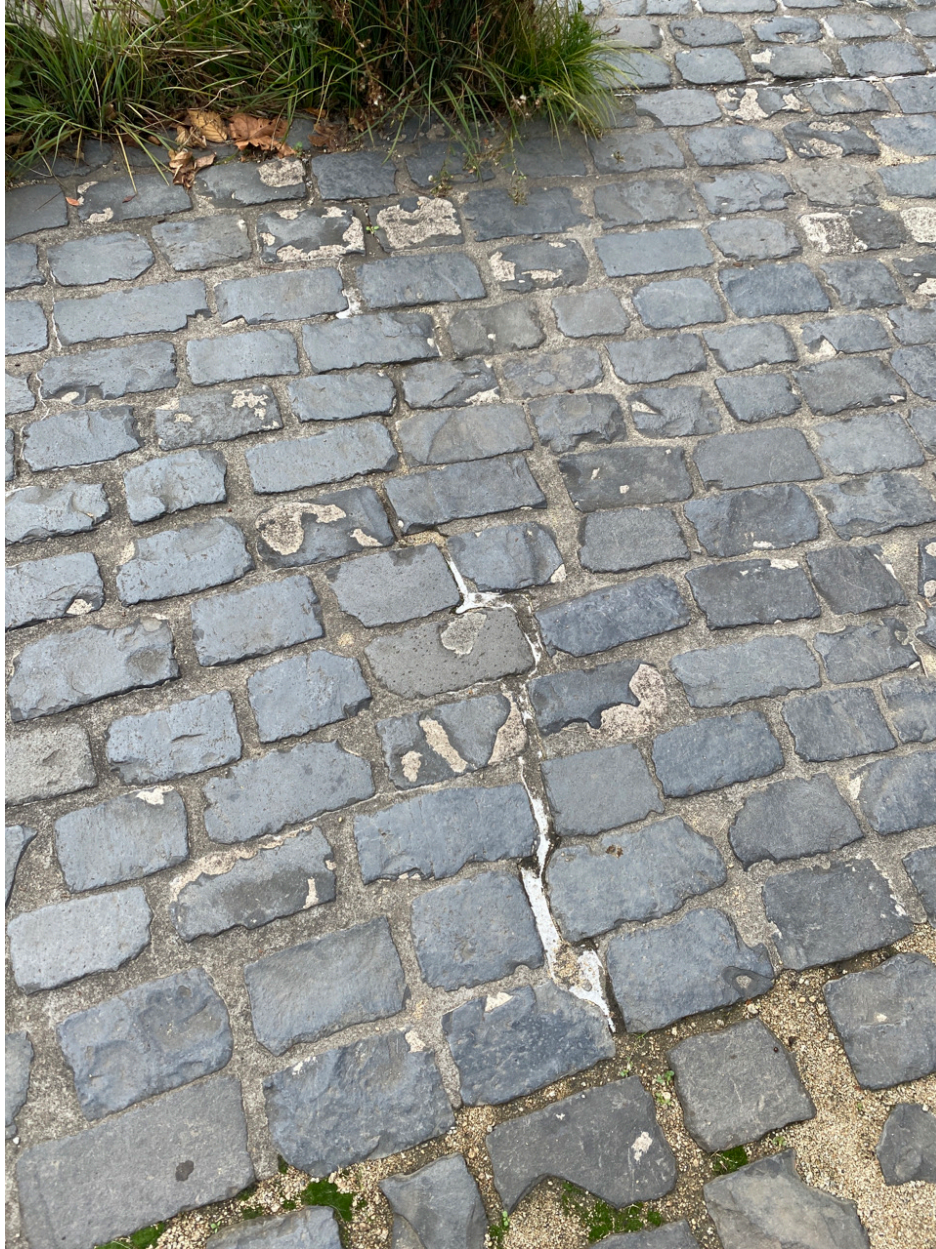
Photo Point 9 – Caulking used on cobblestone path in fair condition in some places, missing in others. However, none of the seams appear to be penetrating the cap.
