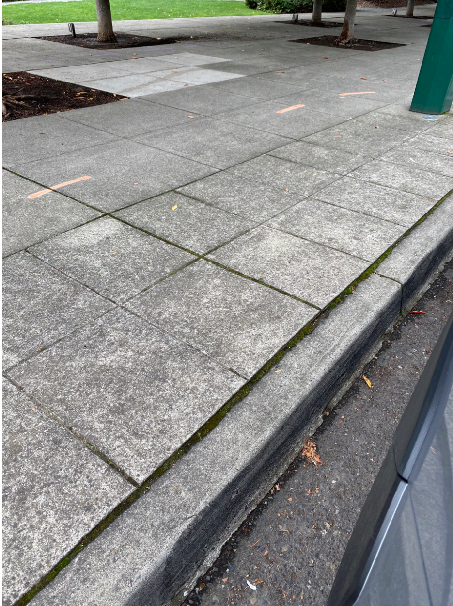
Photo Point 4 – cement panels uplifted less than 1 inch.
