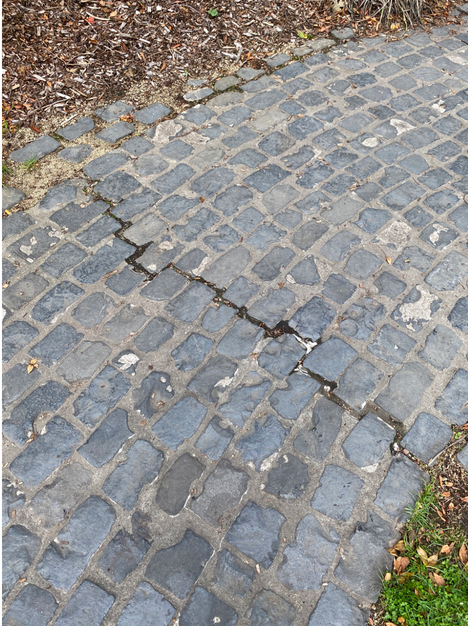
Photo Point 9 – seams missing in cobblestone path in a couple of locations where caulking appears to have been used before. None of the seams where caulking is missing are deep enough to penetrate the cap.
