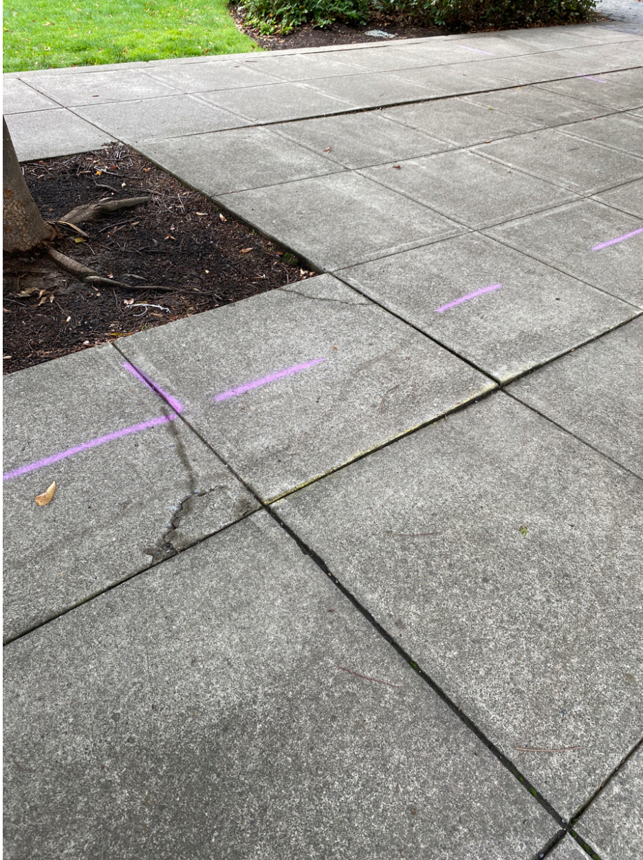
Photo Point 5 – minor cracks in cement panels around tree base. Likely caused by tree roots.
