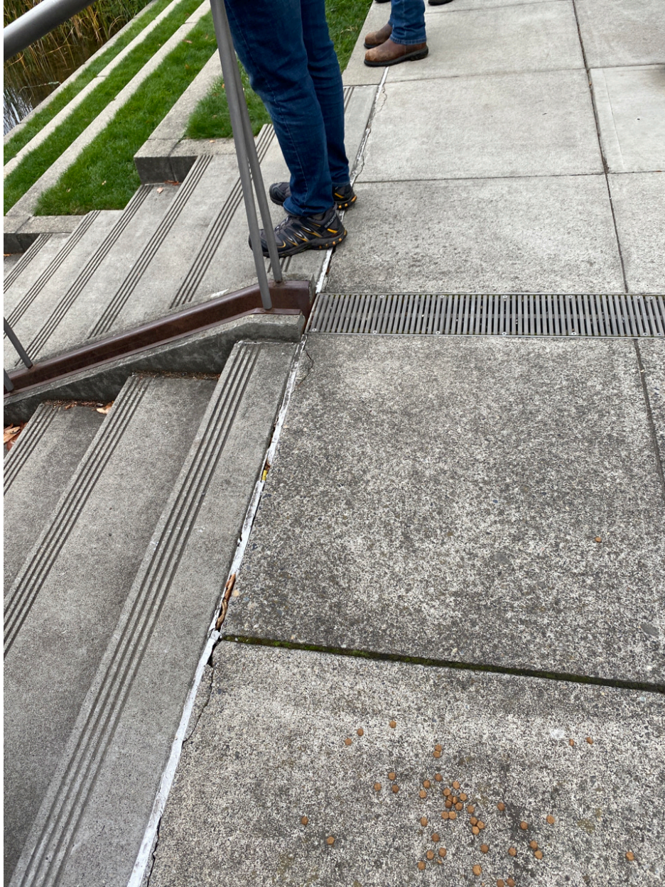
Photo Point 3 – cracks and worn caulking have not changed since last inspection
