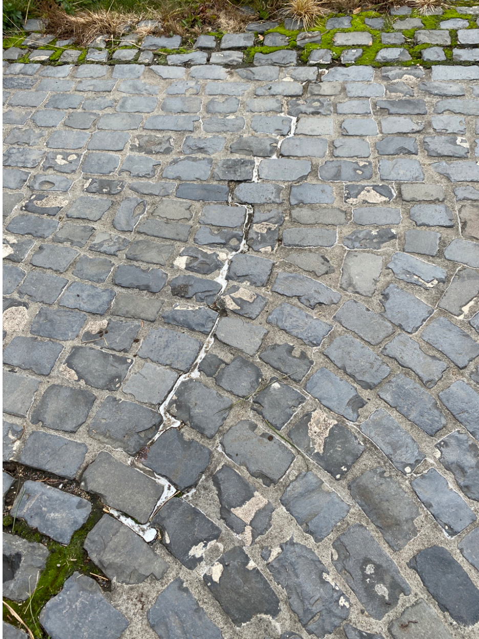
Photo Point 1 – condition of caulking in path. Fair condition, no cap penetration, no need for repair
