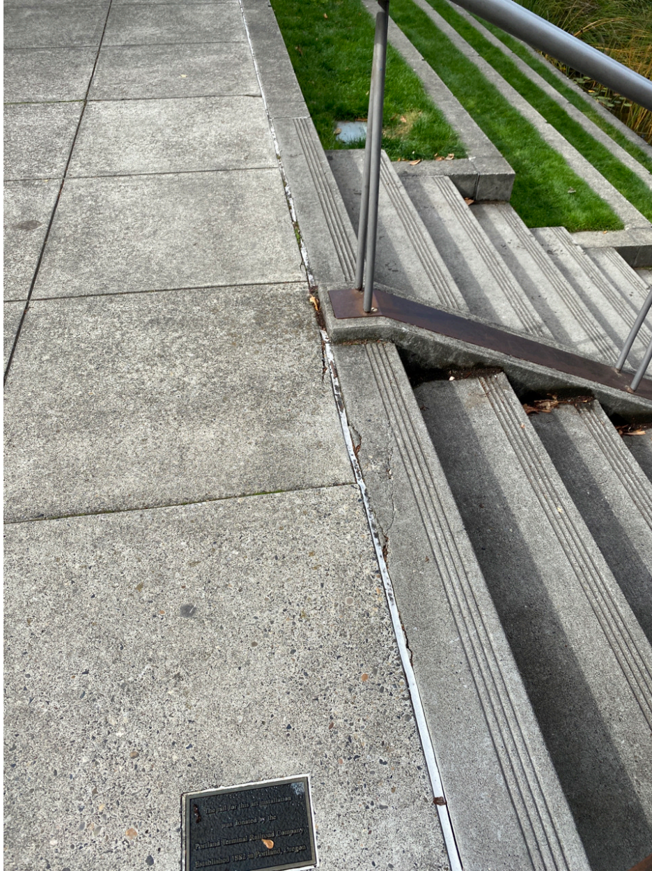
Photo Point 12 – Concrete and caulking at top of staircase at SEC of the park are in good to fair condition, appear similar in last year inspection report.
