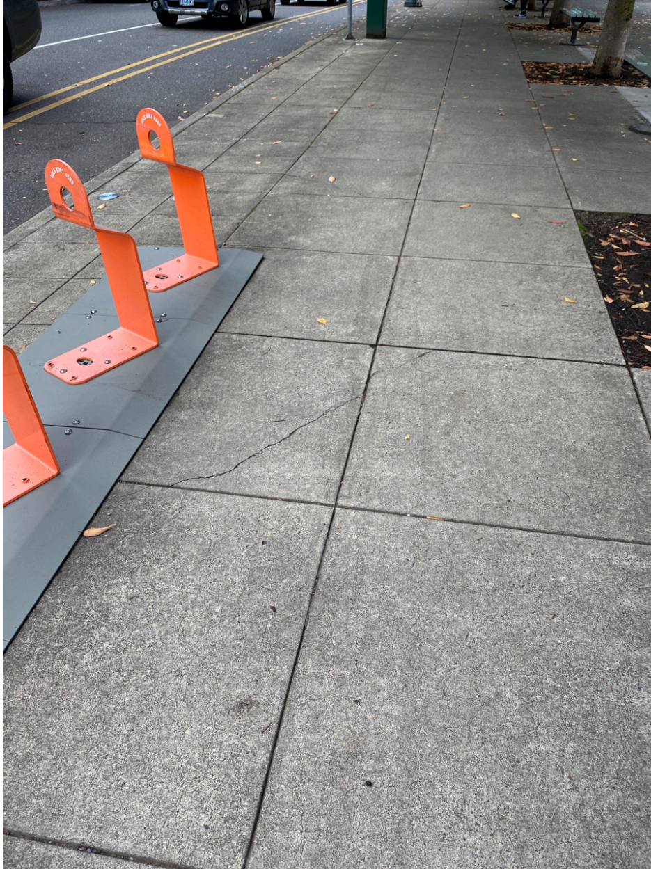
Photo Point 13 – cracks in concrete near Biketown station looks like last year’s inspection photo.
