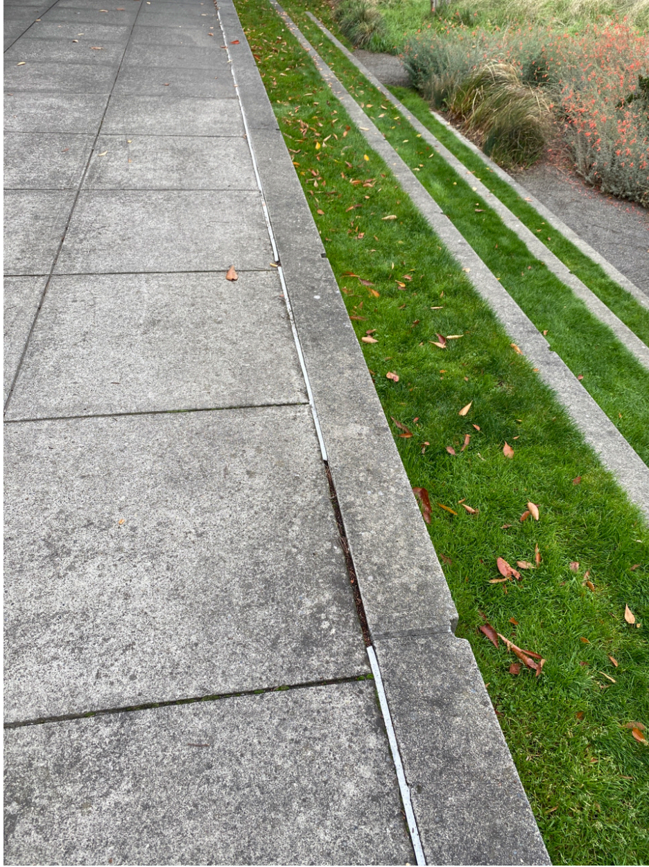
Photo Point 2 – small section (about 2 ft) of caulking missing from hardscape on top of terraced area. Does not penetrate or pose risk to the cap.
