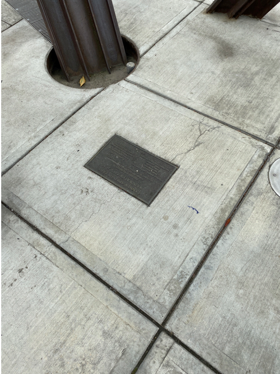
Photo Point 3 – small cracks in concrete noticed around plaque in sidewalk
