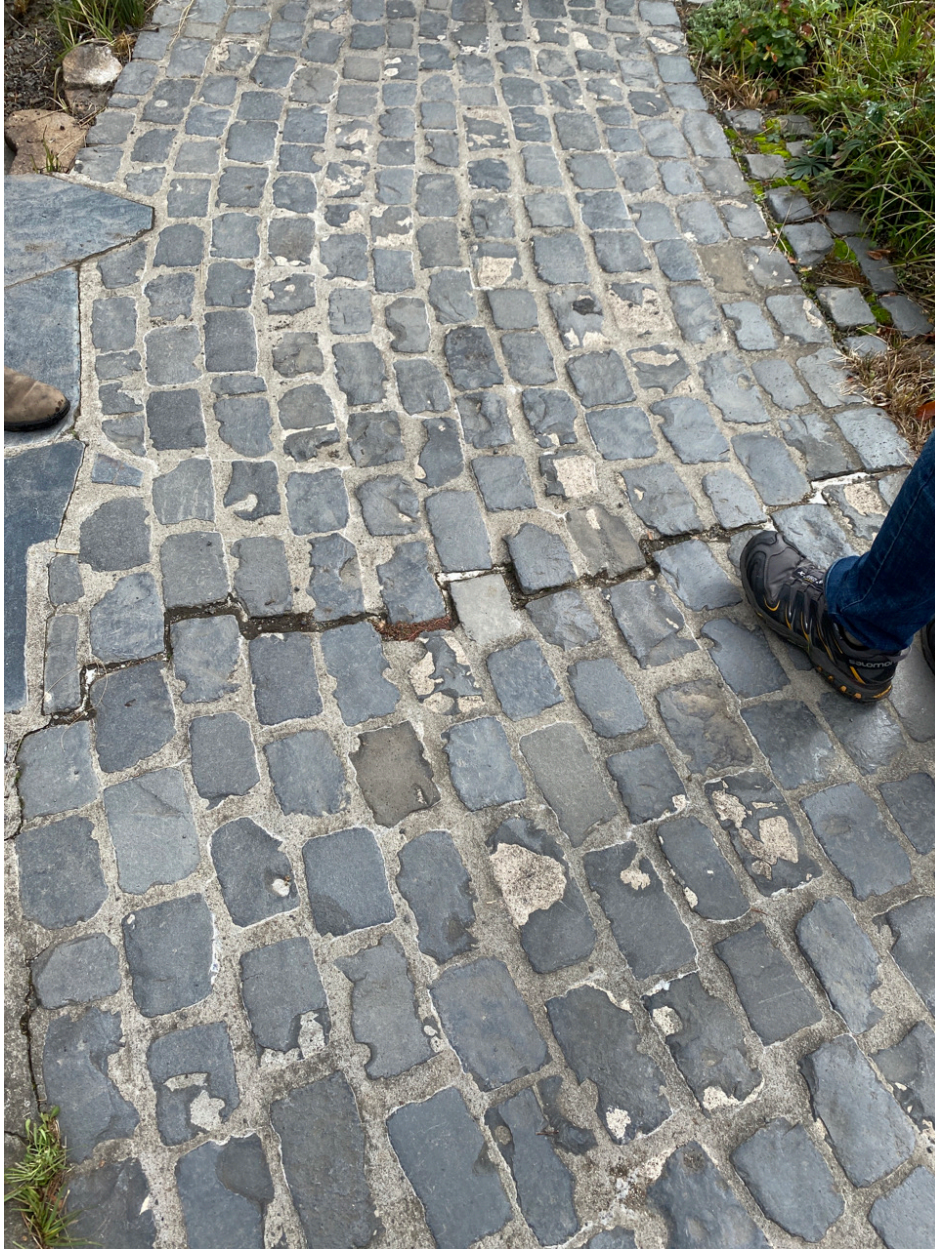
Photo Point 10 – caulking seam missing, worn, or overgrown with moss. Seam does not penetrate the cap.
