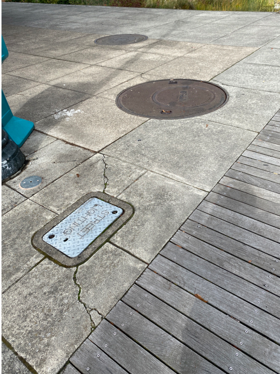
Photo Point 11 – cracks around street lighting vault have not changed since last year.
