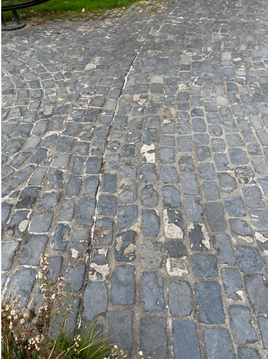
Photo Point 9 – Cobblestone path and seams in fair condition in most locations
