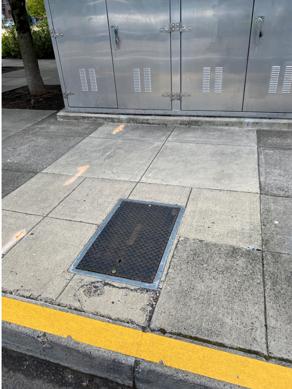
Photo Point 6 – surficial damage to concrete panel around utility vault near roadway. Does not expose soil.
