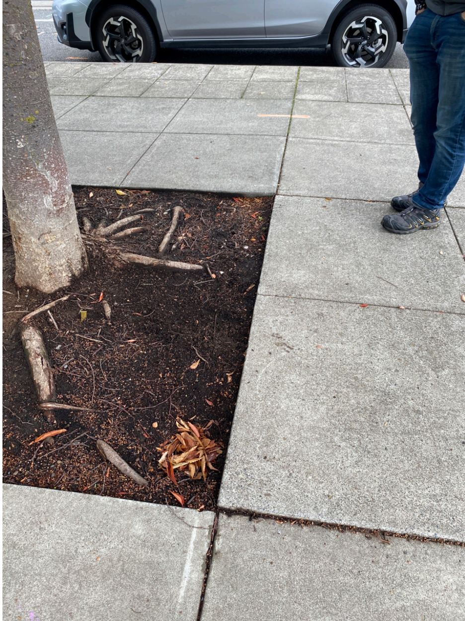
Photo Point 4 – Raised concrete panels from tree roots.
