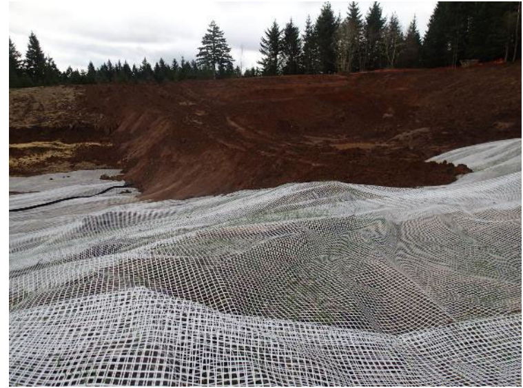
View south of buttress fill and soil cap beginning to be installed above the demarcation grid (March 2, 2018).
