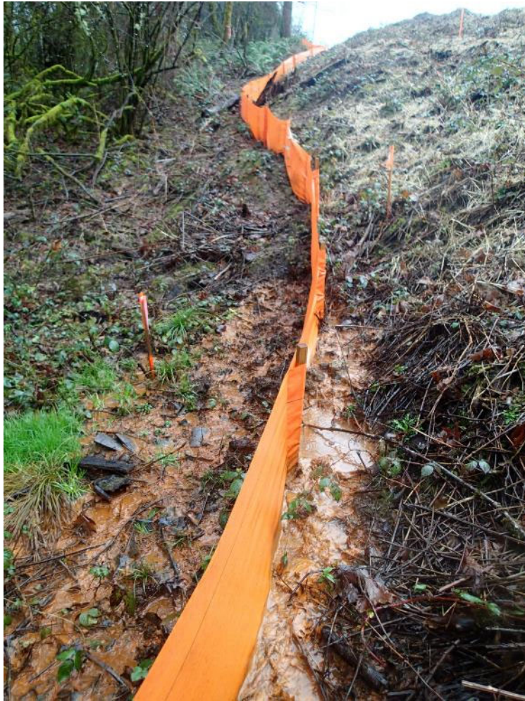
Seep at the landfill toe (January 18, 2018).
