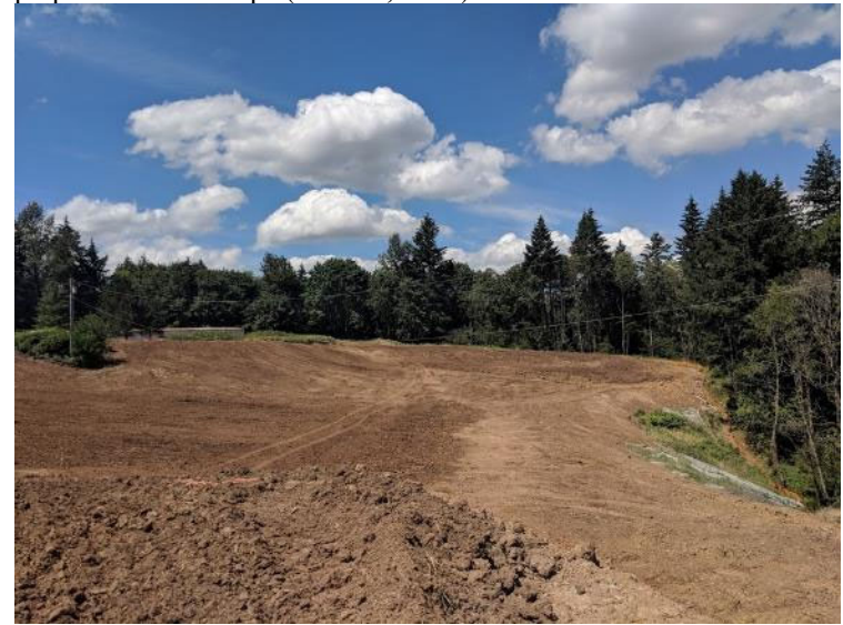
View north of the capped landfill from the vantage of the south buttress fill (July 6, 2018).
