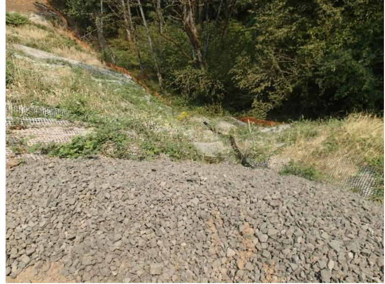
Drain rock was placed over the ravine drain line. Drain pipe exits at the eastern landfill boundary, which has not yet been capped as of this date (August 8, 2018).
