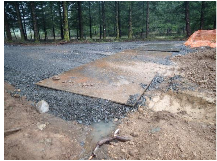
Steel plates positioned at unloading platform at the west margin of the landfill (January 18, 2018).
