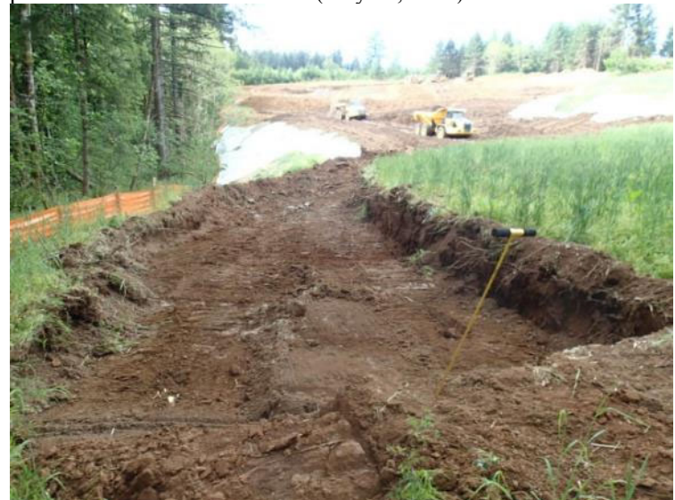
Keyway excavation along the east side of the north buttress fill - view south (June 1, 2018).
