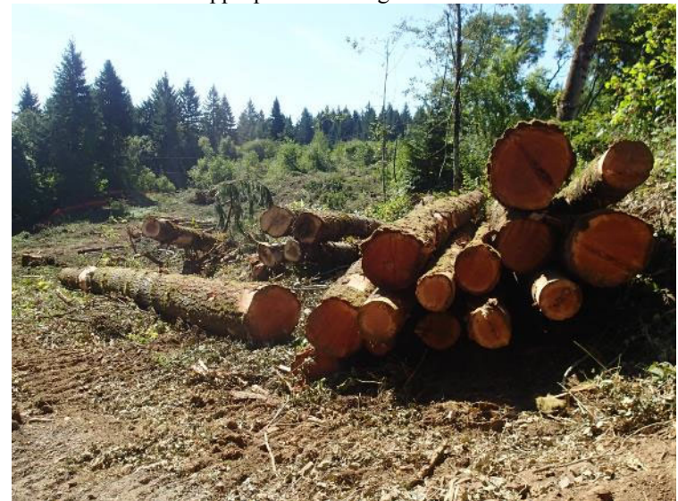
Surface of Troh Legacy Landfill was logged and cleared of brush - view south (August 16, 2017).
