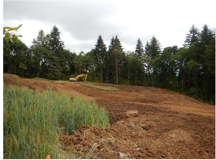
View north of cap at the north end of the landfill (June 7, 2018).
