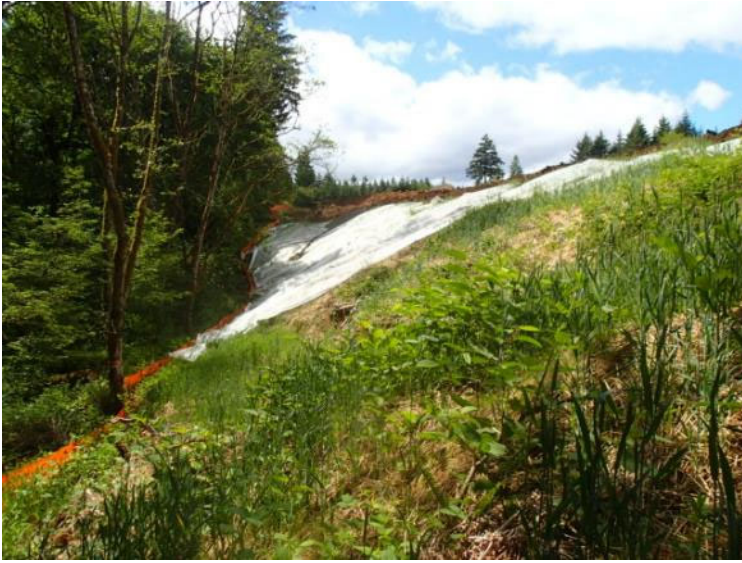
Demarcation grid installation along the east-central edge of the landfill - view south (June 1, 2018).
