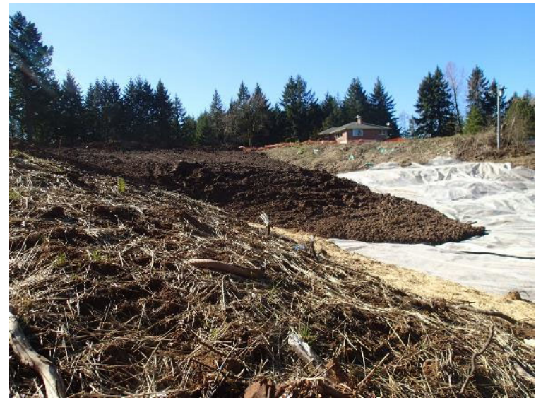
Continued cap installation over the demarcation grid on the southwest part of the landfill – view northwest (March 3, 2018).
