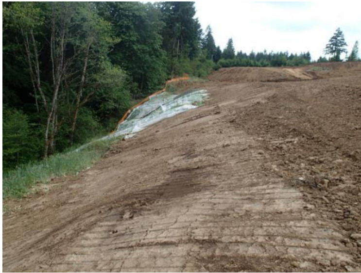
Cap along the east edge of landfill still needs to be completed where demarcation grid is visible (June 14, 2018).
