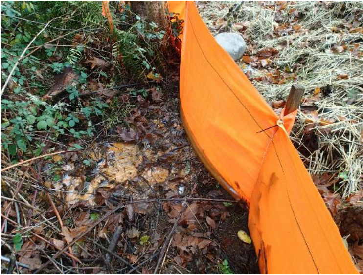
Seeps formed at the landfill toe (east) outside of the disturbed area (November 17, 2017).
