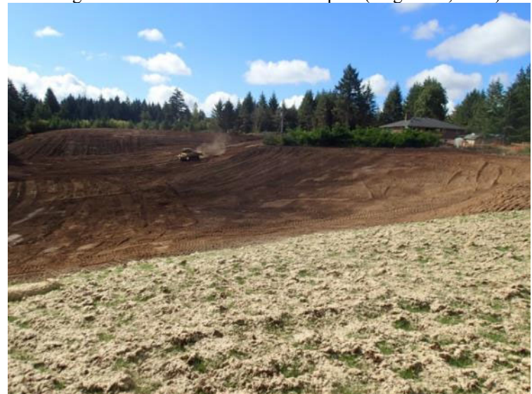
Grass has taken root on the north buttress fill, and the remainder of the landfill is being prepared for hydroseeding (September 14, 2018).
