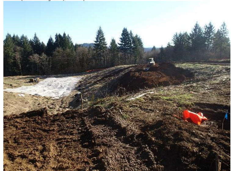
Construction of the buttress fill south of the landfill (right side of the demarcation represents the southernmost extent of the landfill) – view southeast (February 12, 2018).
