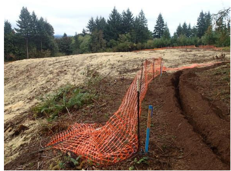
Water line to an east-adjacent residence was diverted around the landfill (October 13, 2017).
