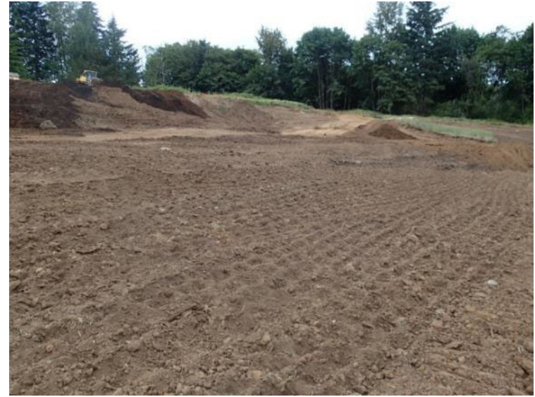
Cap surface was tracked and compacted with a sheepfoot roller perpendicular to slope (June 25, 2018).
