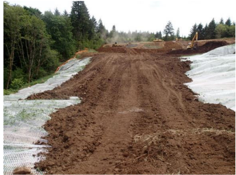
Soil cap being installed over the demarcation grid at the east-central part of the landfill – view south (May 30, 2018).
