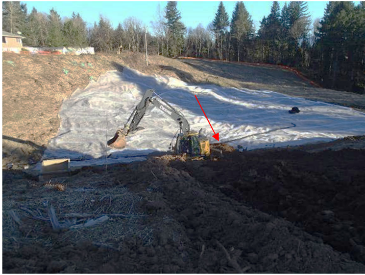
Demarcation placed over southwest corner of landfill. Note drain pipe placed along centerline of ravine – view north (February 13, 2018).
