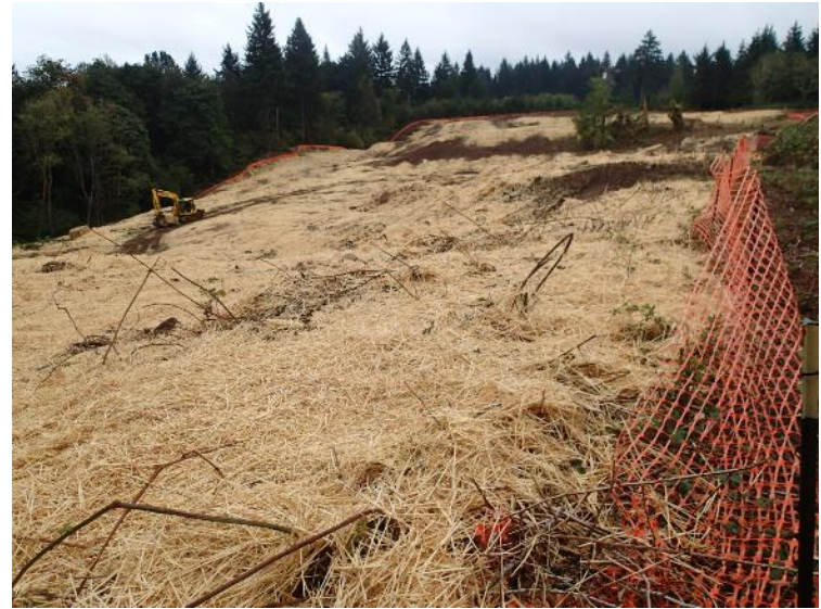
Straw was placed over the soil surface for erosion control purposes – view south (September 29, 2017).
