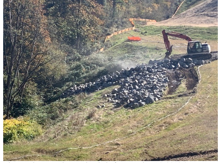
Rip-rap placement began shortly before October 14, 2019 (note, demarcation barrier is present beneath area where rip-rap was placed, however is obscured by growing grass).
