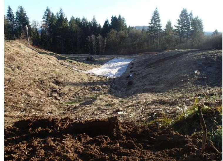
A portion of the demarcation layer rolled out over the landfill – view east (February 12, 2018).
