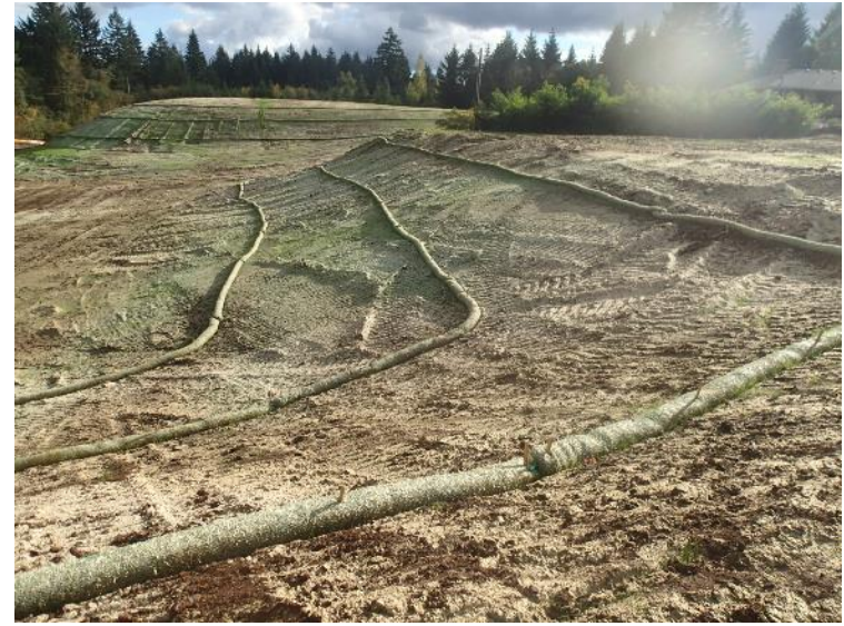
Straw wattles were placed on the remaining portions of the landfill, after which the ground surface was hydroseeded– view south (October 9, 2018).
