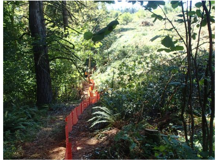
A silt fence was installed around the perimeter of the disturbed area – view of east boundary looking south (August 16, 2017).
