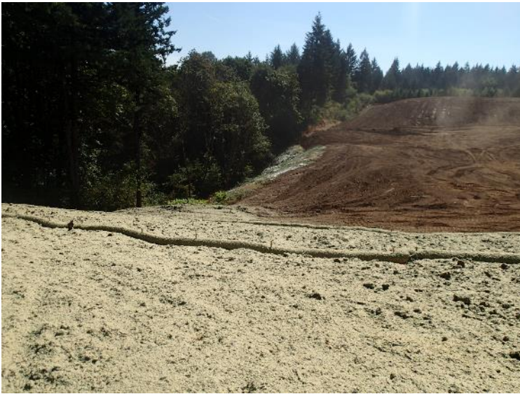
North buttress fill was hydroseeded and straw wattles placed according to erosion and sediment control plan (August 29, 2018).
