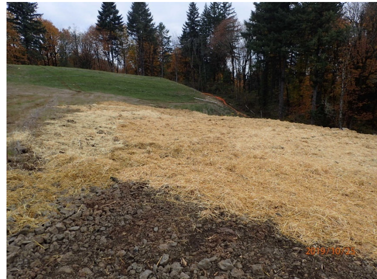
The construction area was stabilized and reseeded following installation of the rip-rap cover.
