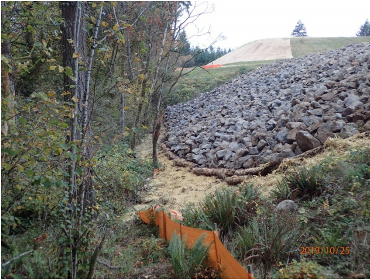
The toe of the rip-rap extended to the east margin of the landfill covering all remaining demarcation fabric.
