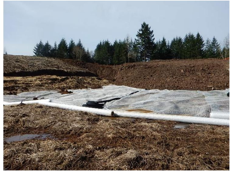
View west showing the buttress fill (left) and demarcation grid and cap (right). Note cap is substantially > 3 feet thick (March 29, 2018).
