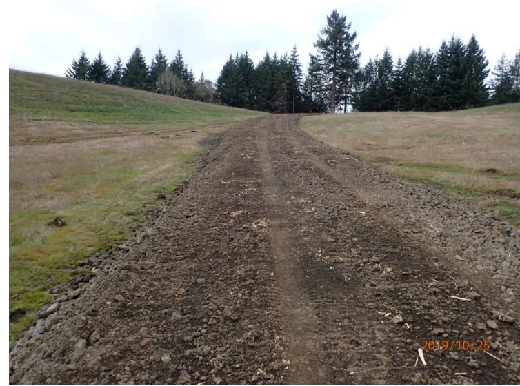
View of access road used to facilitate access for loading equipment while installing the rip-rap.
