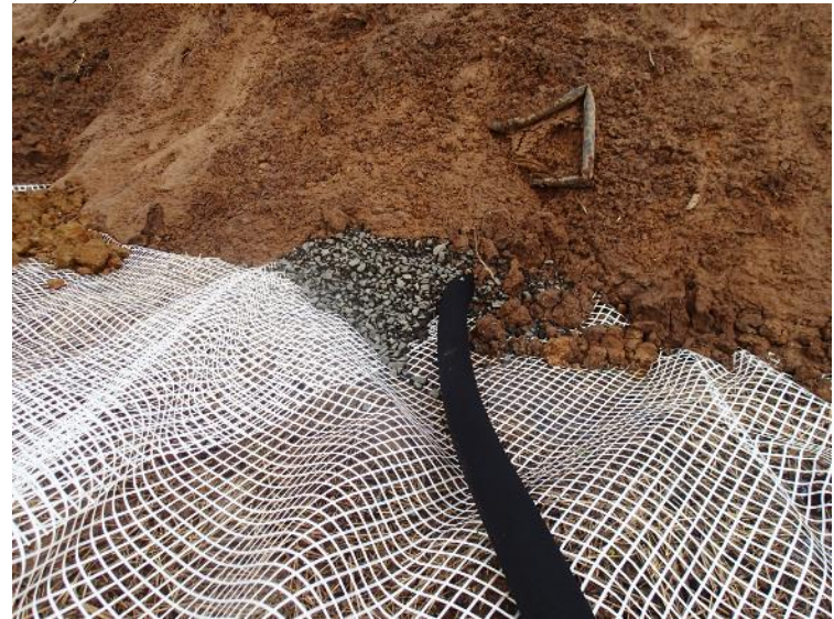
Drain pipe were bedded and covered with gravel prior to placing the soil cap (March 2, 2018).
