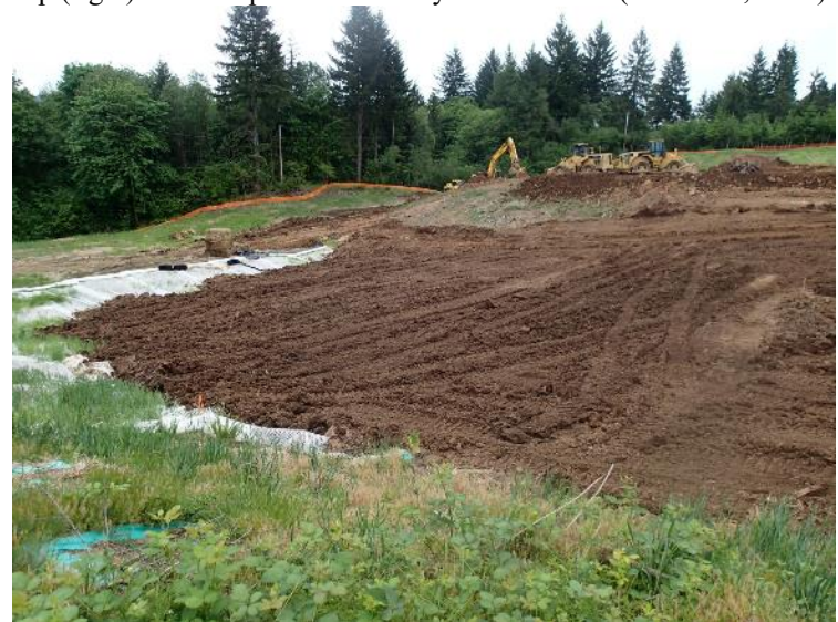
Landfill cap as it appears on May 17, 2018 – view southeast. Heavy equipment is sitting on the south buttress fill.
