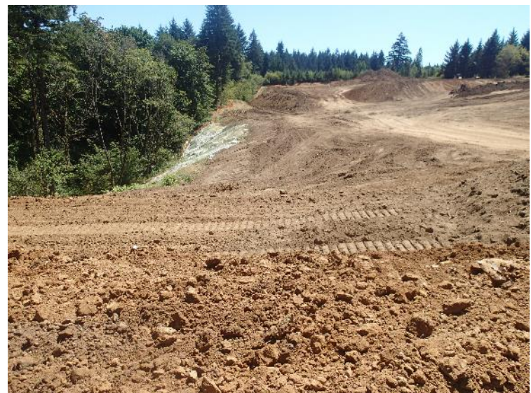
South buttress fill (under construction) from the perspective of the north buttress (July 24, 2018).
