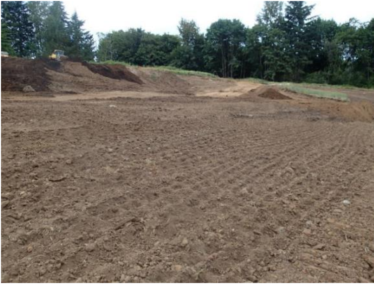
Cap surface was tracked and compacted with a sheepsfoot roller perpendicular to slope (June 25, 2018).
