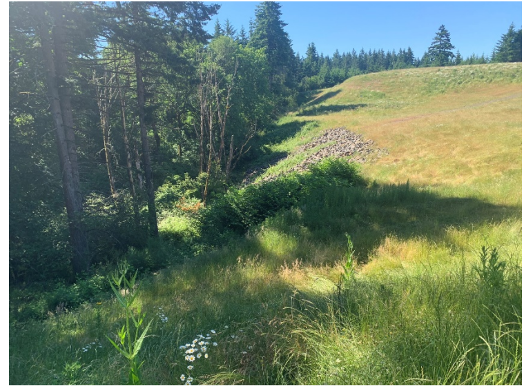
View south showing toe of the landfill. Due to steepness, the toe of the landfill is capped by riprap.
