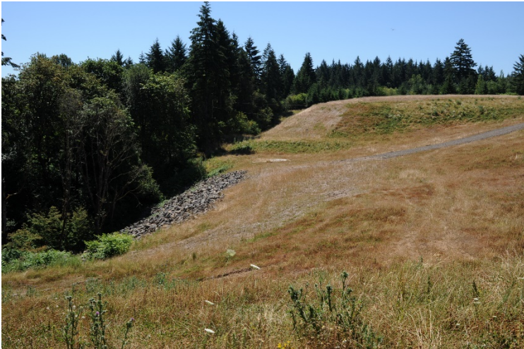
View south across landfill cap showing summer season grass cover to provide stability of slope conditions.
