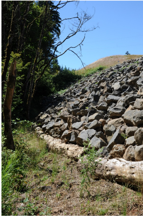
Closer view of landfill toe cap showing riprap with large logs at the toe.
