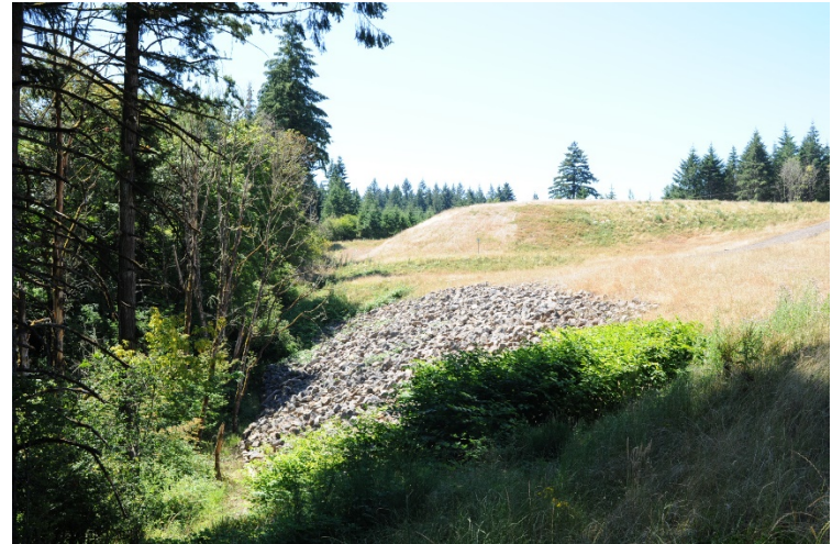
View south showing toe of the landfill. Due to steepness, the toe of the landfill is capped by riprap.
