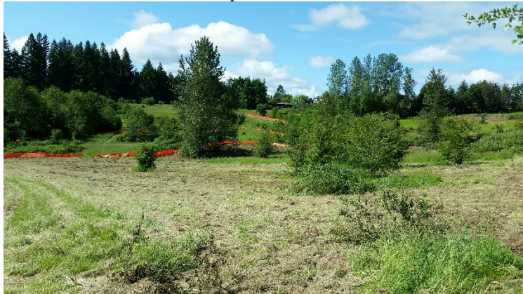
View looking south and east across DU03 and DU06 on June 2, 2017. Work to set up erosion control was beginning and areas had been mown and silt fencing was being erected.
