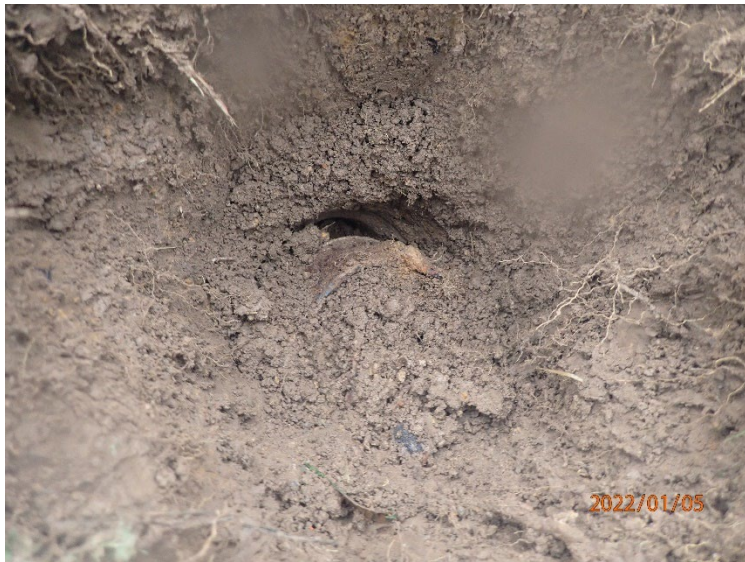
Hand excavation of MA01 revealed a broken 4-inch cast iron pipe possibly associated with a septic tank.
