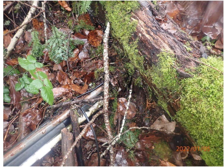
Vent line with other misc. conduits (MA03).
