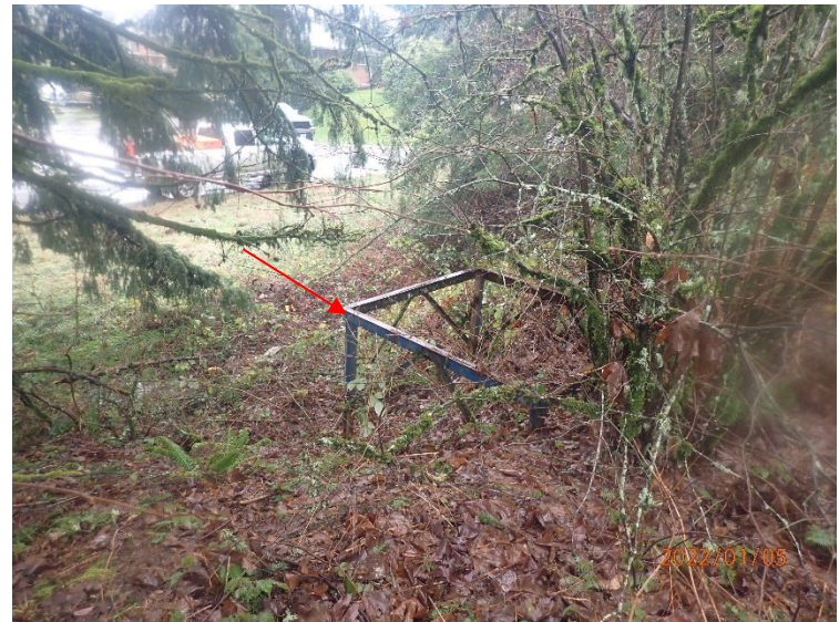
A rectangular metal structure believed to be a support for a former above-ground storage tank, where Comp01 was collected.
