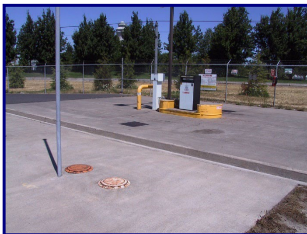
South Auto Gas Fueling Station
