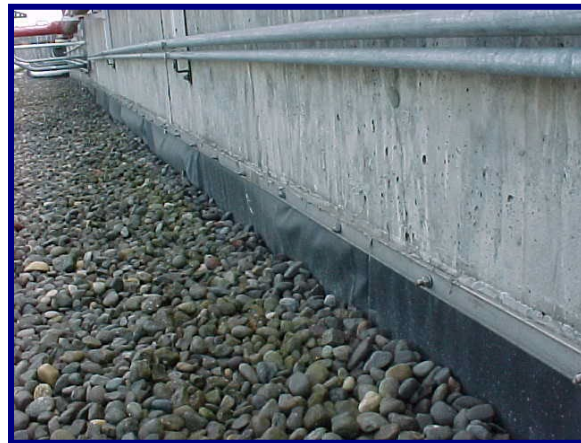
Secondary containment for ASTs.
