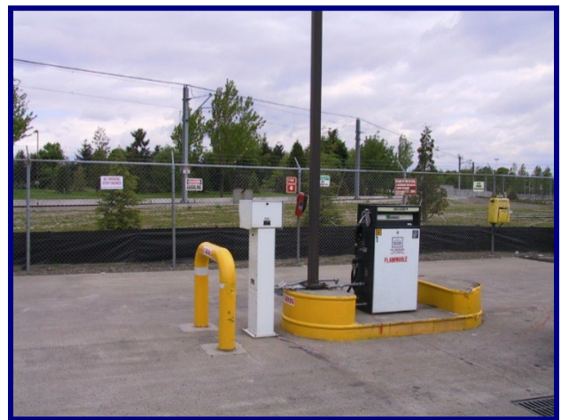
South GSE fueling station.
