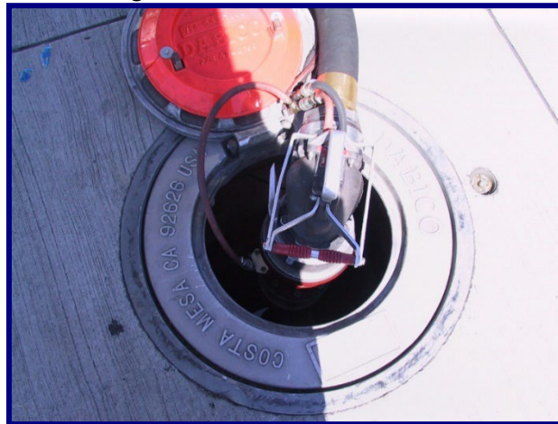
Hydrant pit (typical).
