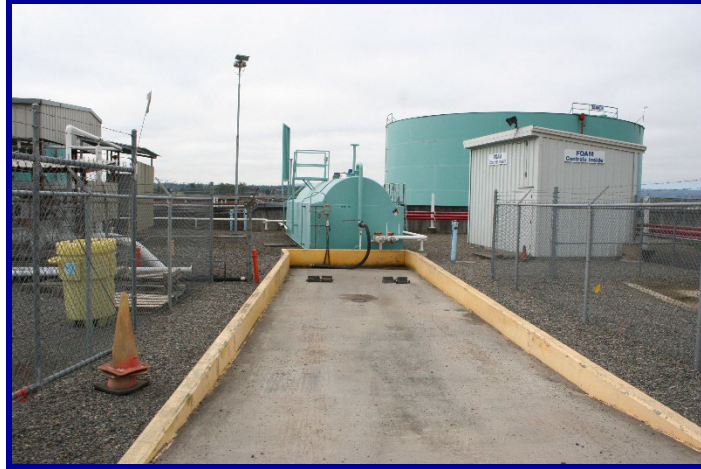
10,000-gallon Sump Fuel AST.
