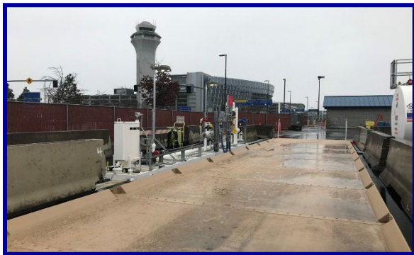
North GSE fueling station.
