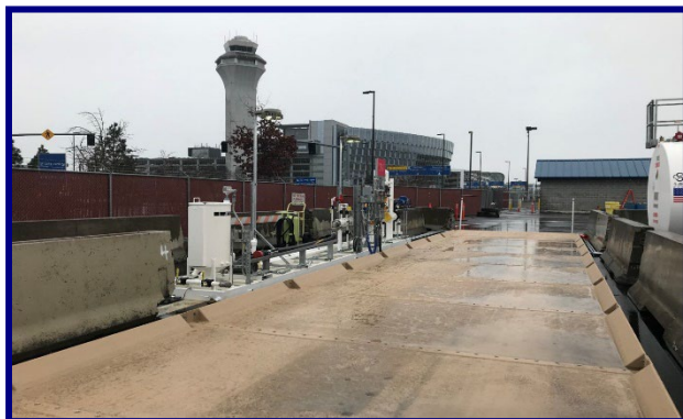
North Reload Rack.
