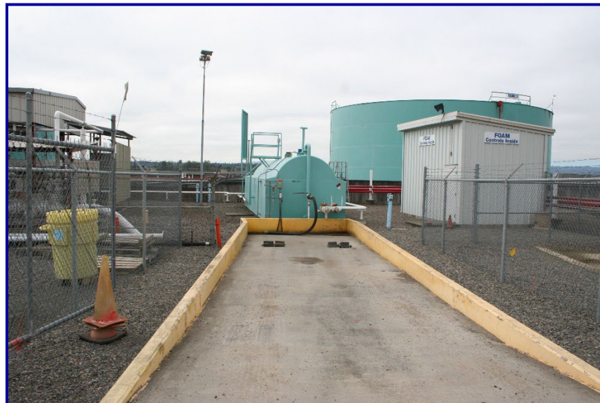
Sump fuel AST (USF).
