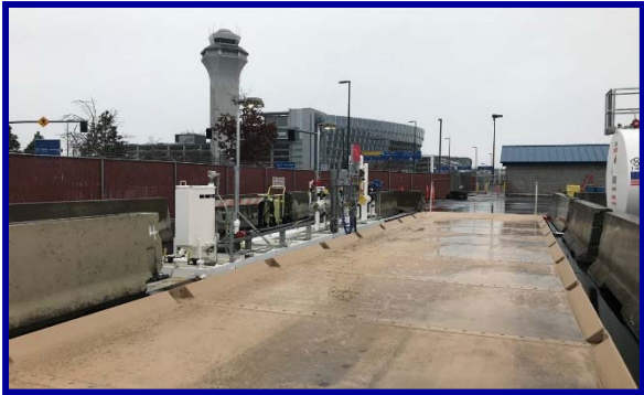
North GSE fueling station.
