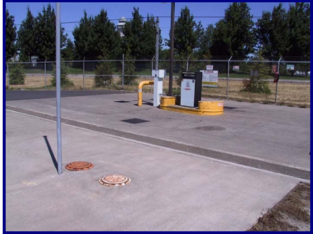
South Auto Gas Fueling Station
