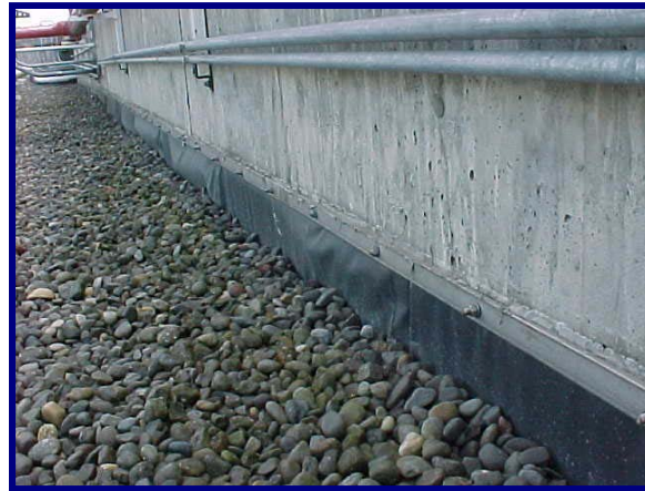
Secondary containment for ASTs.
