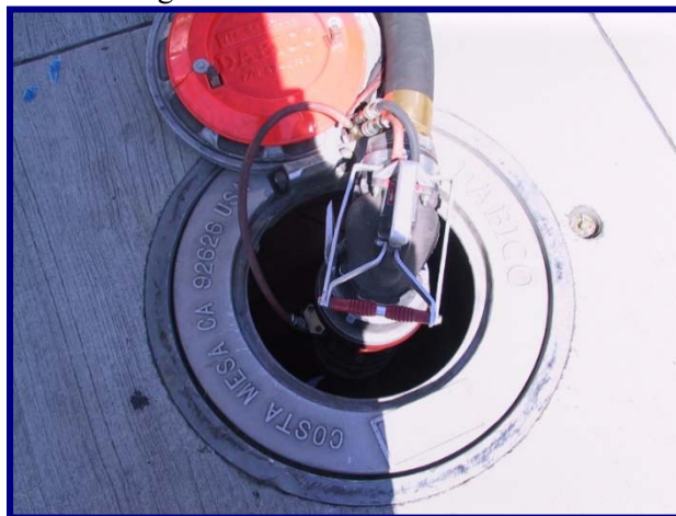
Hydrant pit (typical).
