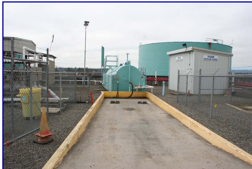
Sump fuel AST (USF).
