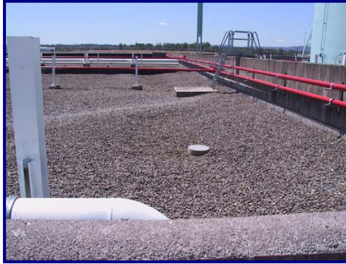
Secondary Containment for Tank #1 and #2 showing drain in foreground.
