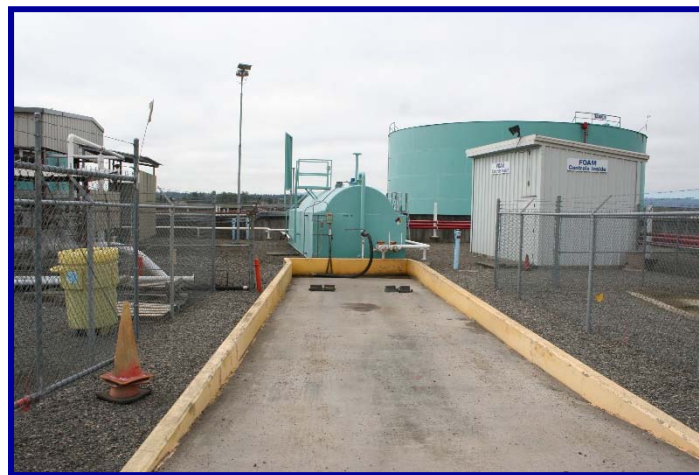
10,000-gallon Sump Fuel AST.
