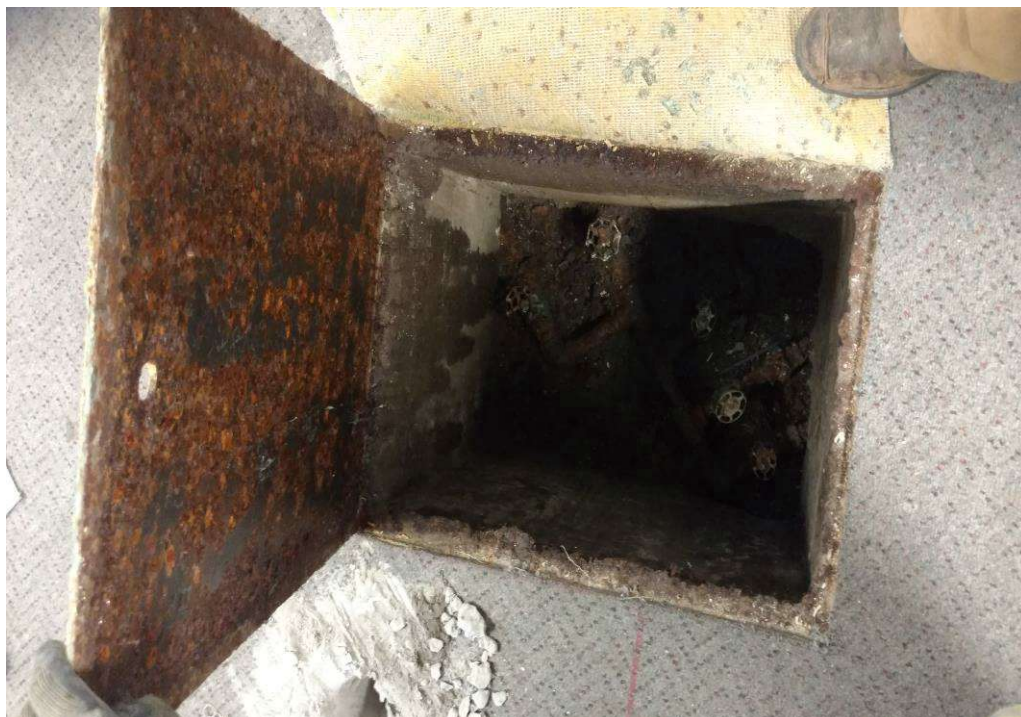
Photo 2 View of the suspect former waste pit / valve box located inside the Goodwill building.
