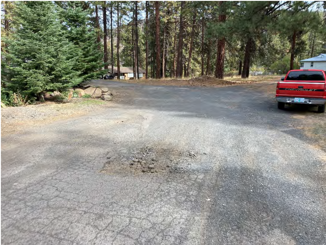
Potholes were evident further north toward the loop at the northern end of the road.
