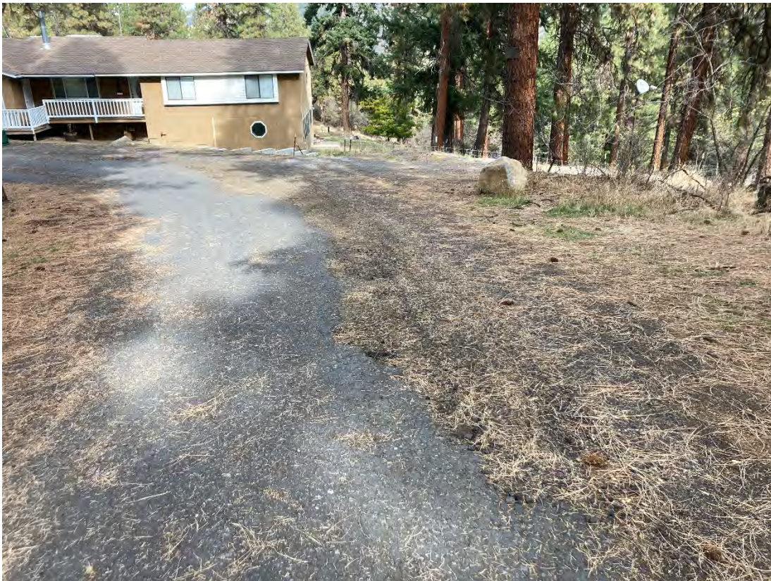
More of the worn pavement in the northern loop of Thicket Court.
