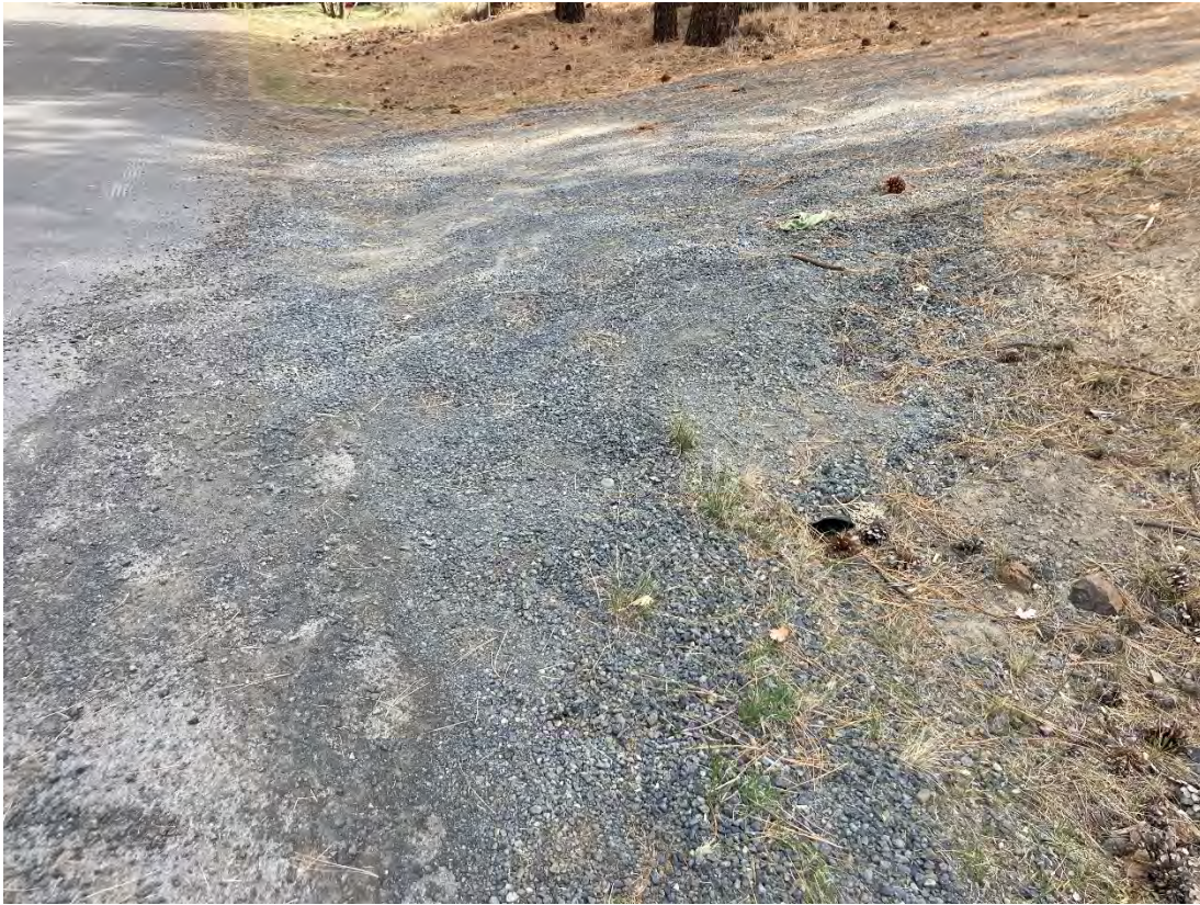
Several of the driveways on the southern end of Thicket Court have culverts that are obstructed.
