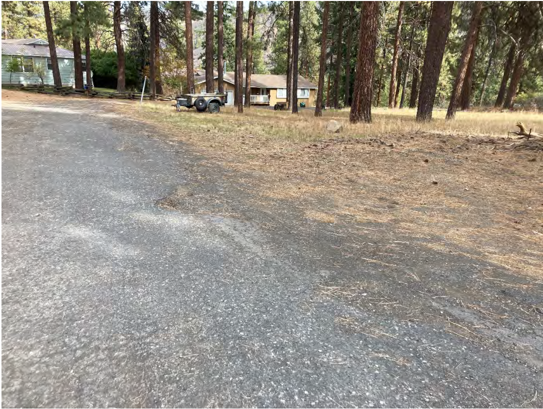
On the loop at the northern end, the pavement was worn away on the outside edge.
