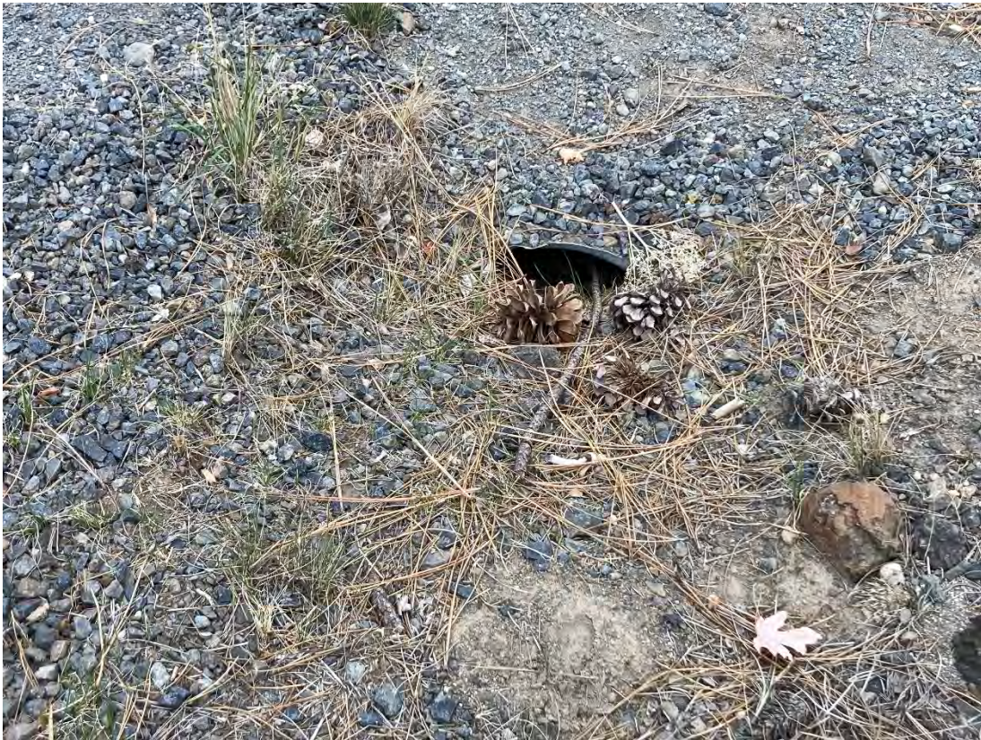
Majority of the culverts on the southern end of Thicket Court are obstructed by debris and soil.
