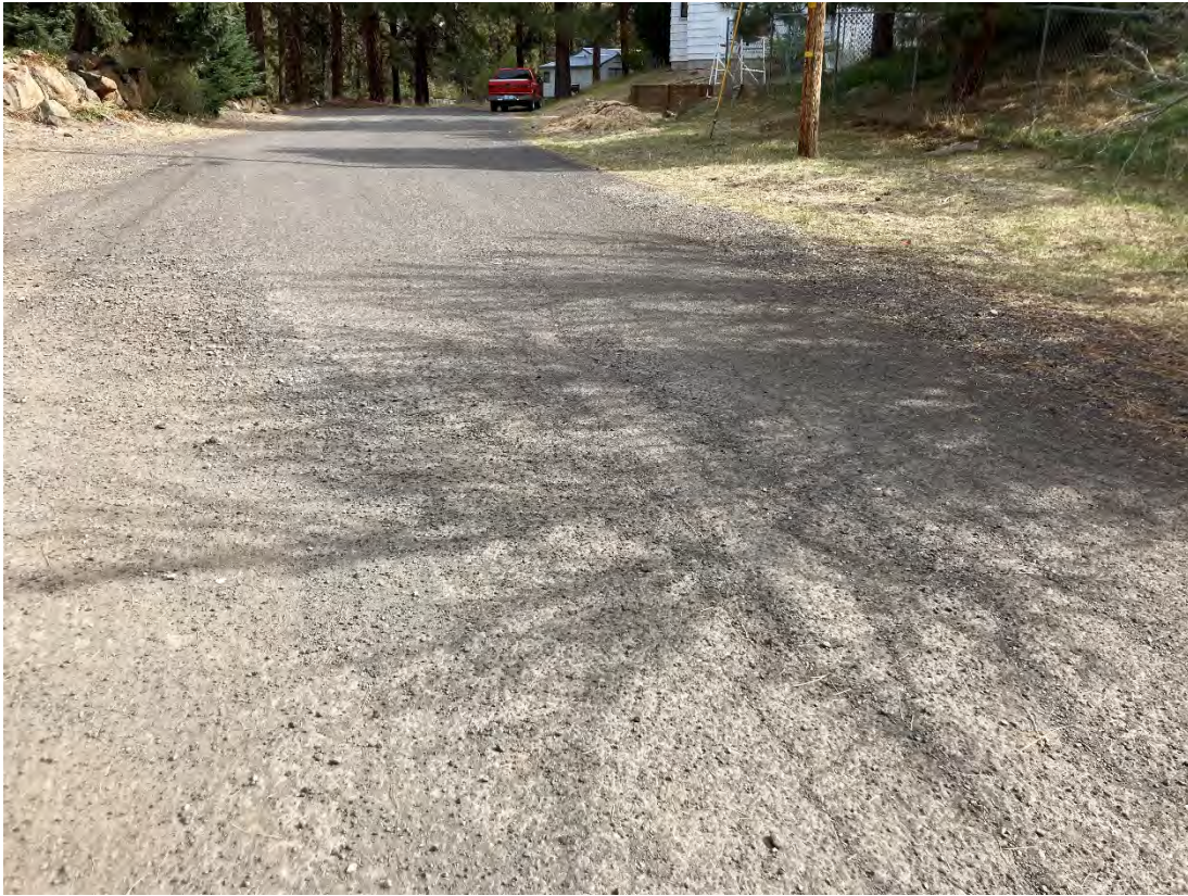
Several cracks were located on Thicket Court after proceeding north, away from Old Fort Road.
